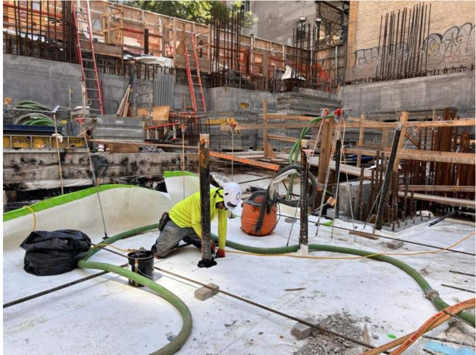
Photo 1: View of Urban installing waterproofing in the central part of the site (facing northeast).
