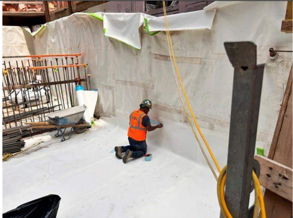
Photo 2: Urban installing the waterproofing /vapor barrier membrane in the northern part of the site (facing northwest).
