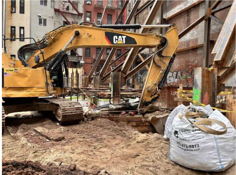
Photo 1: View of Urban excavating in the southern part of the site (facing east).
