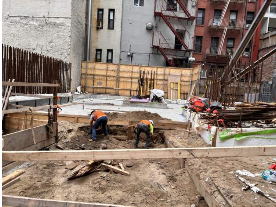
Photo 1: View of Urban excavating in the central part of the site (facing east).
