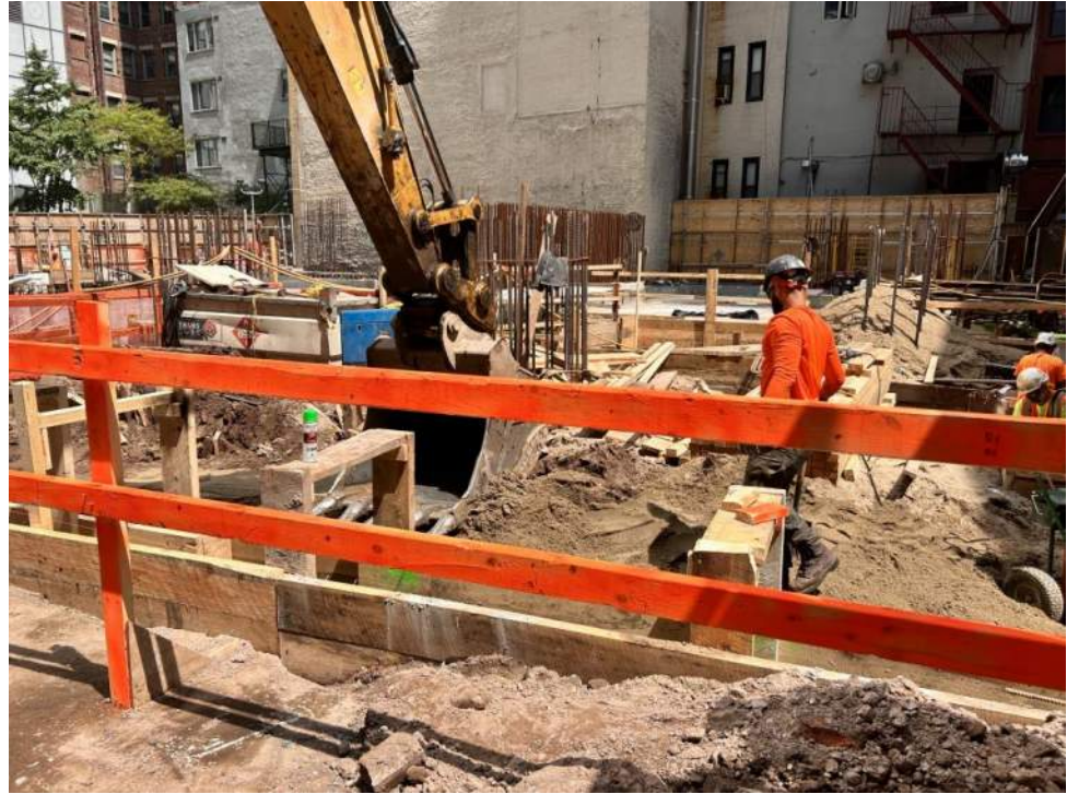
Photo 1: View of Urban grading in the southwestern part of the site (facing east).
