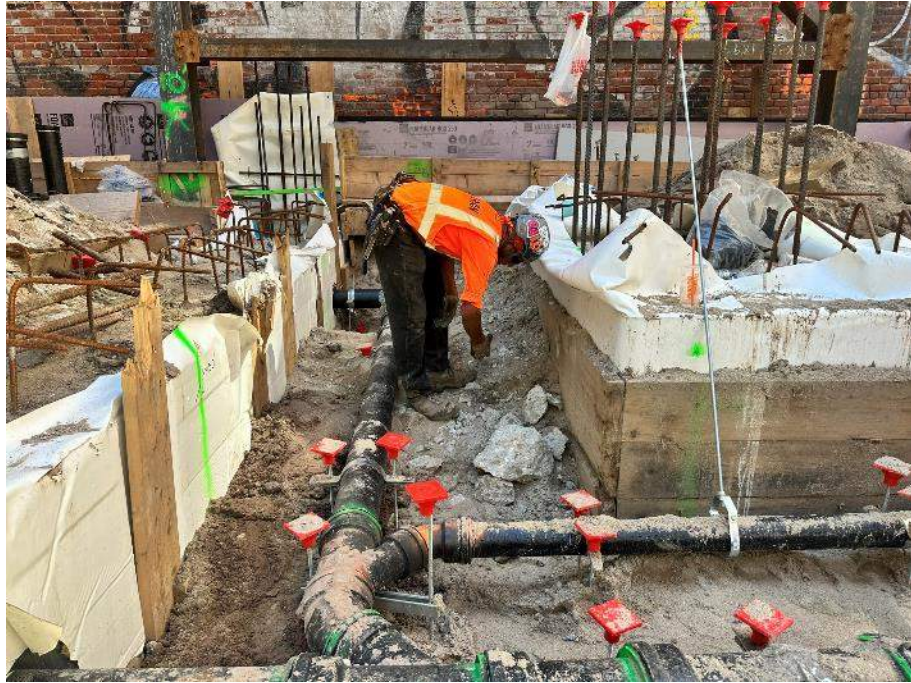
Photo 1: View of Urban excavating in the southern area of WC04 (facing south).
