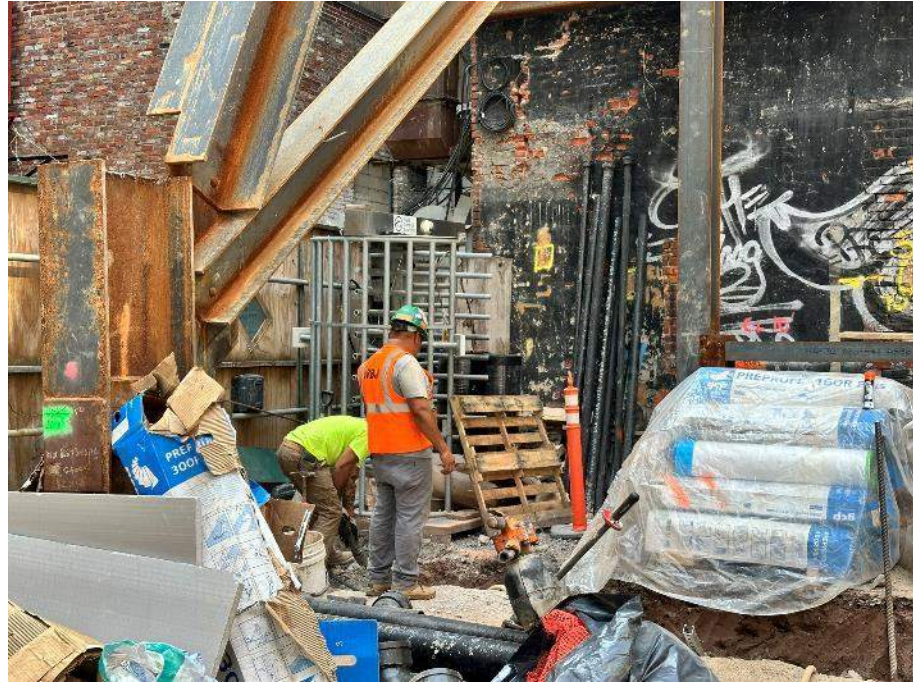
Photo 1: View of Urban removing concrete in the southeastern part of the site (facing southeast).
