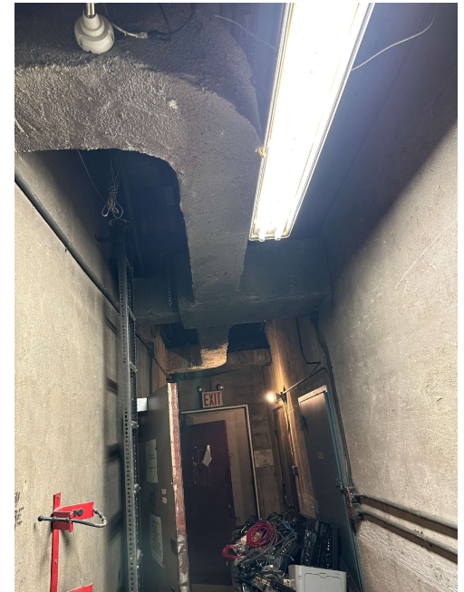
Ventilation ducts in basement
