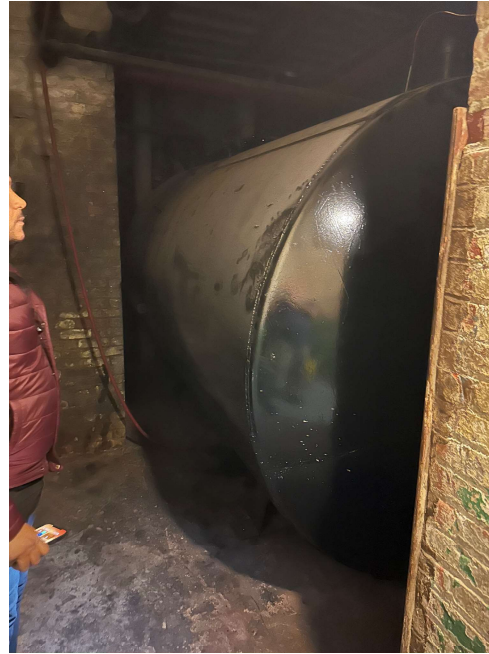
Fuel oil tank in basement
