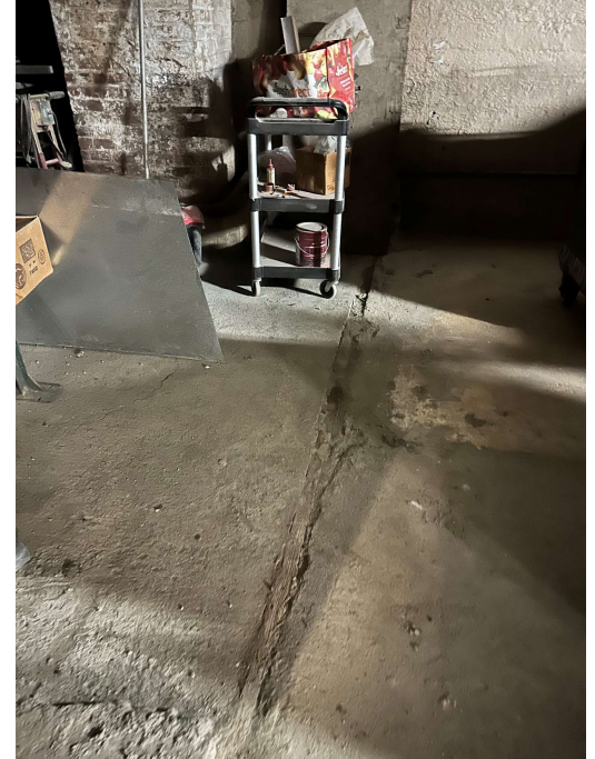
View of cracks in slab
