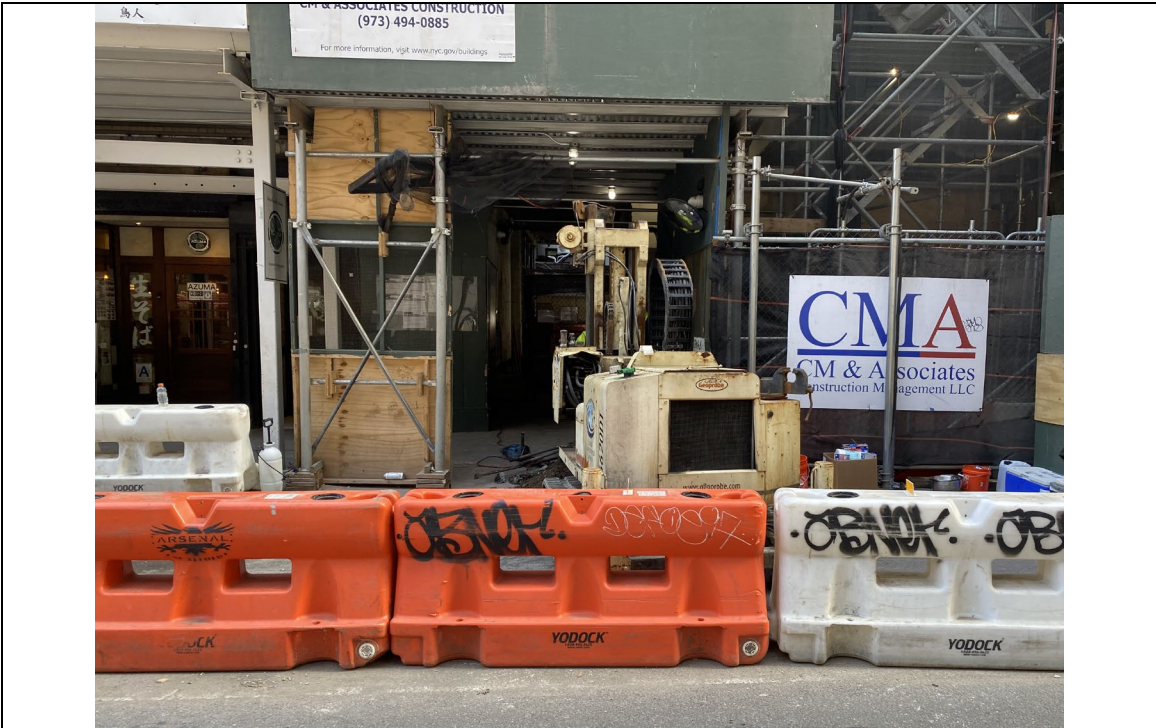
Photo 1: Drilling at SB-8/MW-8 location on the sidewalk off the southwestern corner of the building.
