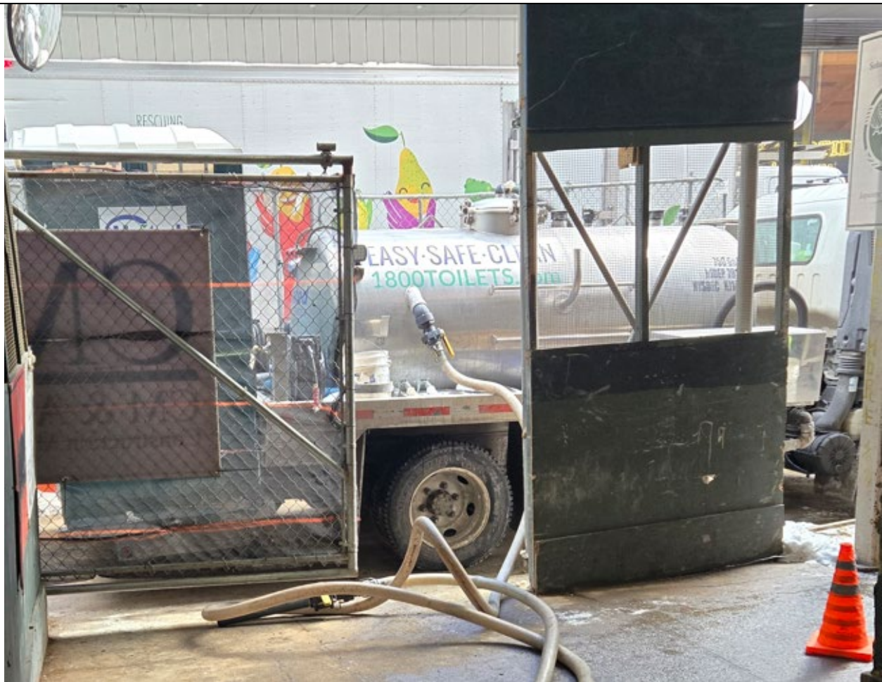
Photo 3: Running truck was likely the source of CAMP exceedance. Monitoring station (not pictured) is located immediately to the left of the gate.
