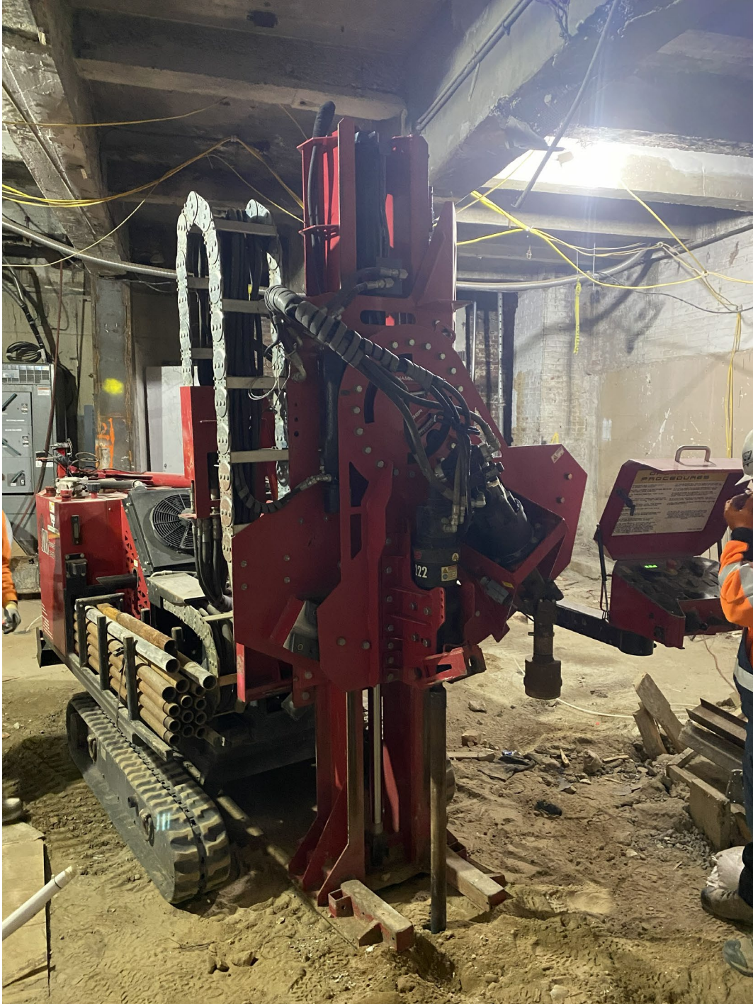
Photo 4: Refusal at 1.75' below basement grade for vapor probe point 15' northeast of SVE-3
