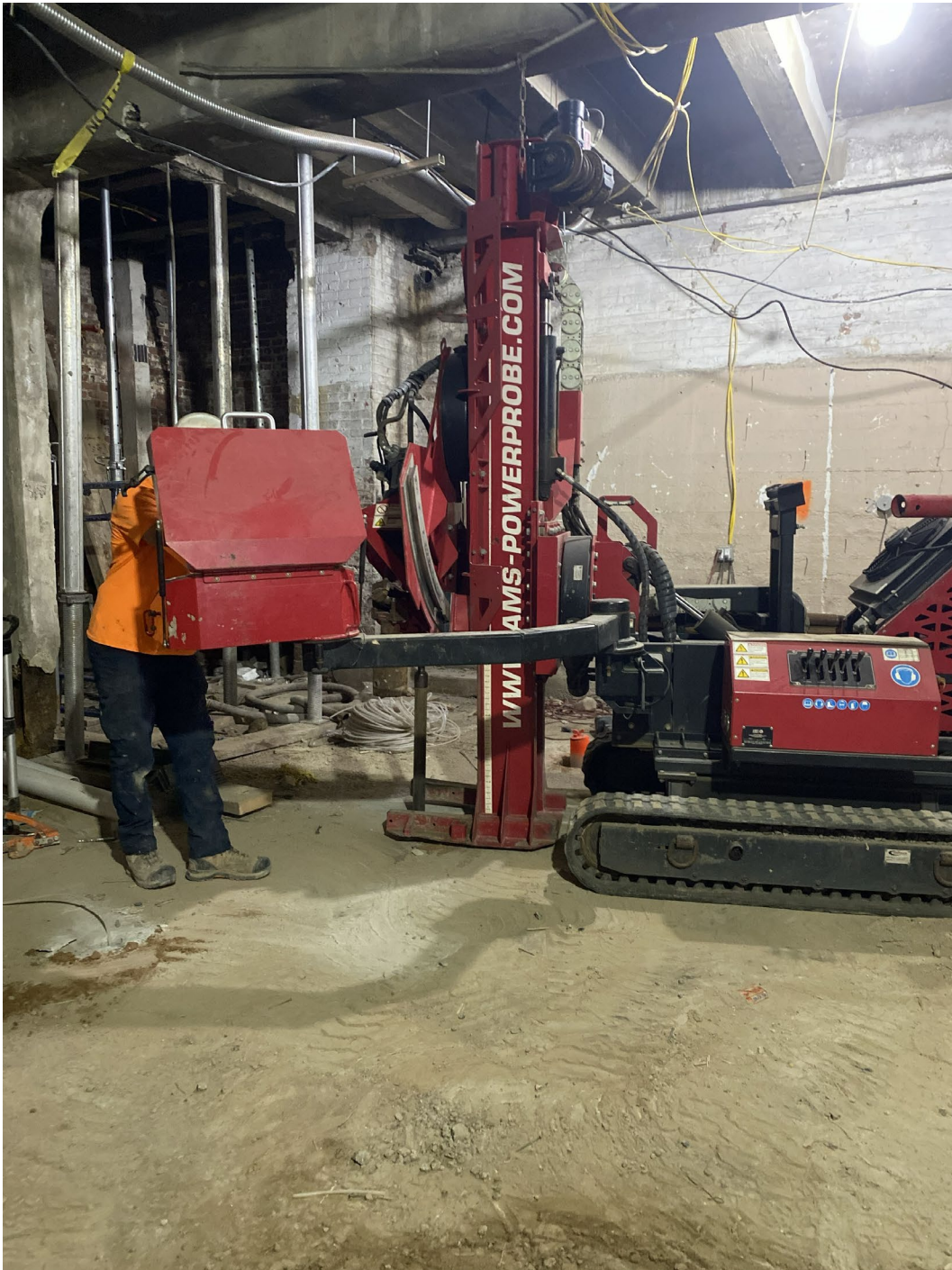
Photo 3: Refusal at 3.25' below basement grade for vapor probe point 5' east of SVE-3
