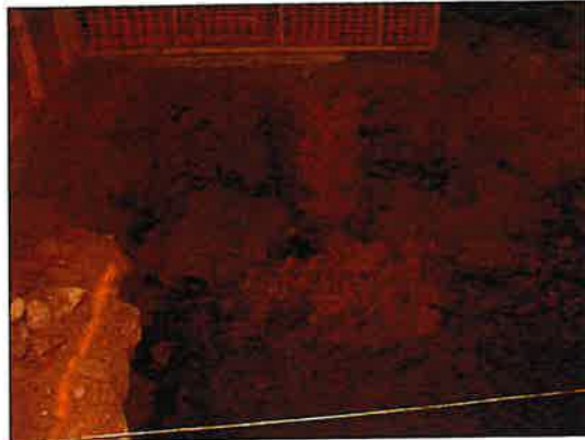
4. View into bottom of excavation with undermined column located to the left.
