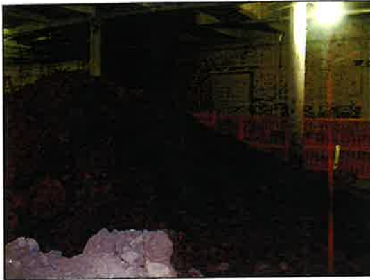
1. Stockpiled petroleum contaminated soil adjacent to the excavation.
