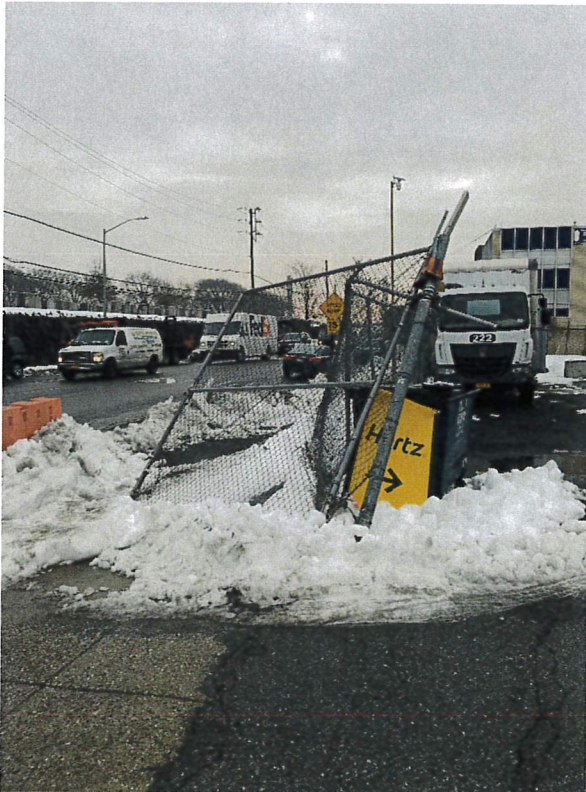
Photo 4. Damaged Gate Main Entrance RAD II
