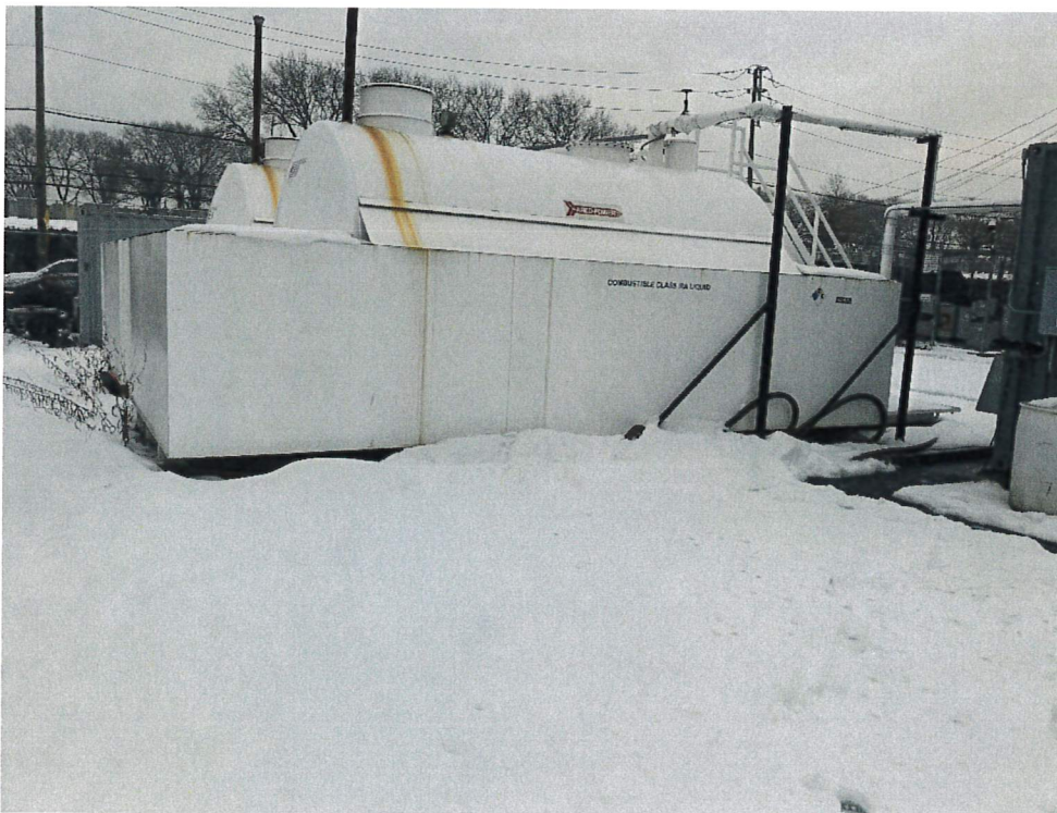
Photo 2. Waste Oil Storage Tanks
