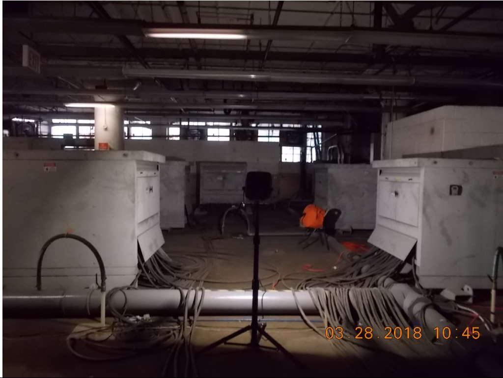
Photo # 9: Electrode Field/Electrical Transformers
