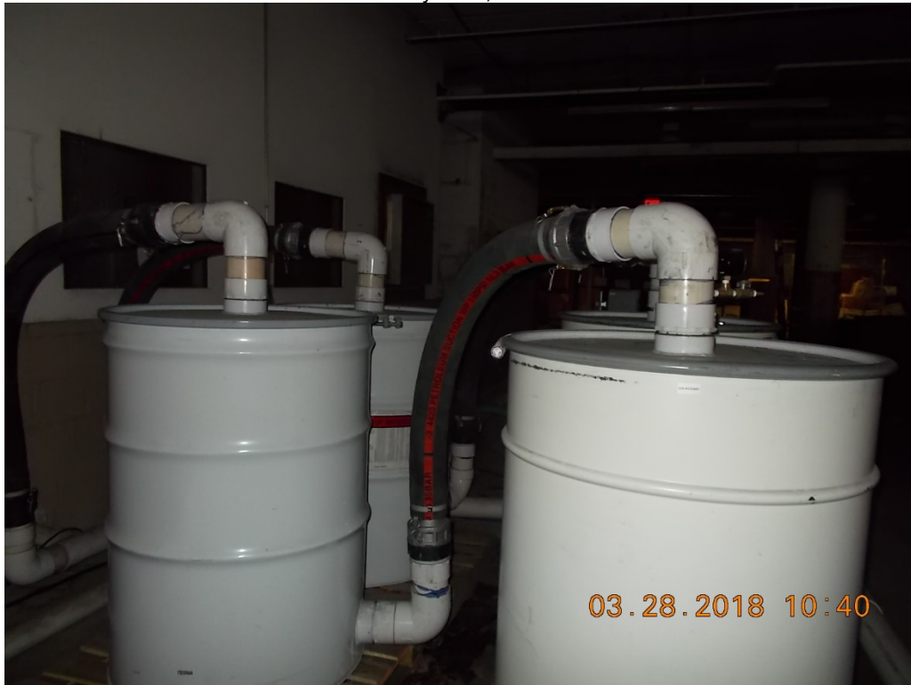
Photo # 6: SVE System, Carbon Canisters
