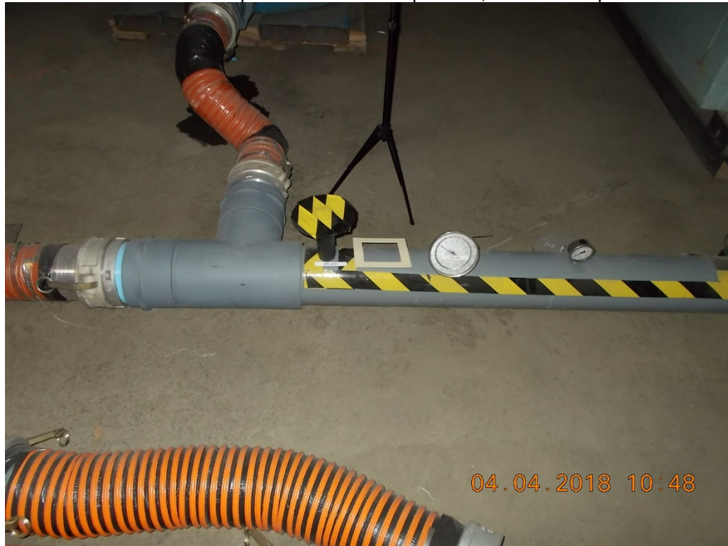
Photo # 20: Surface Sample Location #3 – Vapor Line, Influent Sample Port Area
