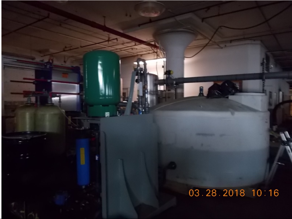
Photo # 5: Condensate Tank
