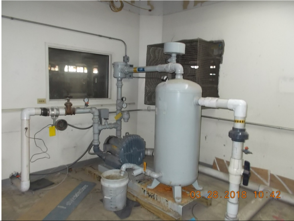
Photo # 7: SVE System, Knock-out Tank
