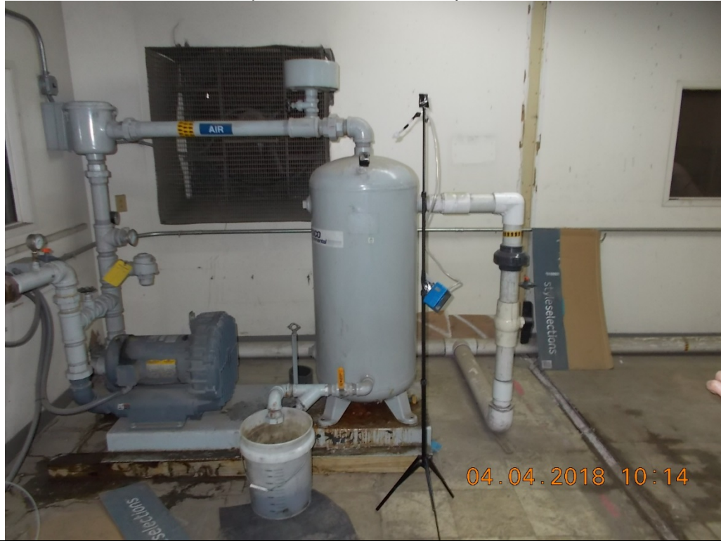
Photo # 15: Air Sample Location #3 – SVE System, Knock-out Tank
