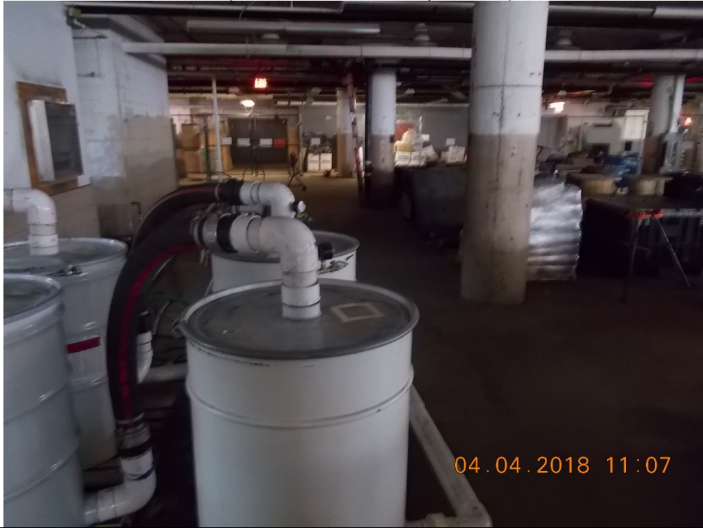
Photo # 23: Surface Sample Location #6 – SVE System, Top of Carbon Canisters
