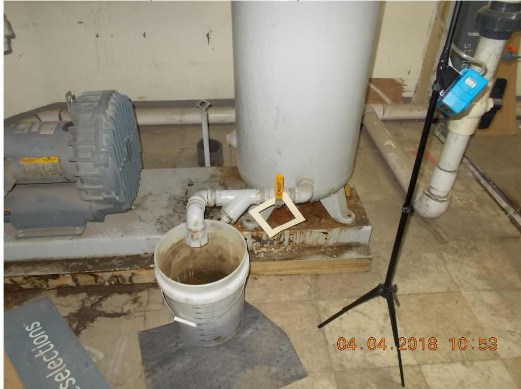
Photo # 21: Surface Sample Location #4 – SVE System, Knock-out Tank (Blower Room)
