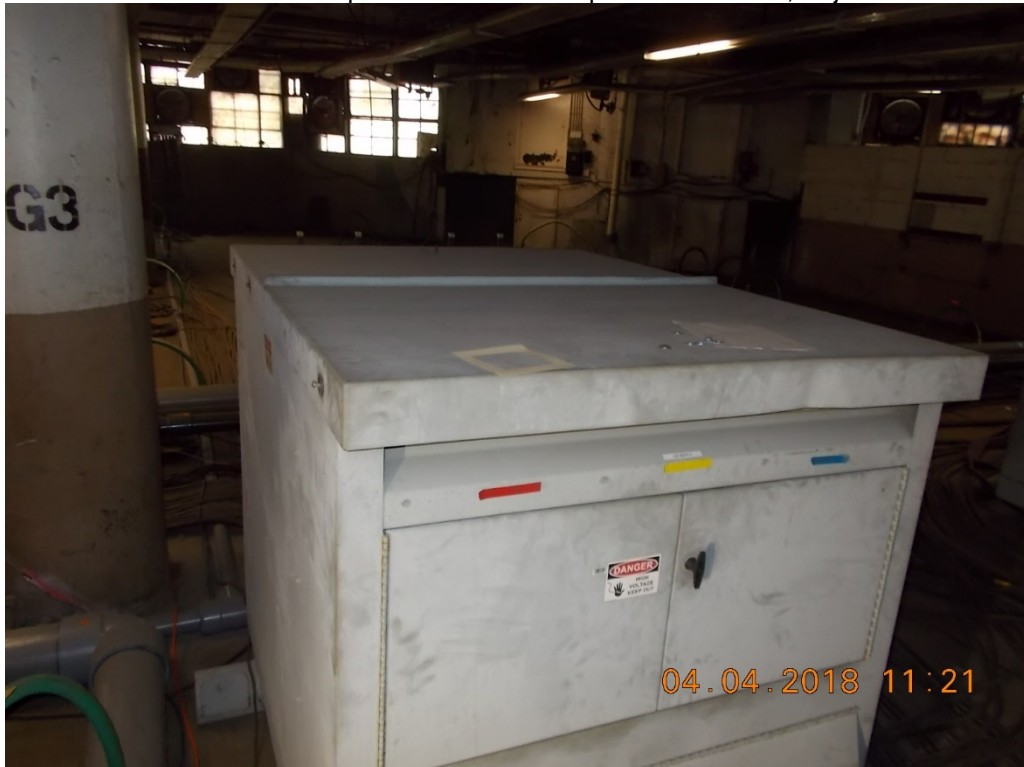
Photo # 26: Surface Sample Location #9 – Top of Transformer, Adjacent to G03
