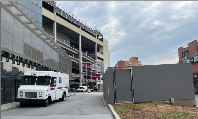
Photograph 7: The concrete slab driveway at the SVP West Entrance Pavilion (Parcel 2).
