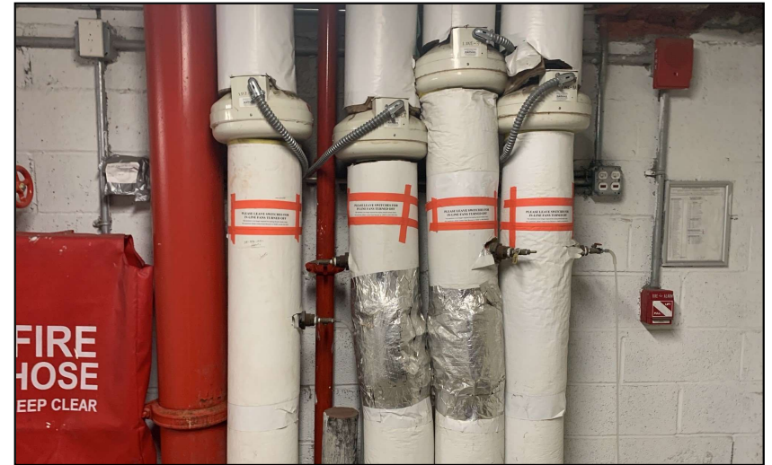
Photograph 4: The SSDS fans and riser piping in the 1 st floor southern stairwell of the retail building on the western portion of the Property (Parcel 2).
