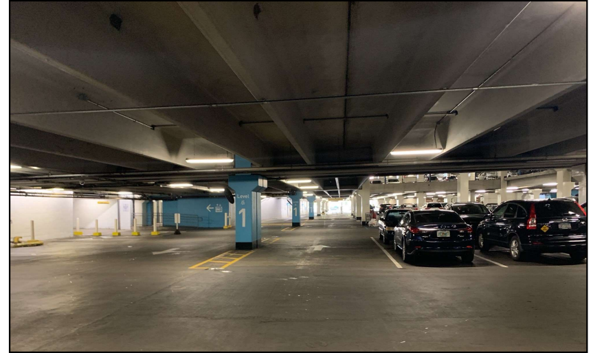
Photograph 2: The concrete slab in the underground parking garage on the western portion of the Property (Parcel 2).
