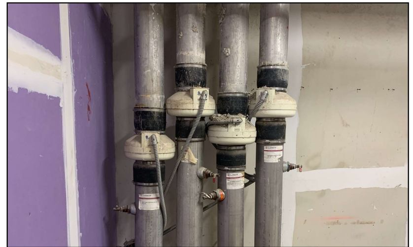
Photograph 8: The SSDS fans and riser piping in the 1 st floor Northern stairwell of the retail building on the western portion of the Property (Parcel 2).
