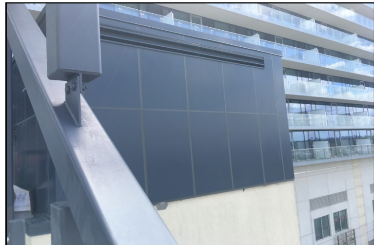
Photograph 12: Newly constructed SSDS pipe enclosure equipped with louvers atop the western retail podium (Parcel 2).
