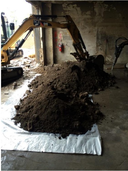
9. Looking north inside Paint Factory Building. Photo taken on Wednesday, September 30, 2015. Excavating soil for Test Pit 5 and stockpiling on poly.
