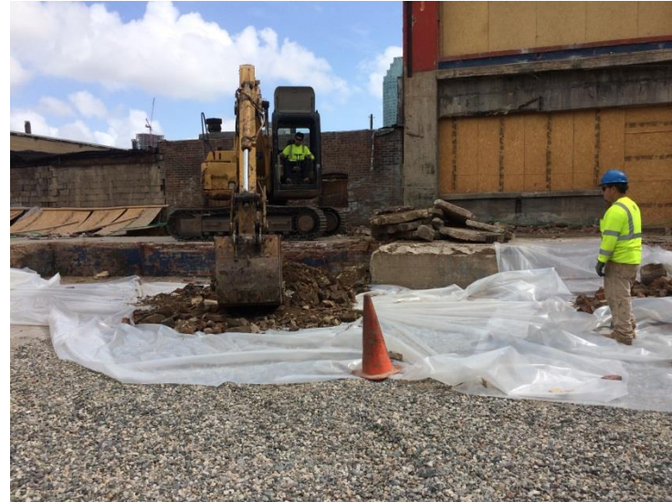
2. Looking northeast in courtyard. Photo taken on Tuesday, September 29, 2015. Backfilling Test Pit 1 with material that was excavated from test pit.
