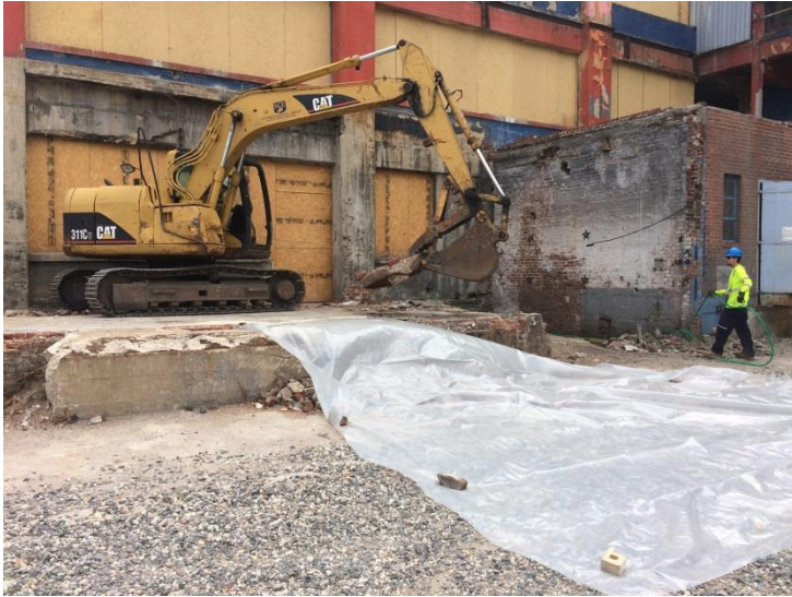
1. Looking southeast in courtyard. Photo taken on Tuesday, September 29, 2015. Removing concrete before beginning excavation for Test Pit 1.
