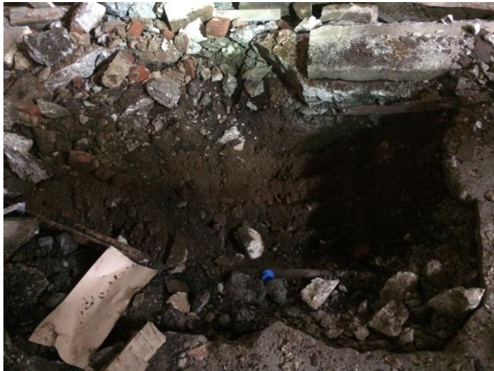
11. Photo taken on Thursday, October 01, 2015. Test Pit 6 excavated to final depth of approximately 5 ft bls.
