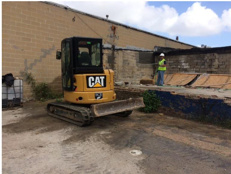
5. Looking northeast in courtyard. Photo taken on Tuesday, September 29, 2015. Breaking apart concrete at location for Test Pit 3.
