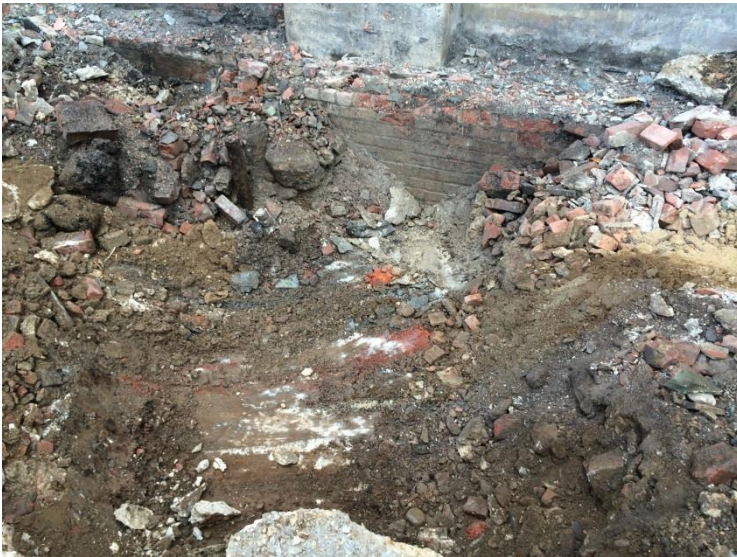
3. Looking east in courtyard. Photo taken on Tuesday, September 29, 2015. Excavating soil from Test Pit 2.
