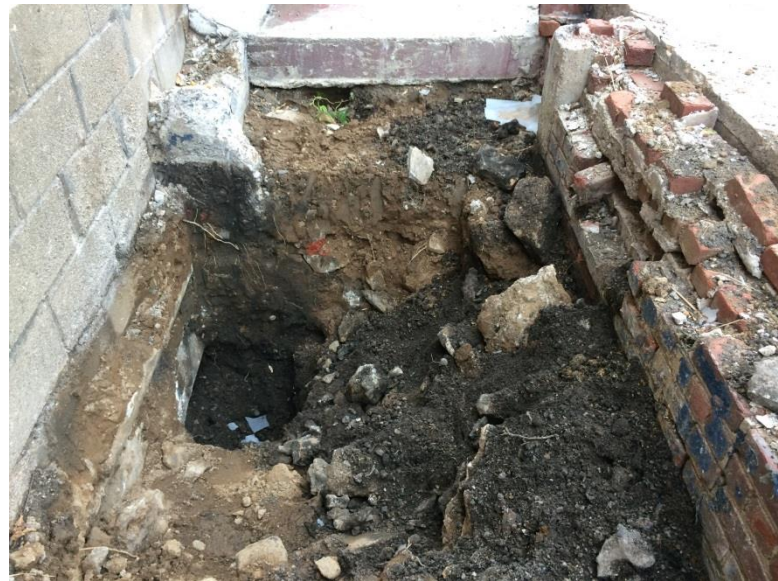
6. Looking east in courtyard. Photo taken on Tuesday, September 29, 2015. Excavating soil in Test Pit 3 to final depth of approximately 5 ft bls.
