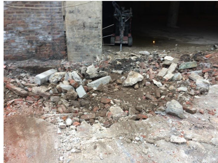
4. Looking east in courtyard. Photo taken on Tuesday, September 29, 2015. Test Pit 2 backfilled to previous grade at the end of day with material that was excavated from test pit.
