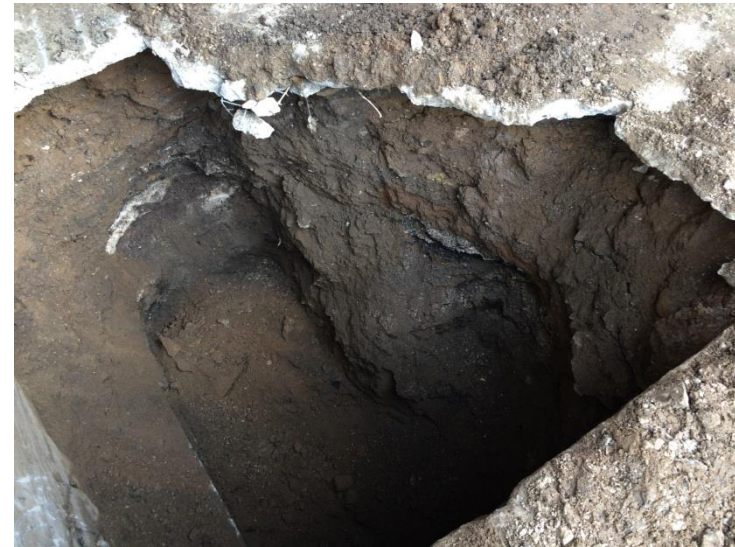
10. Photo taken on Wednesday, September 30, 2015. Test Pit 5 excavated to final depth of approximately 5 ft bls.
