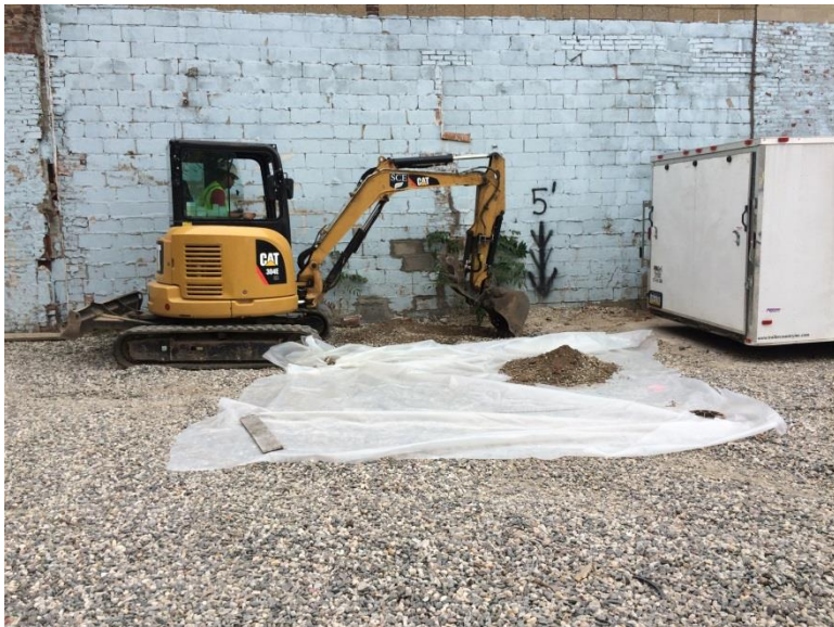
7. Looking west in courtyard. Photo taken on Tuesday, September 29, 2015. Beginning to excavate for Test Pit 4, stockpiling soil onto poly.
