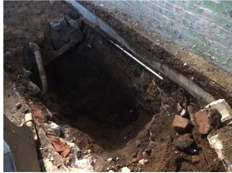
14. Photo taken on Thursday, October 01, 2015. Excavated to final depth of approximately 5 ft bls at Test Pit 7.
