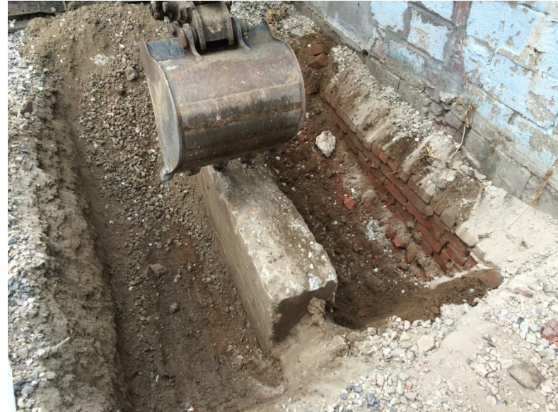
8. Looking southwest in courtyard. Photo taken on Tuesday, September 29, 2015. Excavating soil in Test Pit 4 to final depth of approximately 5 ft bls.
