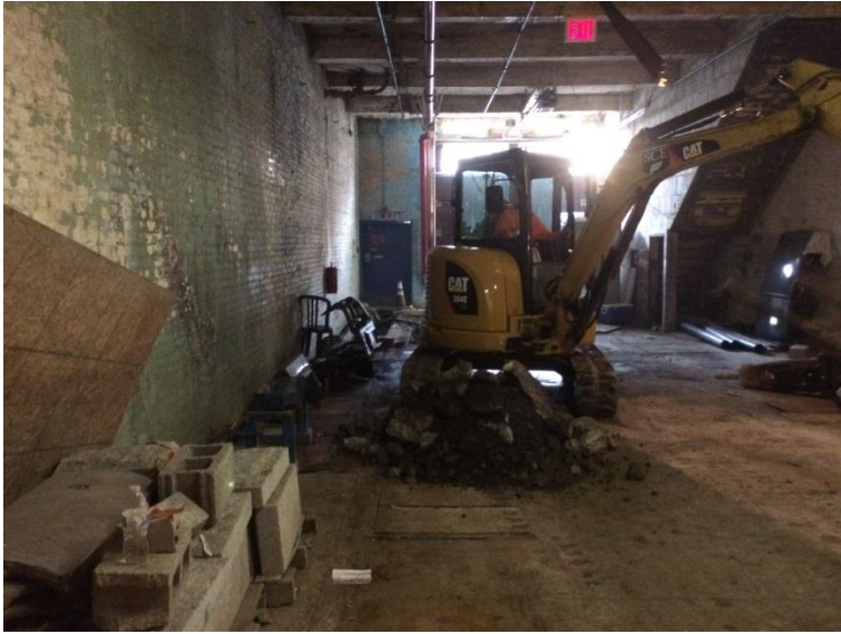
13. Looking south inside Garage Photo taken on Thursday, October 01, 2015. Excavating at location for Test Pit 7.
