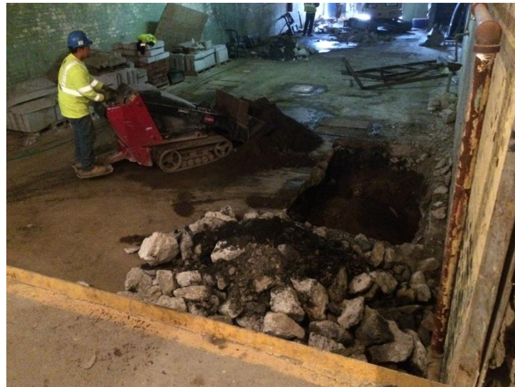
12. Looking southwest inside Garage Building Photo taken on Thursday, October 01, 2015. Backfilling Test Pit 6 with soil excavated from test pit.
