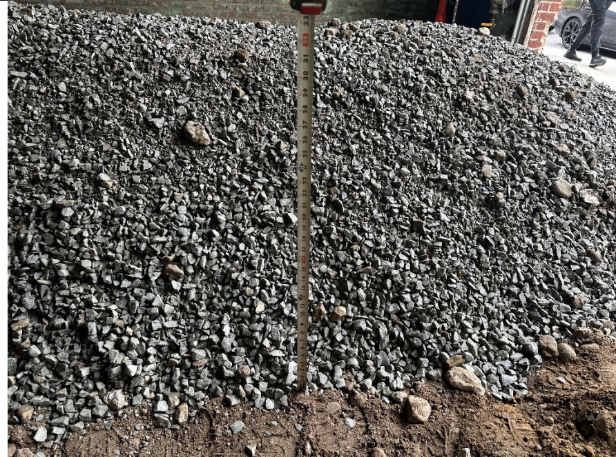
Photo 3: Facing east, measurement of minimum 2 feet of NYSDEC-approved backfill material covering area of disturbance.
