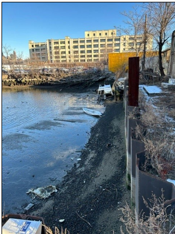
Photograph 8: View of Anable Basin and condition of bulkhead looking north
