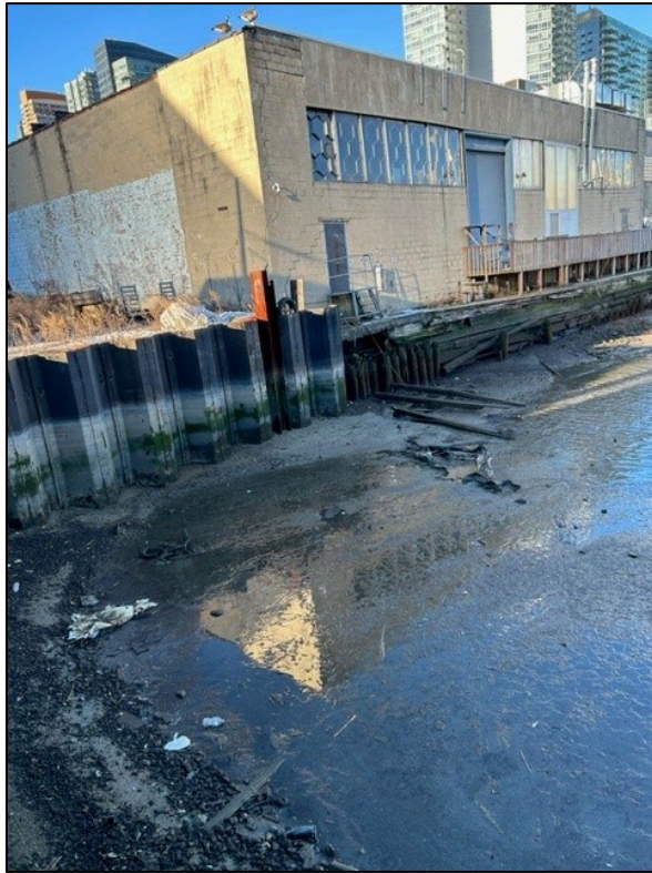
Photograph 7: View of Anable Basin and condition of bulkhead looking west
