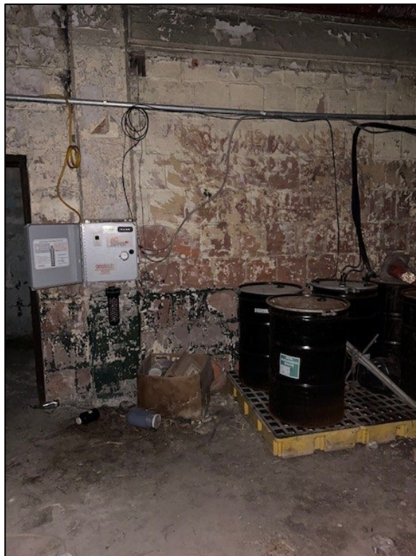
Photograph 10: Geotech AC Sipper control panel
