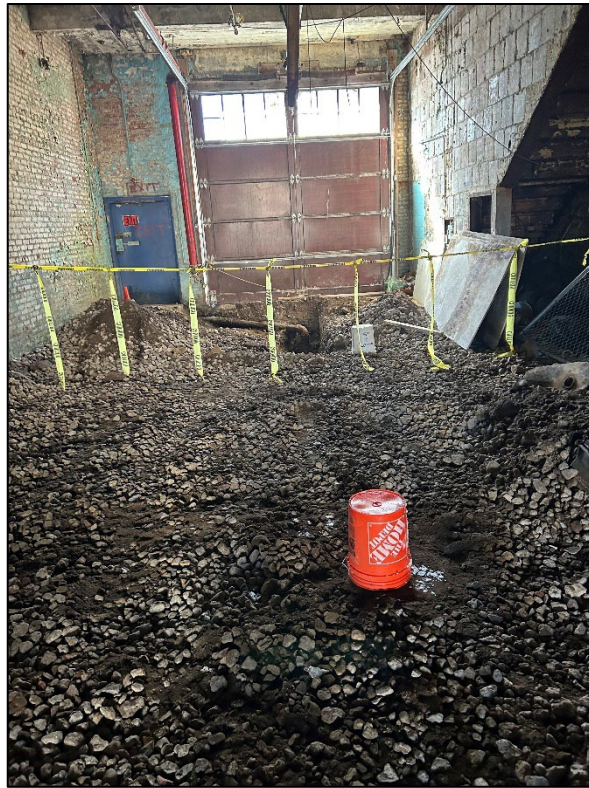
Photograph 13: RCA cap disturbance observed in garage
