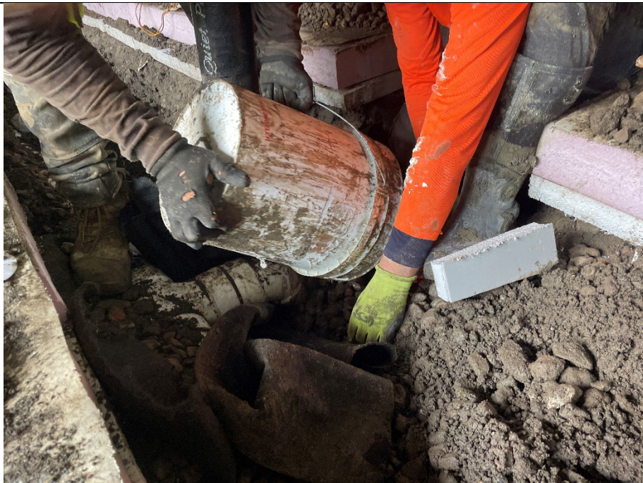
Photo 2: Facing southeast, view of NY Axon filling space around SSDS PVC piping with RCA.
