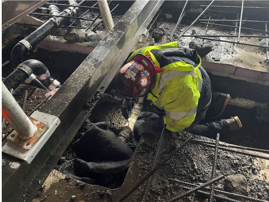
Photo 1: Facing north, NY Axon drills drainage holes in SSDS piping on the utility crossing areas.
