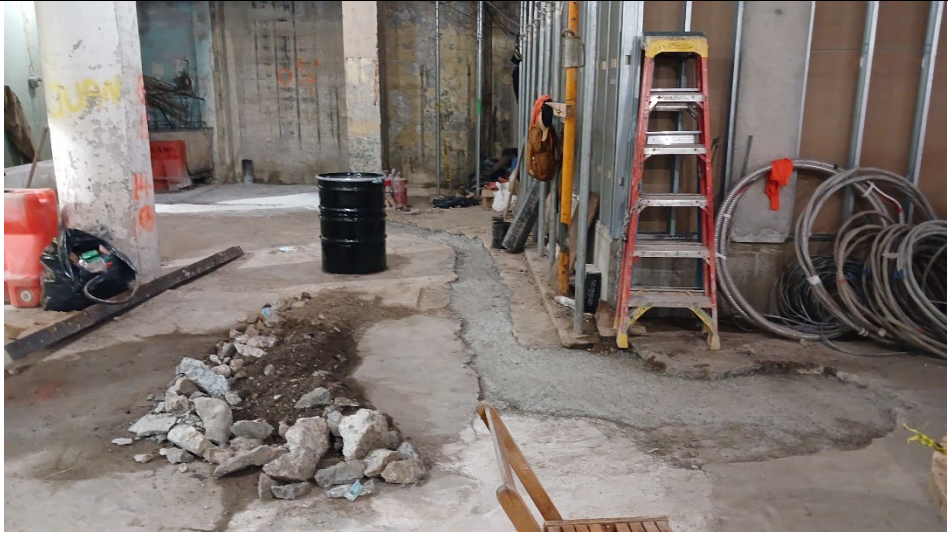
Photo 1: Facing south-southwest, view of conditions within the trench work area after recent concrete pouring.
