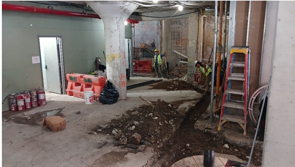
Photo 3: Facing southeast, view of Li Xiang Plumbing grading soil within the utility trench.
