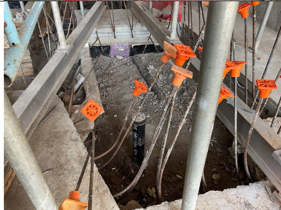
Photo 2: Facing northeast, view of an exposed pit requiring further vapor barrier installation.
