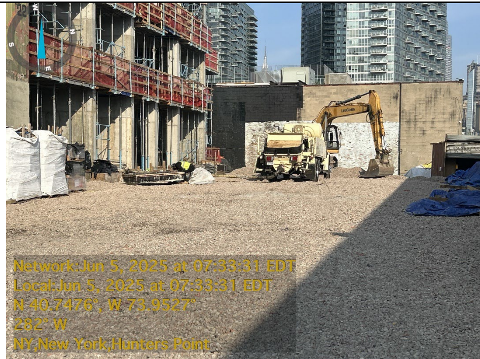
Photo 1: Facing west, view of setting up concrete pump truck in the northern region of the Site.
