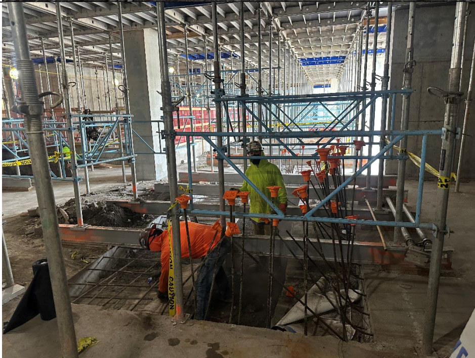
Photo 2: Facing west, view of NYC Axon clearing the open slab on grade sections to reinstall vapor barrier components.
