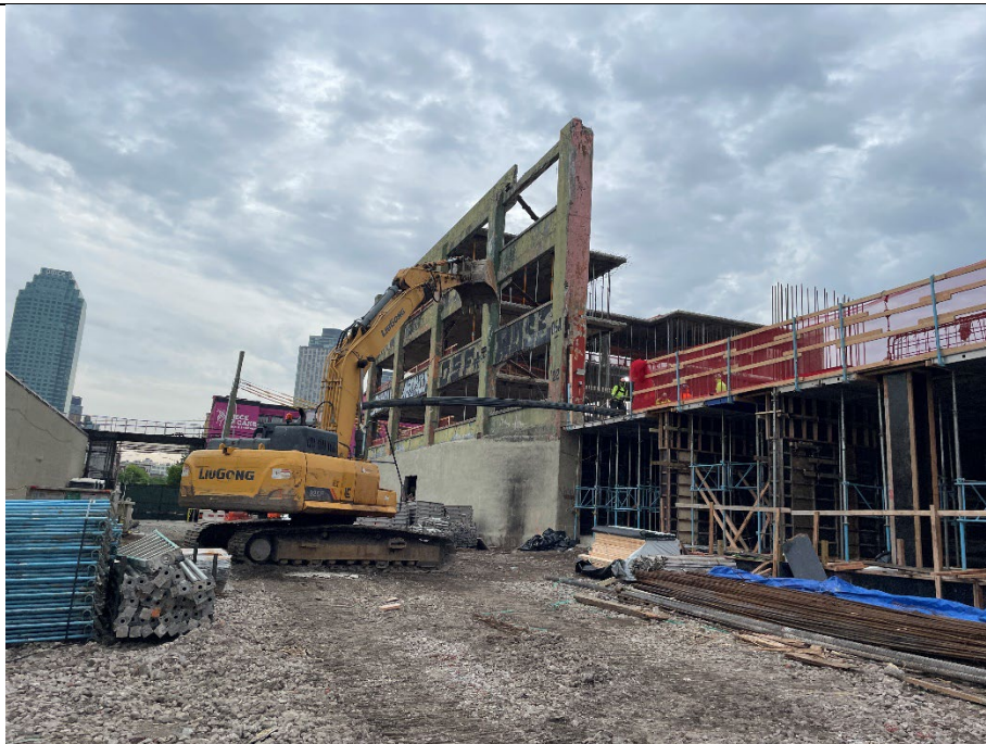
Photo 2: Facing southeast, NY Axon transporting rebar to the second floor after a recent delivery.
