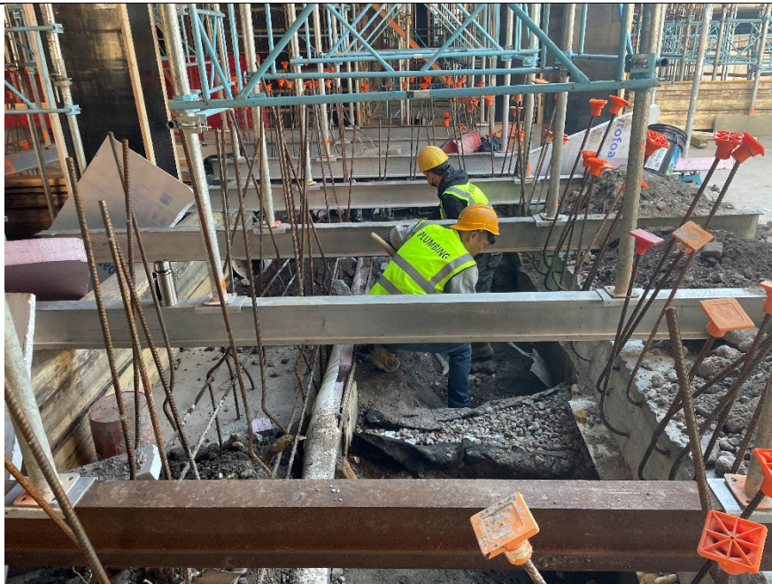
Photo 2: Facing southwest, view of LX plumbers clearing soil for installation of underground utilities.
