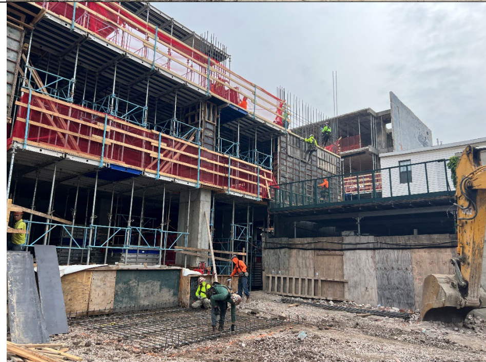
Photo 2: Facing northeast, view of NYC Axon installing concrete formwork and stripping formwork on the second level.
