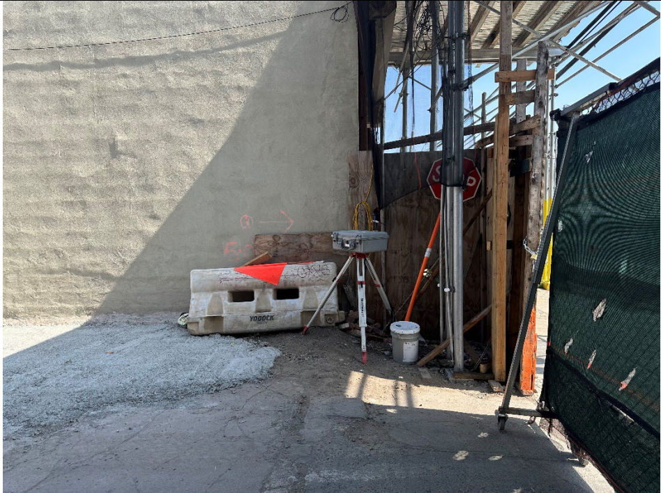
Photo 1: Facing north, view of upwind CAMP station.
