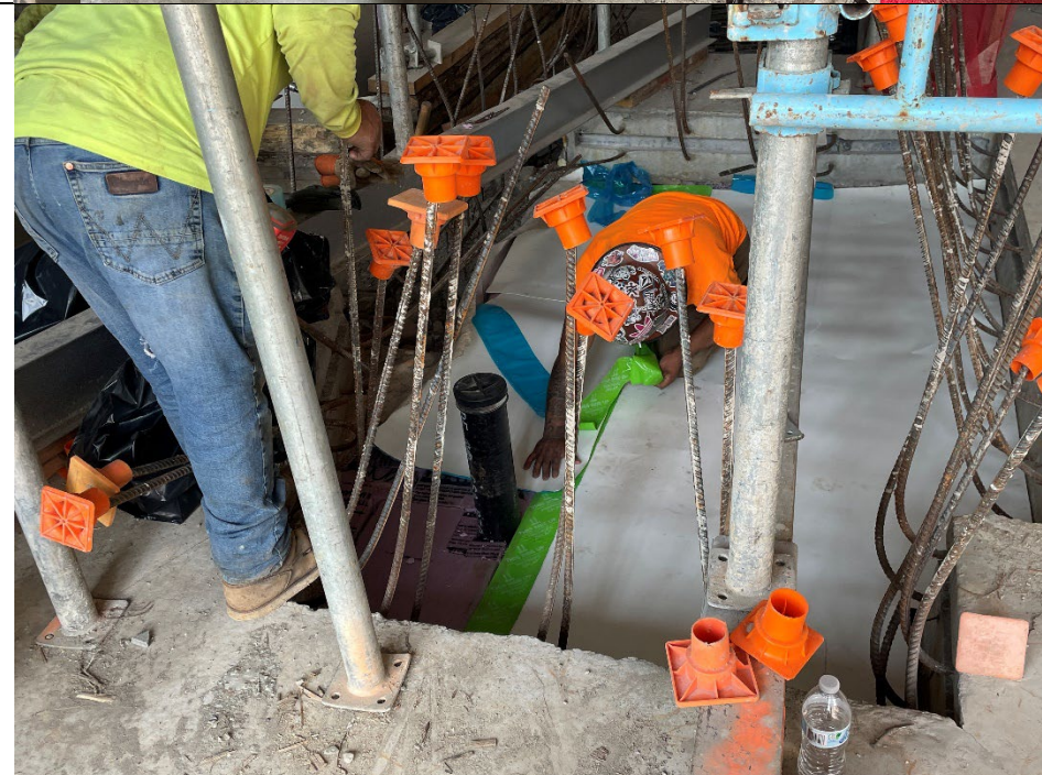
Photo 2: Facing northwest, view of an exposed pit requiring further vapor barrier installation.
