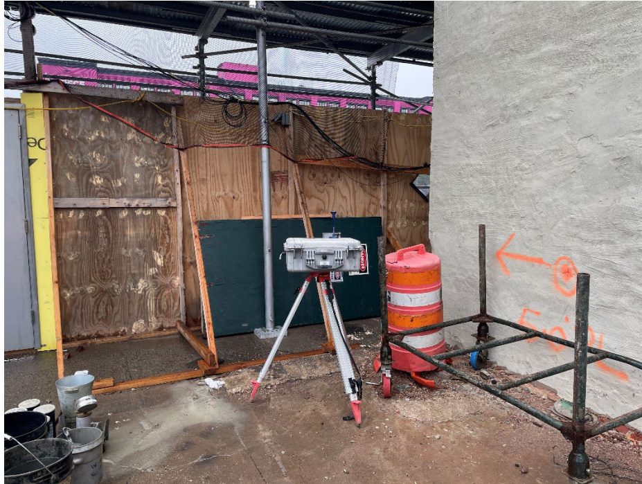
Photo 1: Facing southeast, view of the upwind CAMP station.
