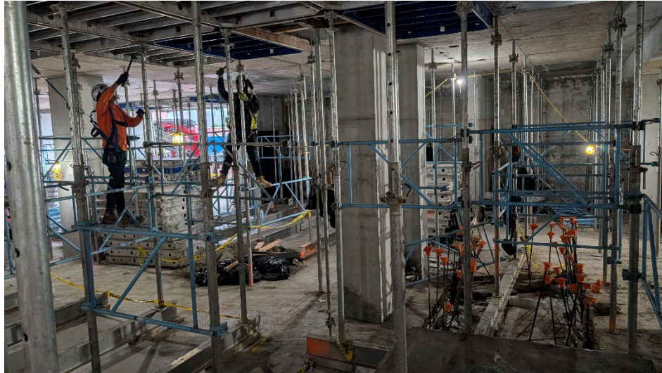
Photo 3: Facing northeast, view of last remaining pit and workers removing concrete forms.
