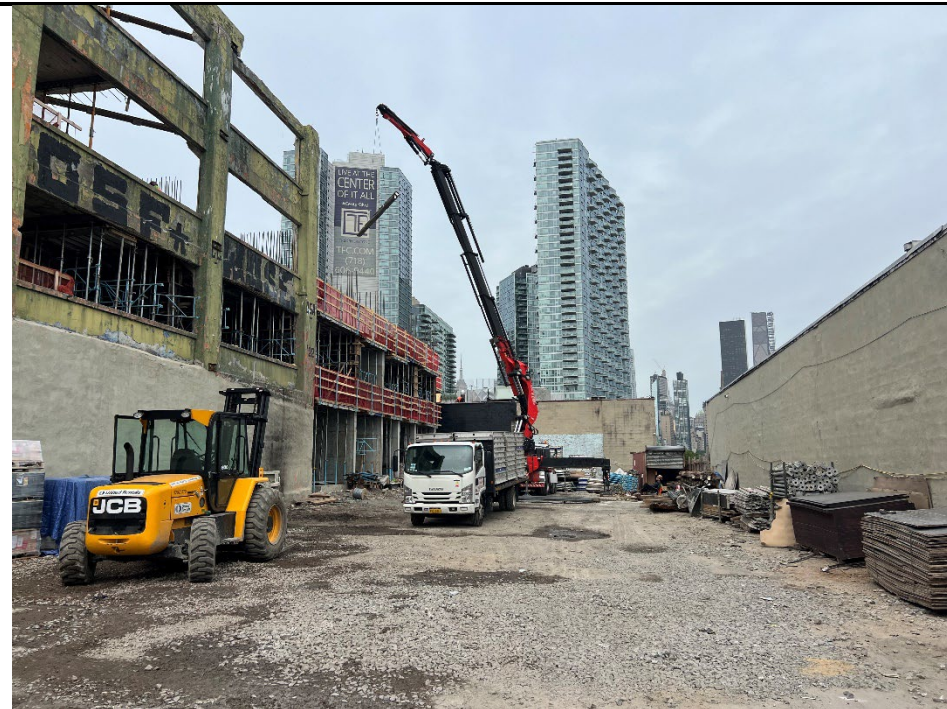
Photo 1: Facing west, view of NYC Axon bringing rebar to the second floor.
