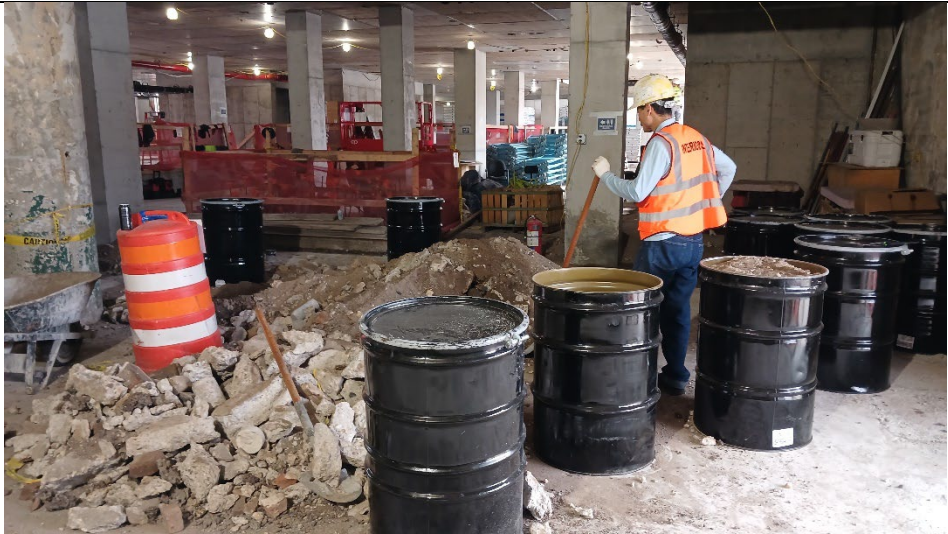
Photo 2: Facing northwest, loading stockpiled soil from the utilities trench into 55-gallon drums, pending analysis and export.
