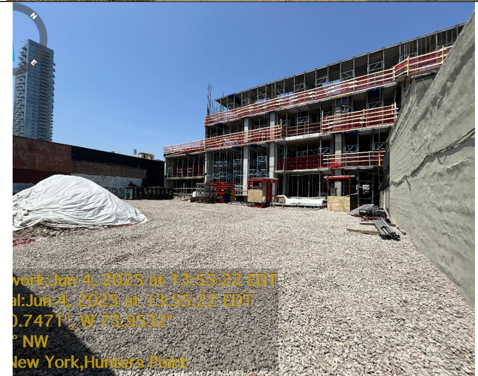
Photo 2: Facing northwest, view of Site cover system in the southern region of the Site.
