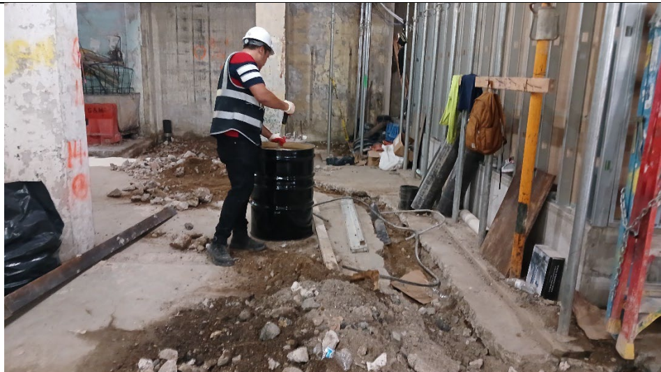
Photo 2: Facing south, loading stockpiled soil from the utilities trench into 55-gallon drum, pending analysis and export.
