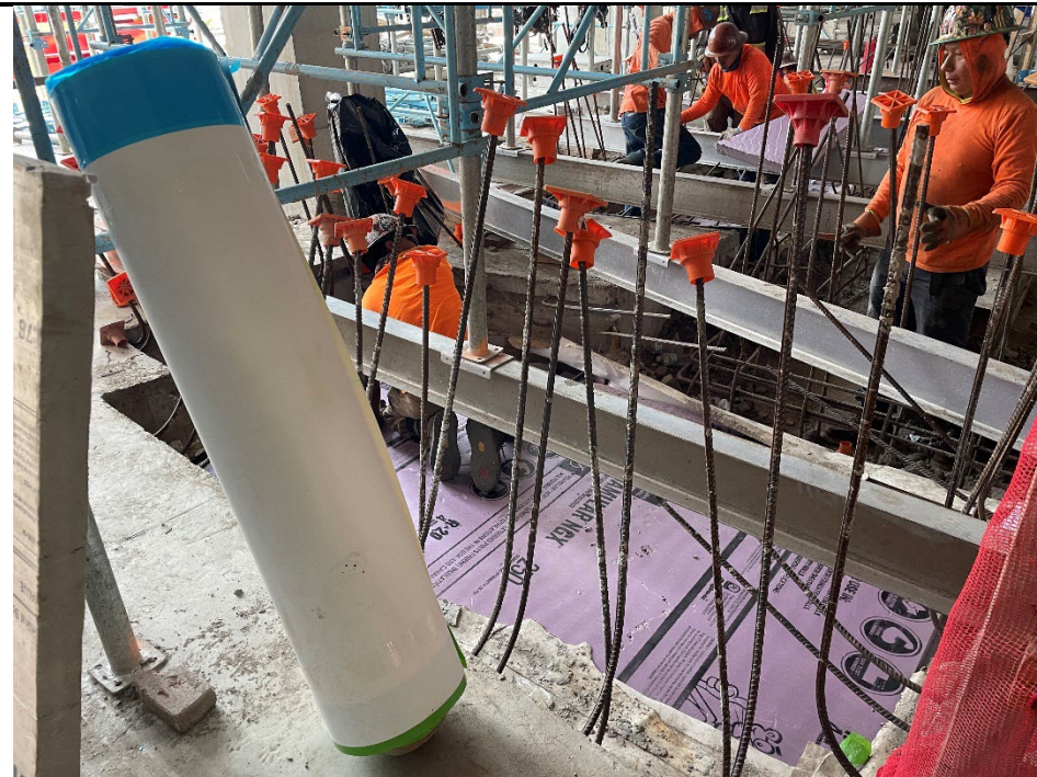
Photo 1: Facing southwest, view of NY Axon laying Styrofoam within the unpoured foundation slab sections.
