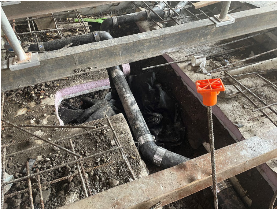
Photo 2: Facing west, view of SSDS piping wrapped in geotextile fabric beneath plumbing utilities.
