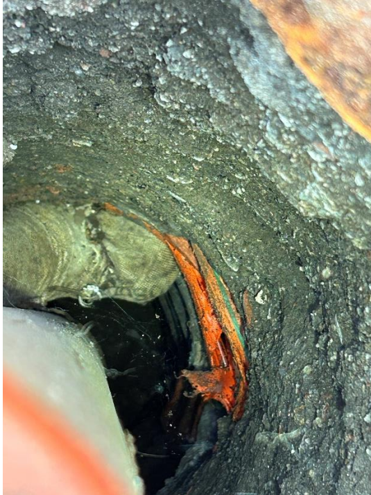
MW-17 with no visible backfill, petroleum sock, and cut wire insulation with no visible wires.
