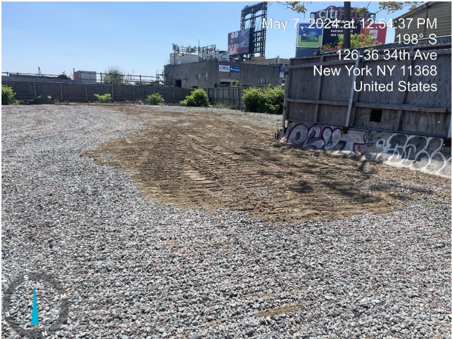
Photo 3: View disturbed site cover system in the northwest portion of the site (facing southwest).
