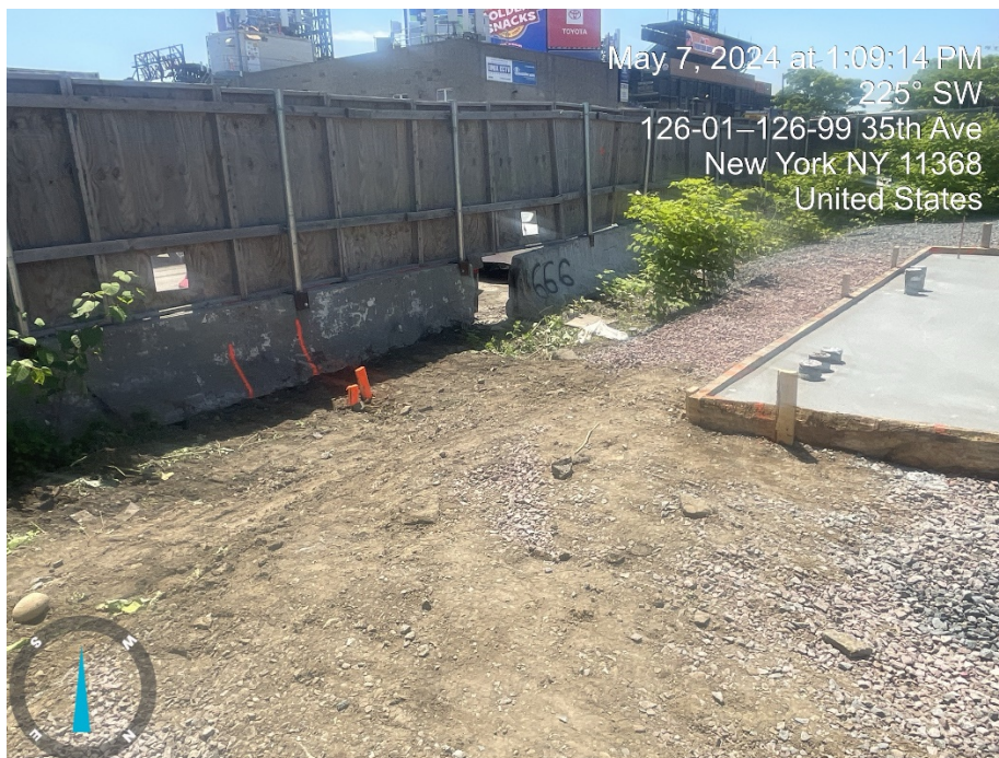
Photo 2: View of trenched area where temporary electrical utilities were installed (facing southwest).
