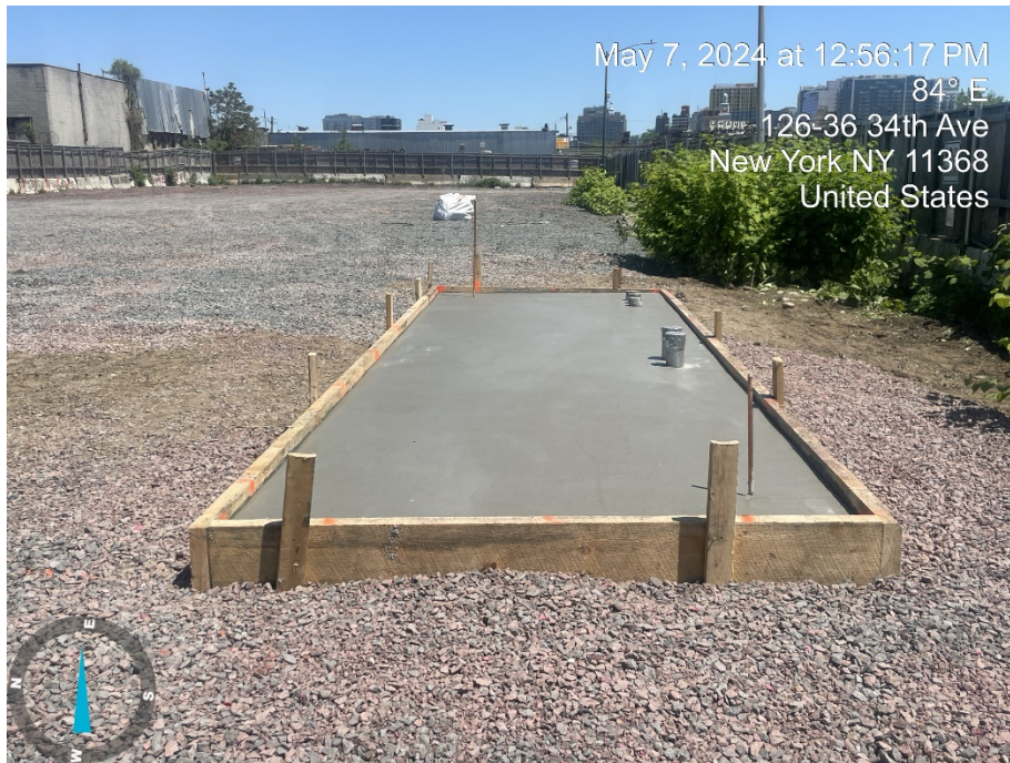
Photo 1: View of concrete slab installed in the southwest portion of the site (facing east).
