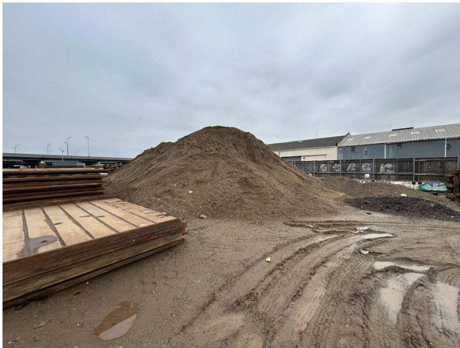
Photo 8: View of imported clean fill material stockpiled on the eastern part of the site, facing northeast (2/19/2026)
