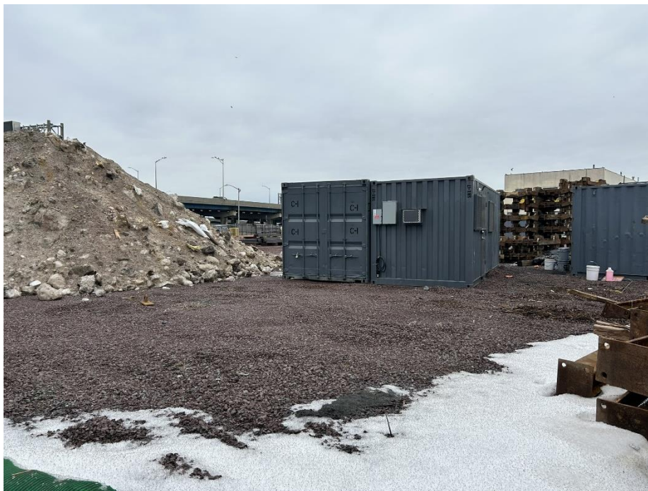
Photo 10: View Conex boxes and snow pile staged on the western part of the site, facing northeast (2/19/2026)
