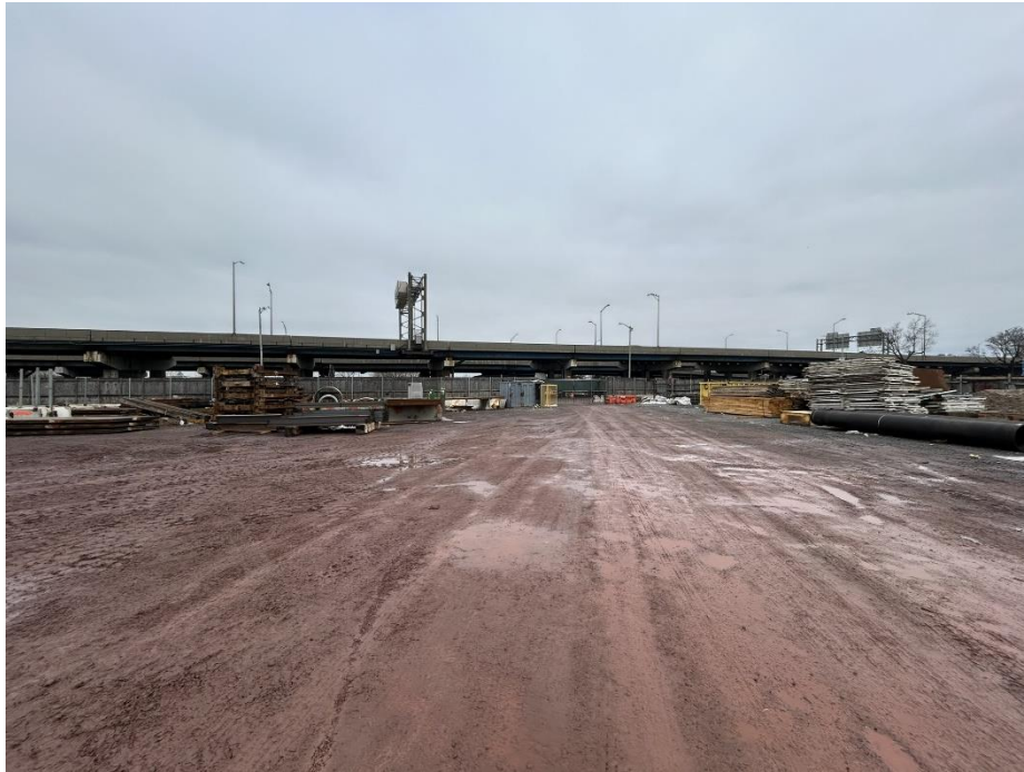
Photo 5: View of composite cover condition in the central part of the site, facing north (2/19/2026)
