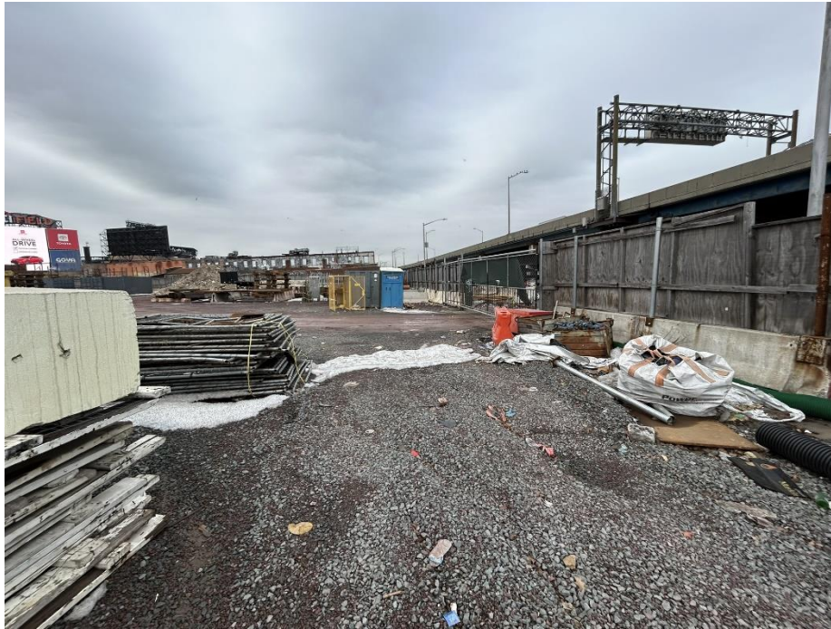
Photo 7: View of composite cover condition and construction materials staged on the northern part of the site, facing east (2/19/2026)
