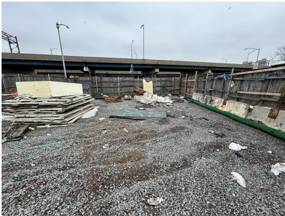
Photo 4: View of composite cover condition, fencing, and construction materials staged in the northeastern part of the site, facing northeast(2/19/2026)
