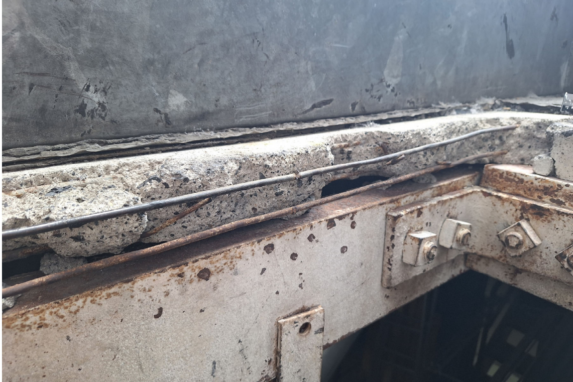
Photo 5. Detail view of exposed wire reinforcement of precast concrete planks.
