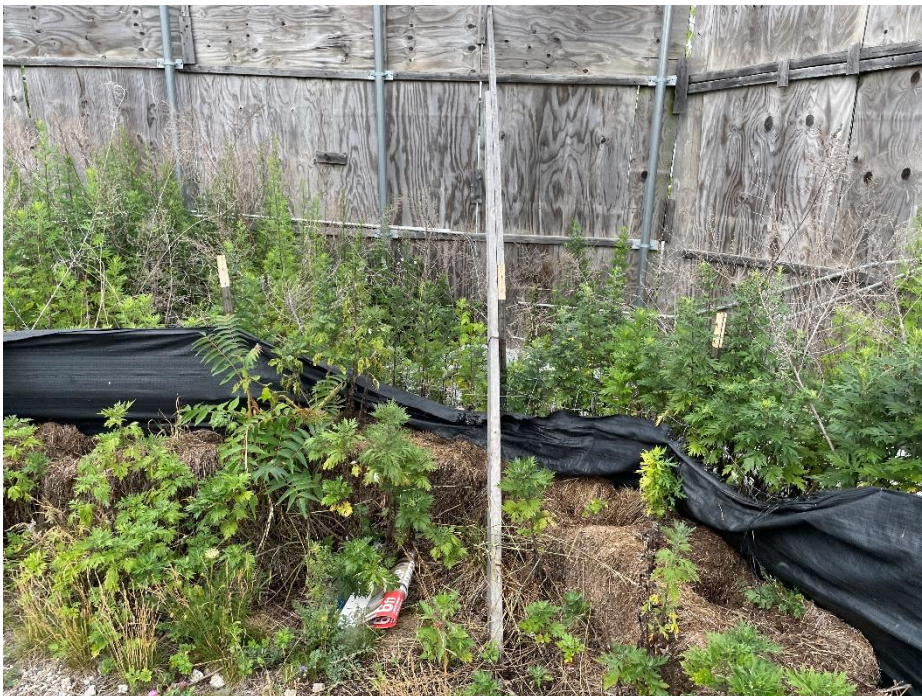
Photo 6: View of damaged sediment/erosion fence and degraded hay bales along the northeastern site boundary, facing north (taken on 06/27/23)
