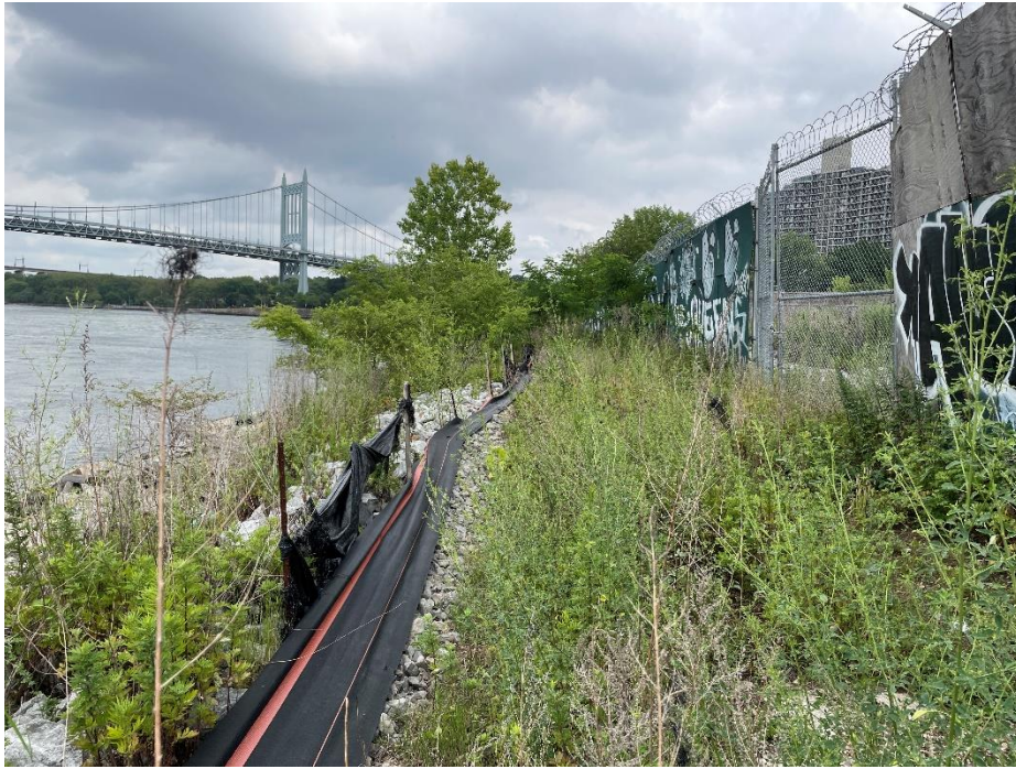
Photo 7: View of detached silt fencing along the river edge, facing east (taken on 06/27/23)
