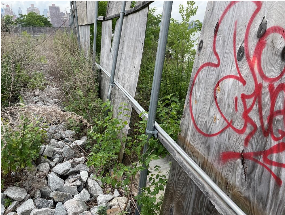
Photo 3: View of rip rap cover and damaged perimeter fencing along the northern site boundary, facing west (taken on 06/27/2023)
