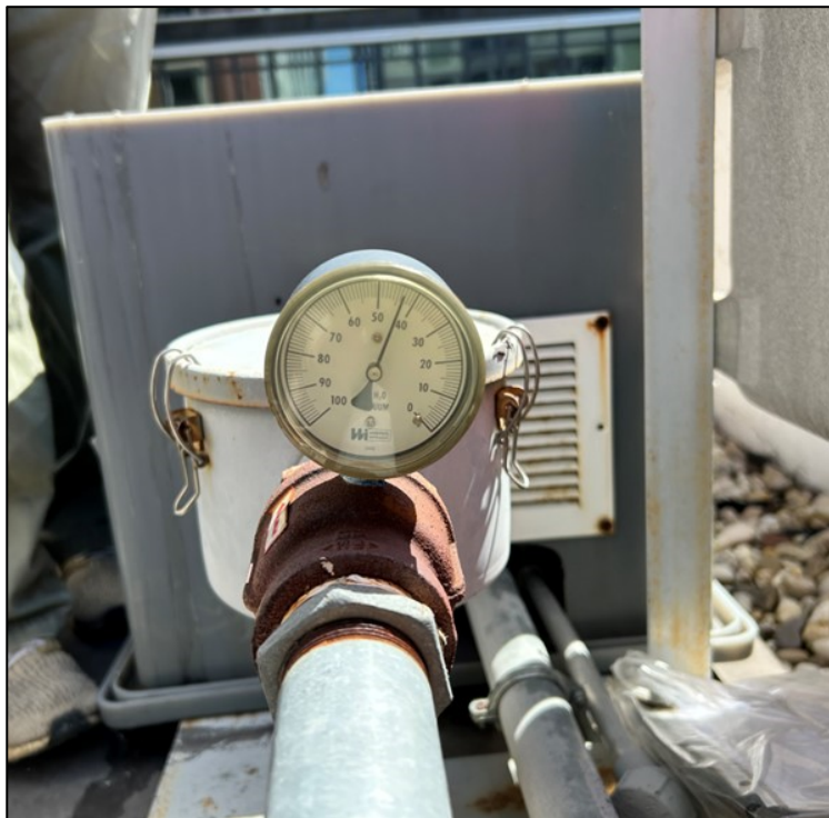
Photo 4, 05/28/2024: View of vacuum gauge connected to roof blower (facing east).
