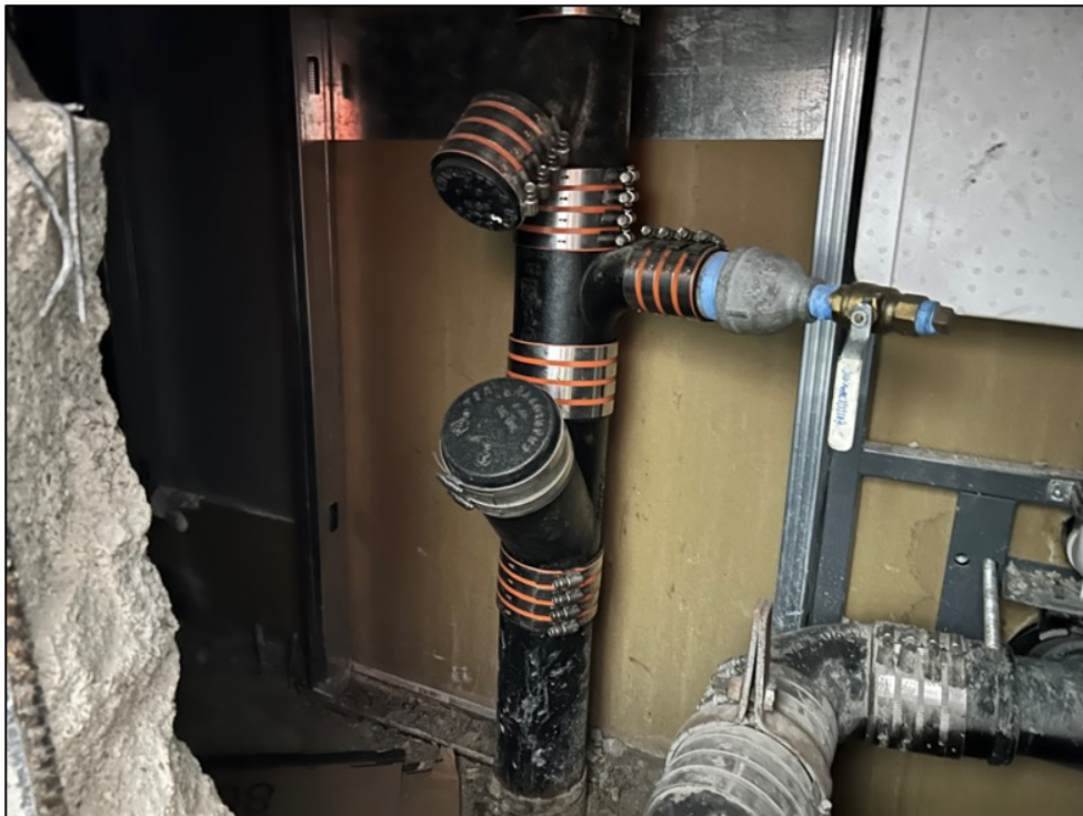
Photo 2, 05/28/2024: View of submembrane depressurization (SMD) system riser pipe penetration through the cellar slab (facing west).
