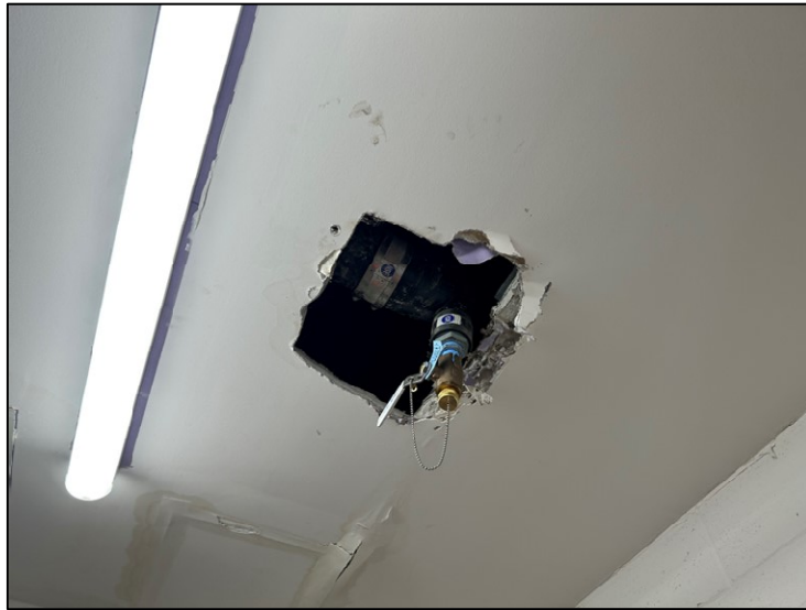
Photo 25, 05/28/2024: View of the clean out valve installed to remove water from the SMD system (facing south).
