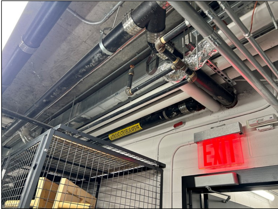
Photo 15, 05/28/2024: View of labeled SMD piping in storage room (facing northeast).
