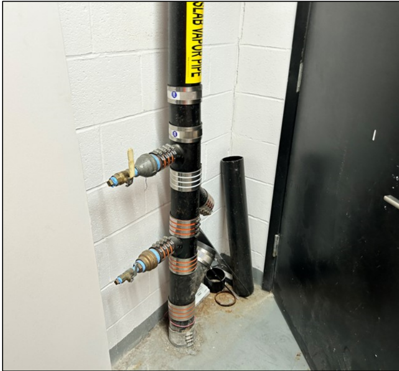
Photo 21, 05/28/2024: View of SMD riser behind maintenance hallway wall panel.
