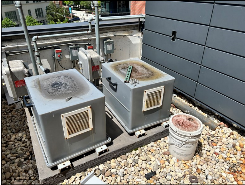
Photo 3, 05/28/2024: View of blower units on roof (facing northwest).
