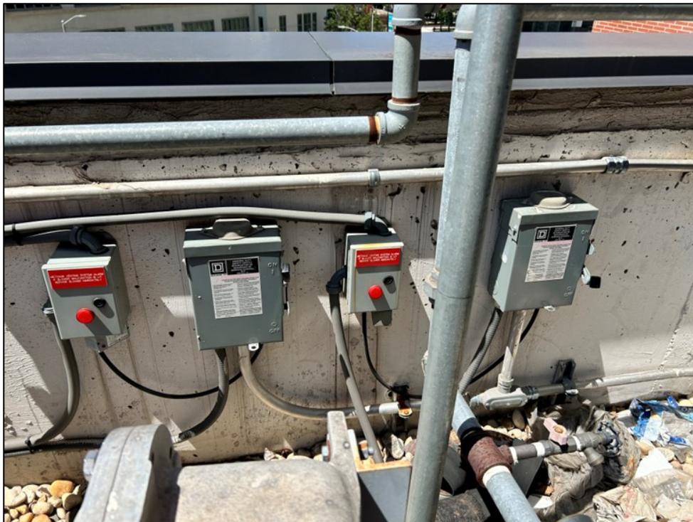
Photo 24, 05/28/2024: View of SMD system breaker and alarm panels (facing west).
