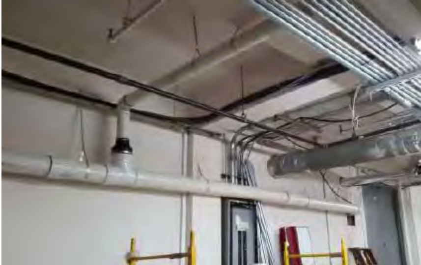
Photo 6 – View of ceiling suspended piping for SVE system.
