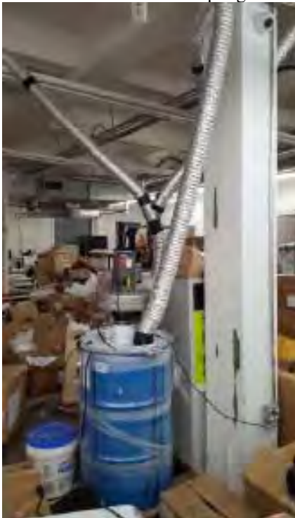
Photo 2 – View of temporary carbon filtration system installed on 1 st floor.
