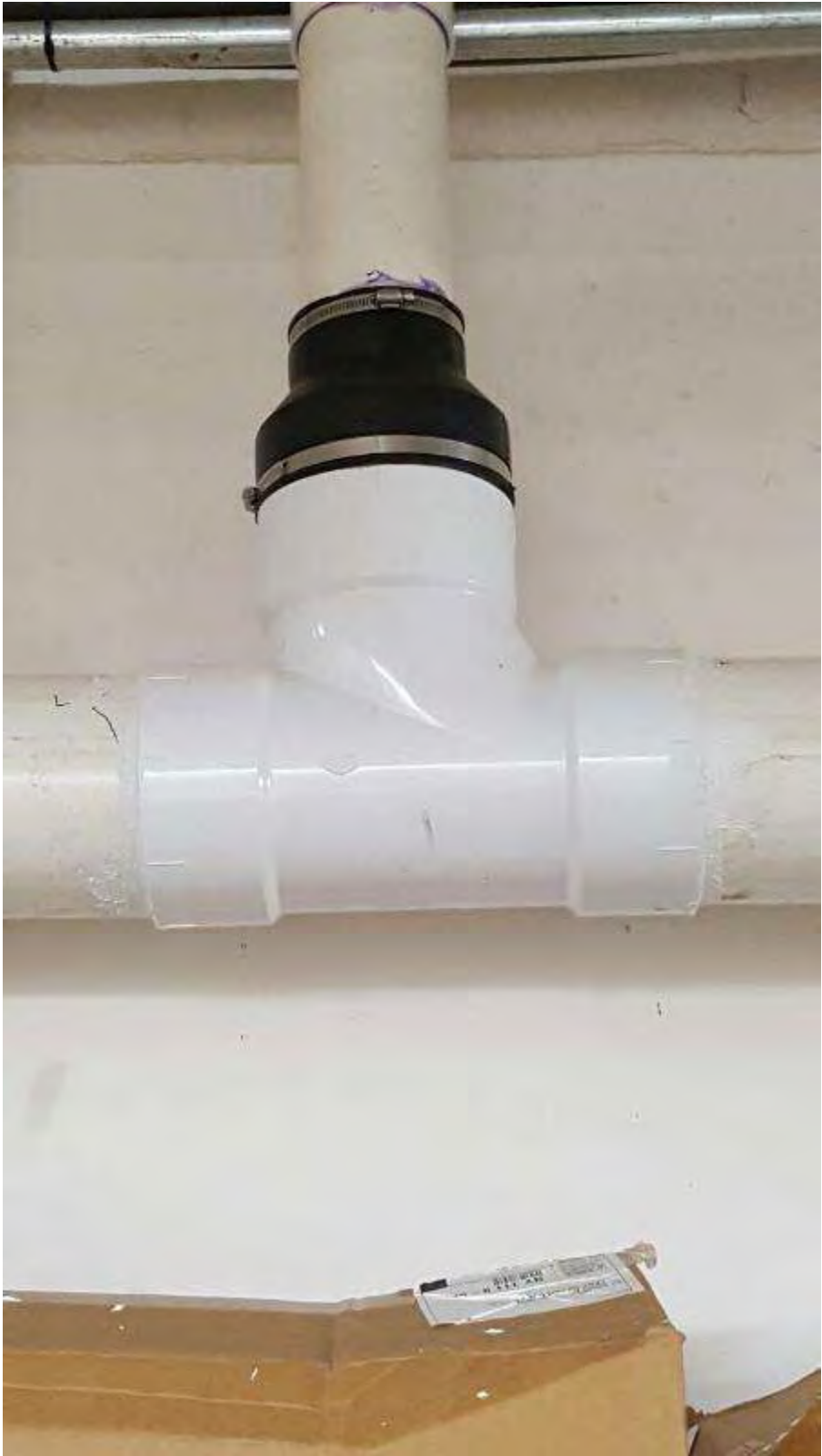
Figure 5 Rear wall / VE4 "T"
