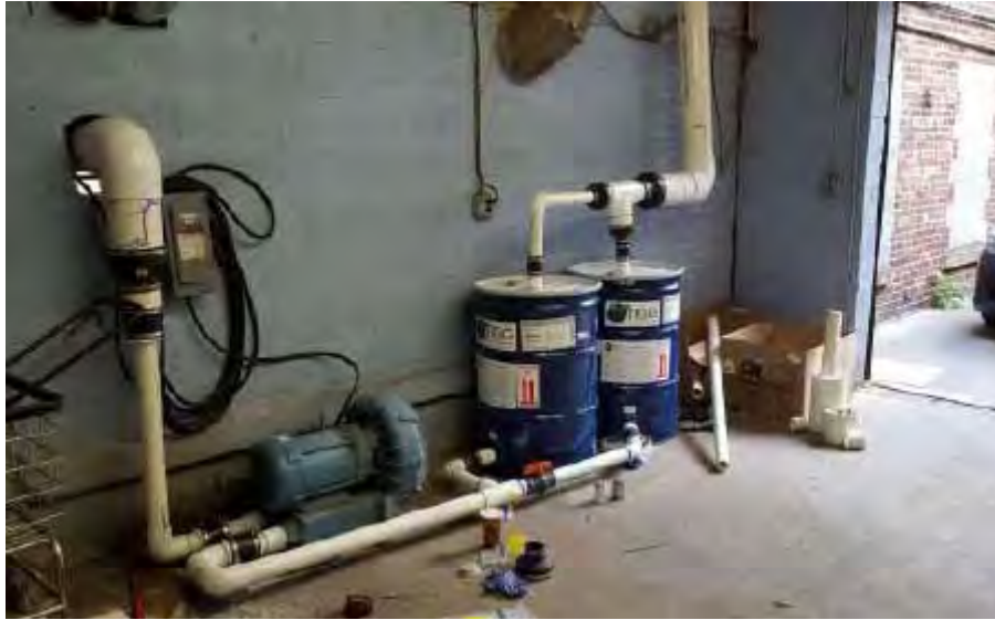
Photo 7 – View of SVE fan and carbon drums.
