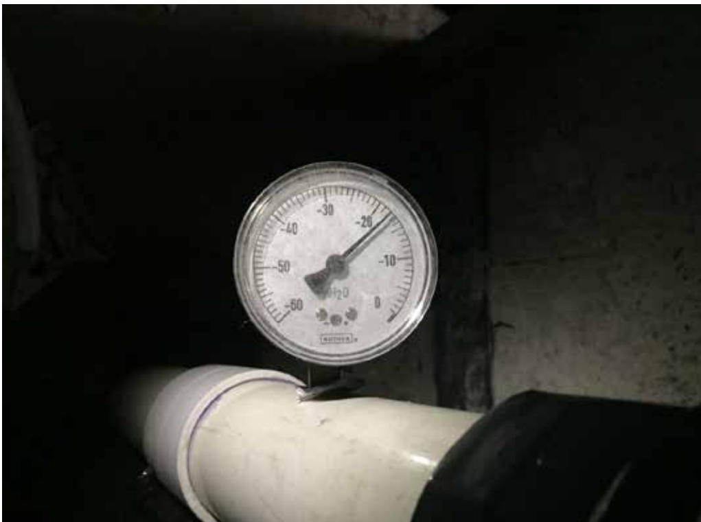
Photo 6: VE-1 vacuum dial showing -18 inches of water gauge.
