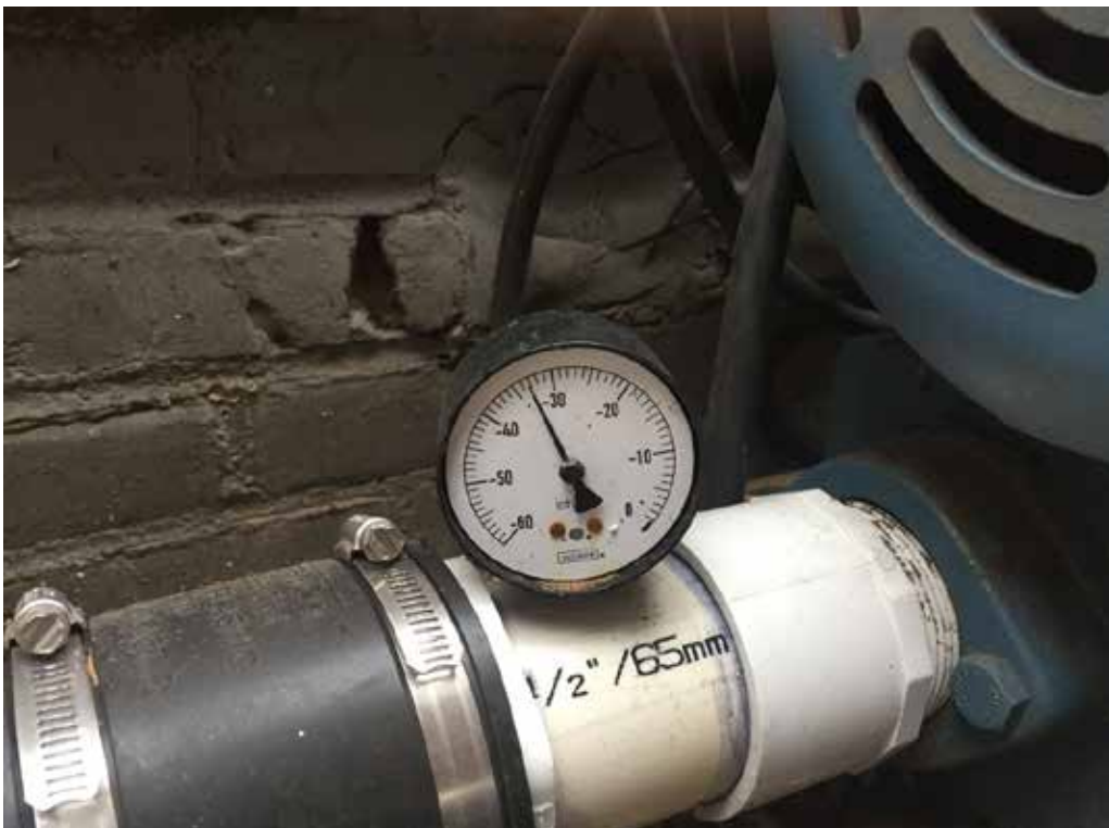
Photo 2: Blower unit inlet vacuum dial showing -33 inches of water gauge.
