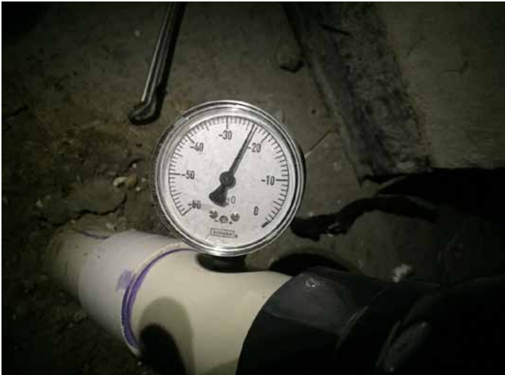
Photo 5: VE-4 vacuum dial showing -24 inches of water gauge.
