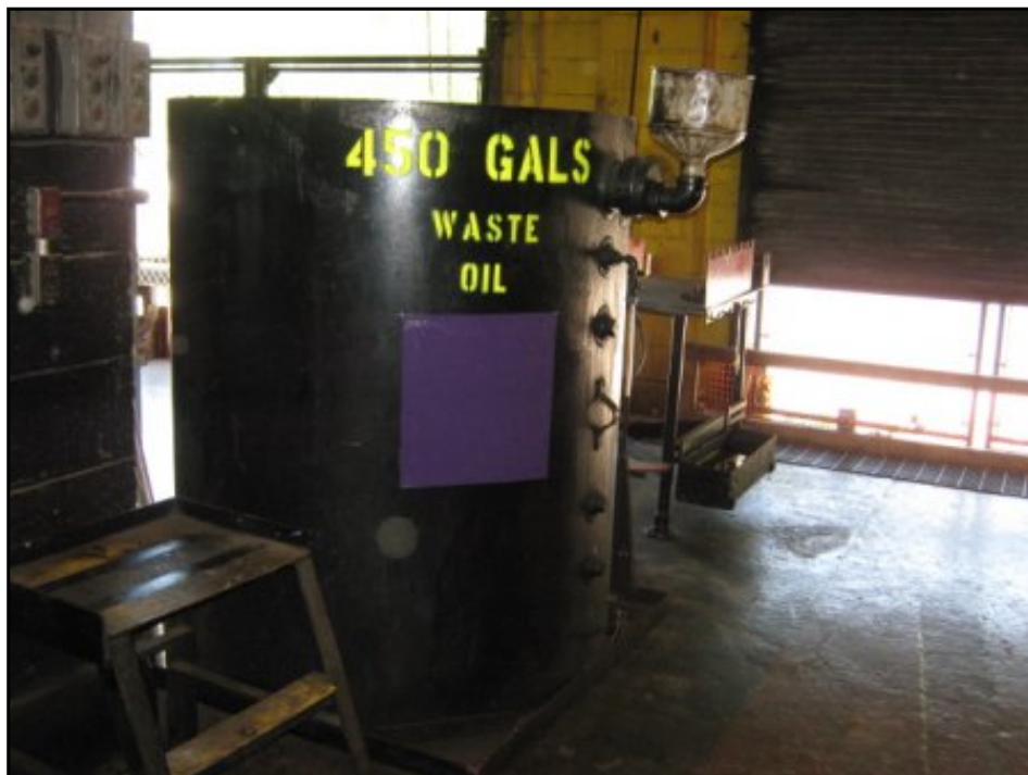
500-gallon waste oil AST at power plant
