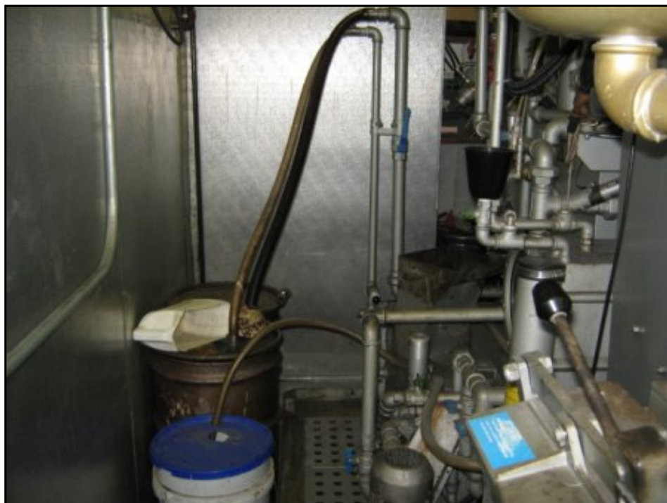
Rear of dry cleaning machine
