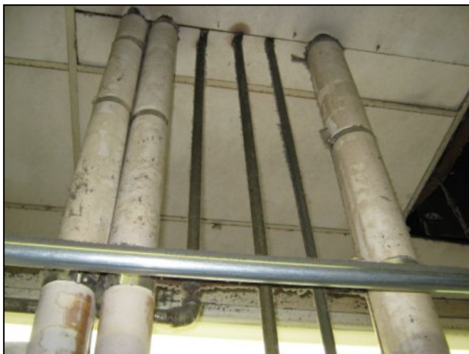
Asbestos-containing pipe insulation at HIP Cleaners
