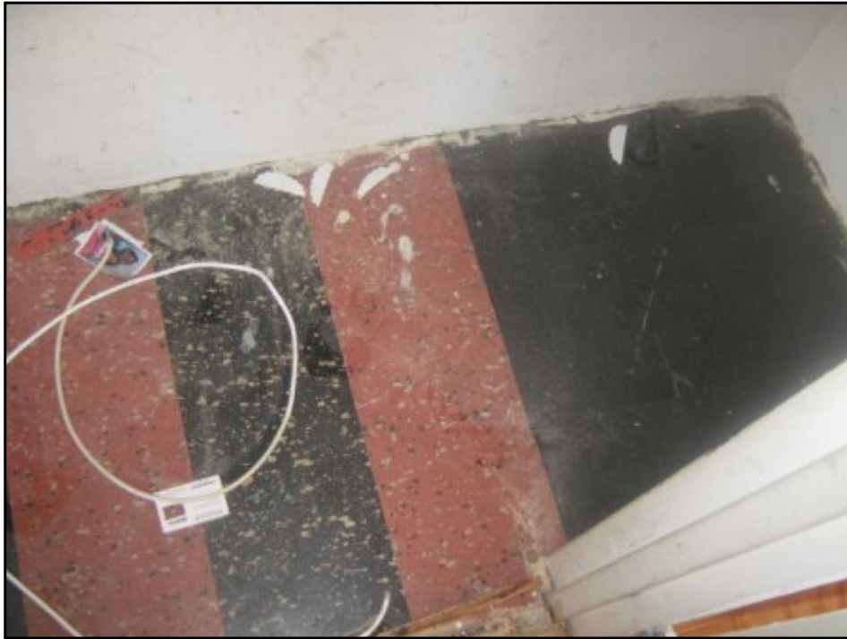
Asbestos-containing vinyl floor tiles Building 10C Unit 12A
