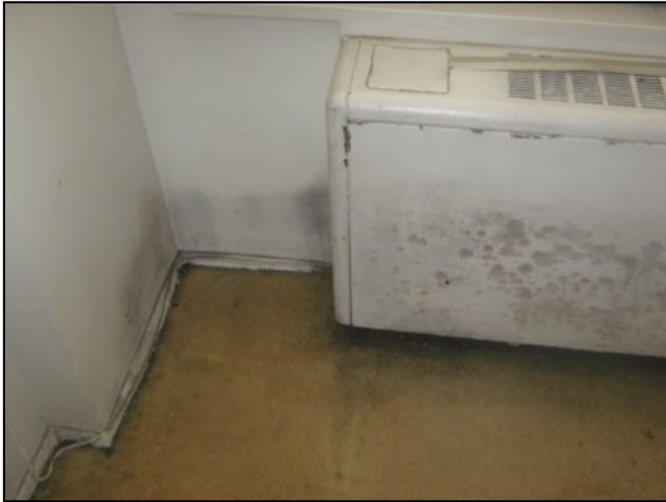
Potential mold in Building 13A Unit 13D
