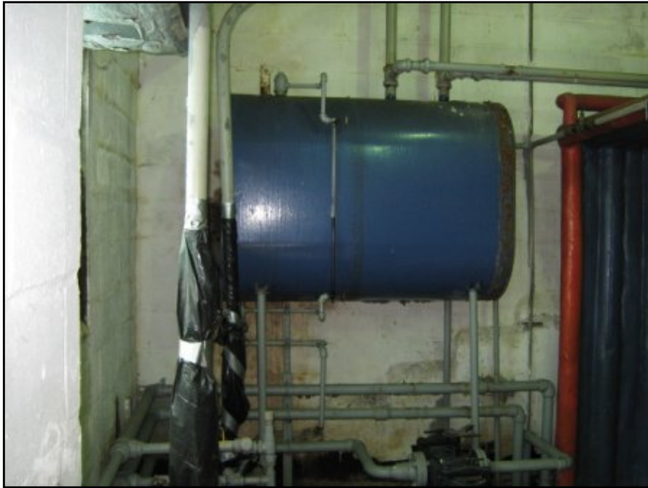
275-gallon AST in pump room at power plant
