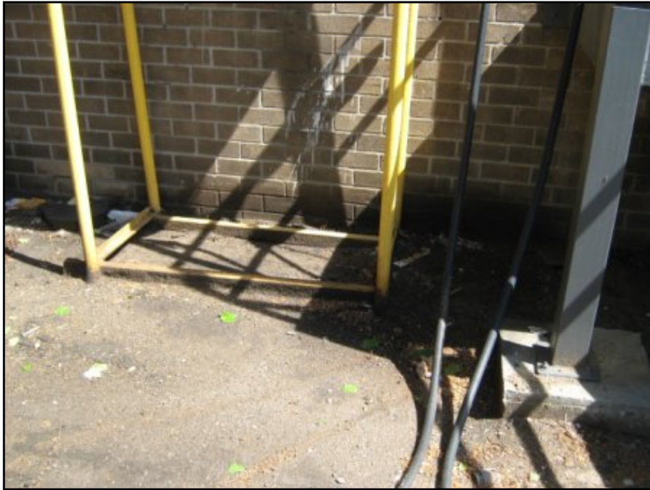
Staining beneath 275-gallon diesel AST
