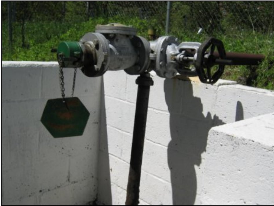
One of the fill ports
