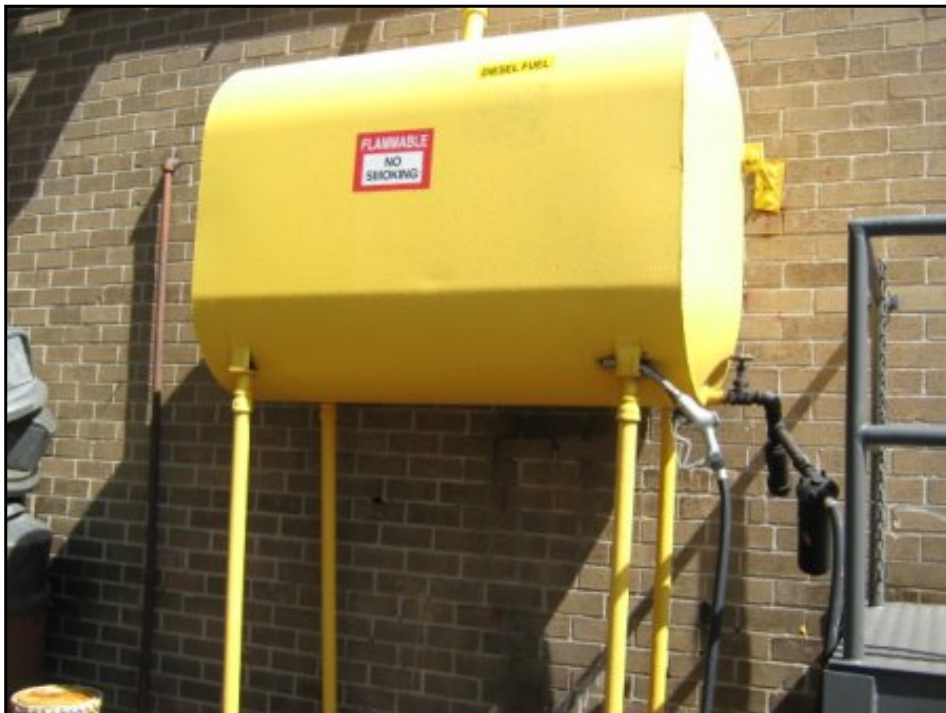
275-gallon diesel AST at maintenance building
