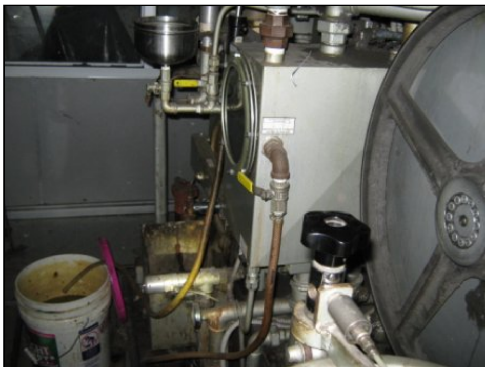
Rear of dry cleaning machine at JS Rochdale Cleaners
