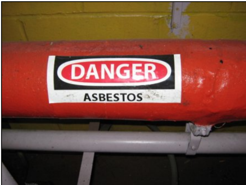
Encapsulated asbestos-containing materials at power plant
