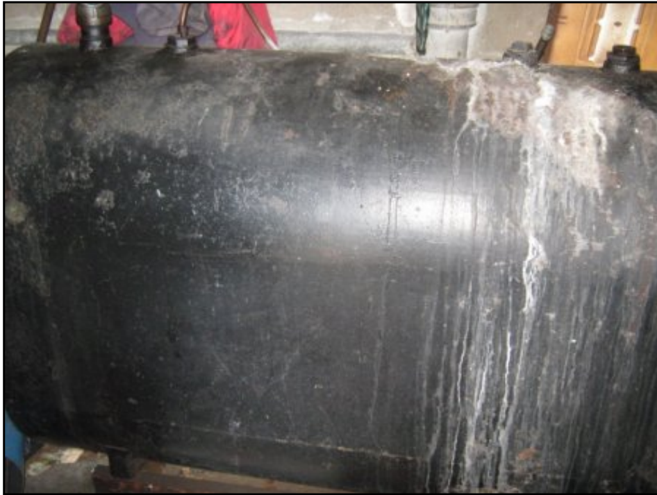
275-gallon fuel oil AST at gasoline station
