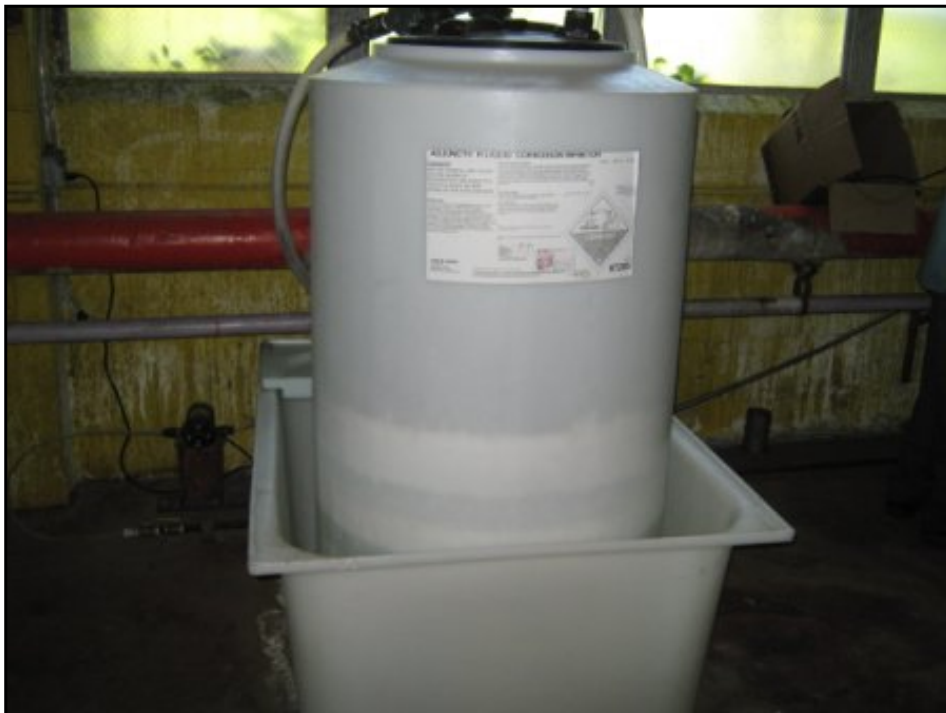
Water treatment chemicals at power plant
