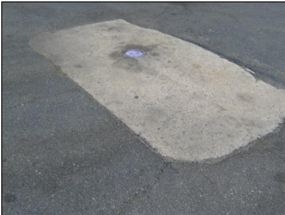
Waste oil UST at gasoline station
