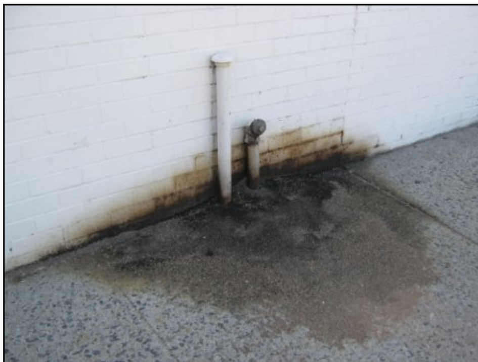
Fill and vent at rear of OB's Bakery
