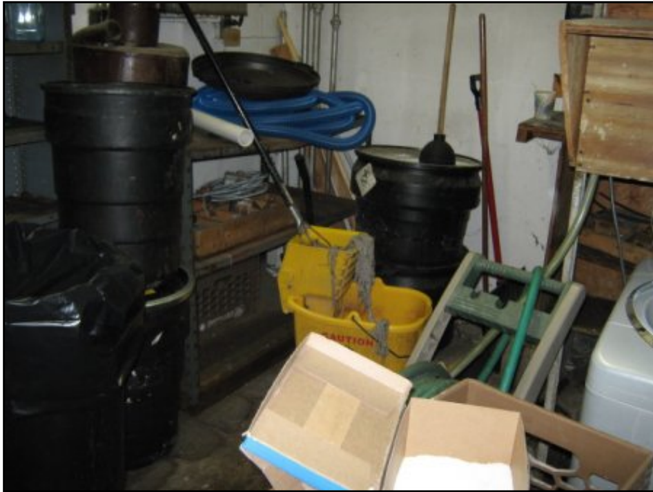
Waste storage containers above damaged flooring
