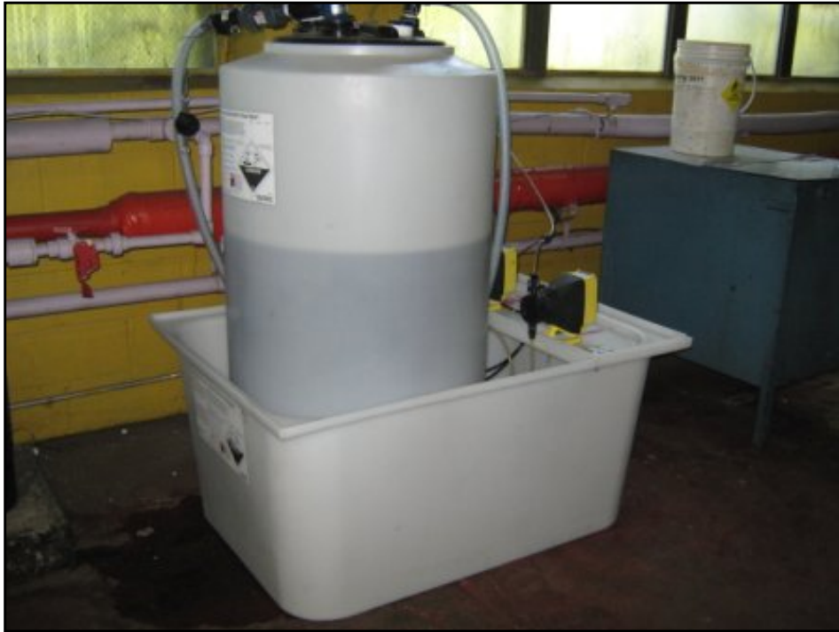
Water treatment chemicals at power plant
