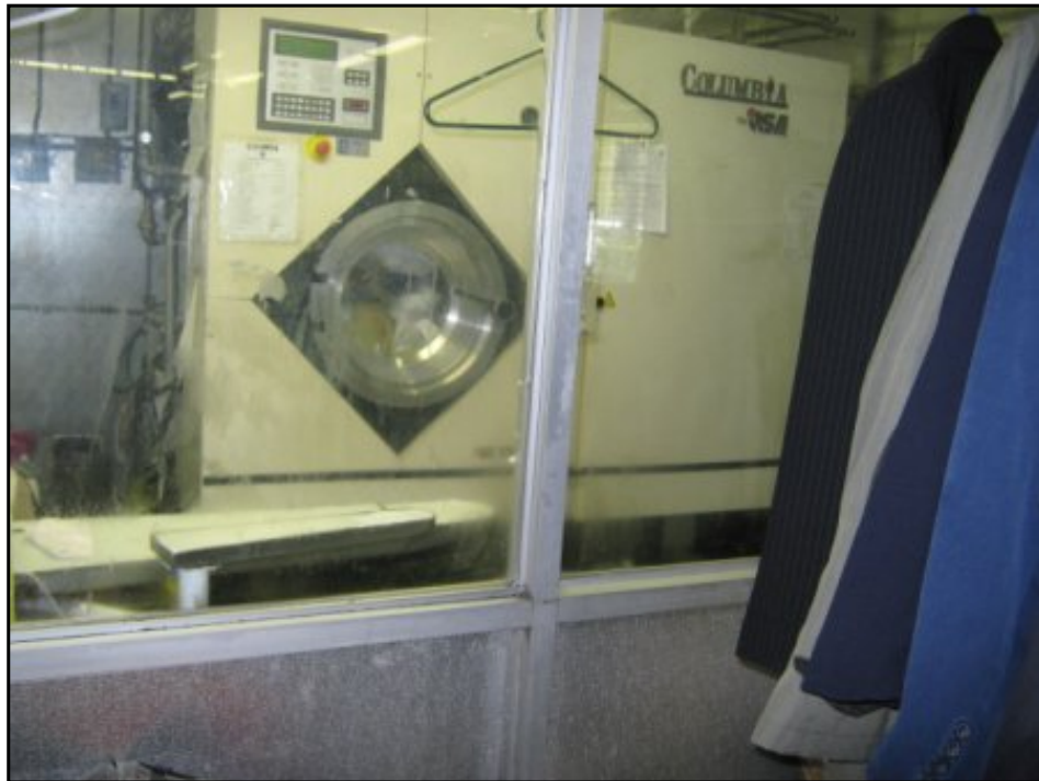
Dry cleaning machine at HIP Cleaners
