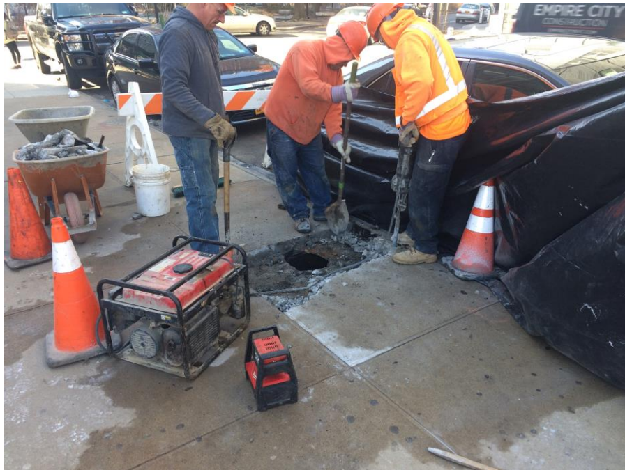
Photo 1: View of the hole in the 41 st Avenue sidewalk where the fill port was previously located (facing southwest).
