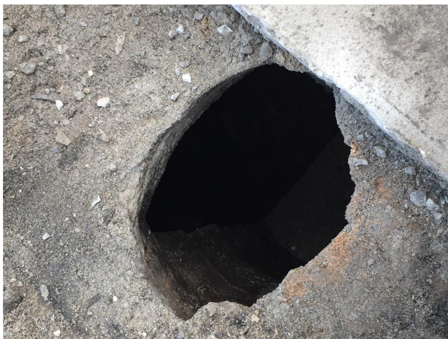
Photo 2: View of hole located beneath the abandoned fuel oil fill port in the 41 st Avenue sidewalk. (2/28/2017)
