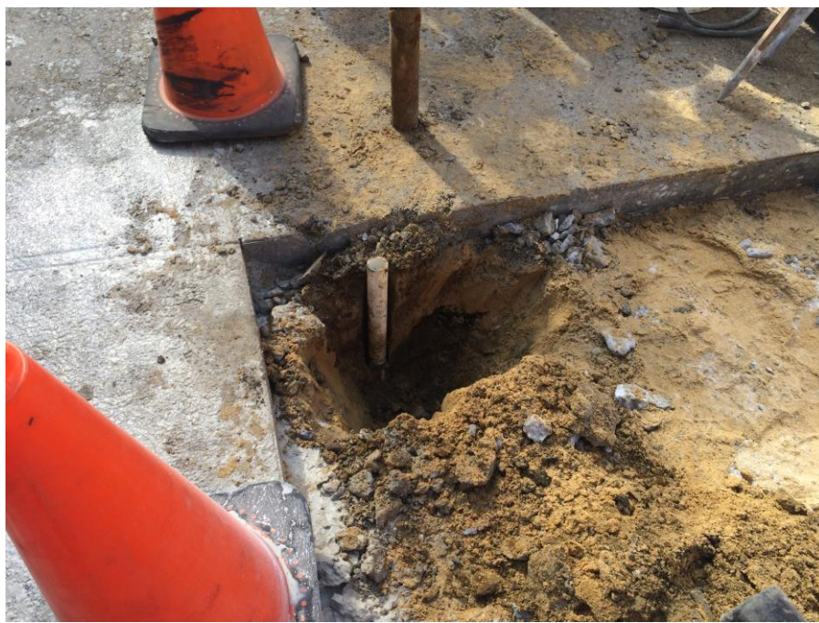
Photo 2: View of the PVC pipe that was attached to the fill port
