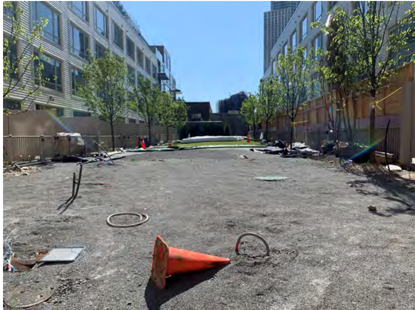
1. Cover system consisting of imported clean soil and crushed stone, exterior courtyard area
