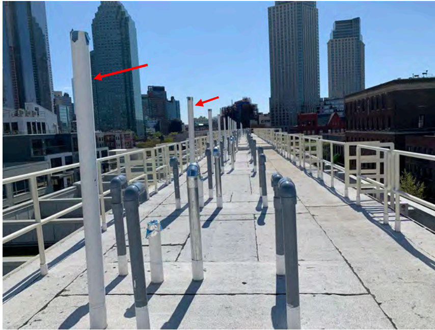
7. SSDS roof riser pipes at units 113 to 130, along 46 th Avenue
