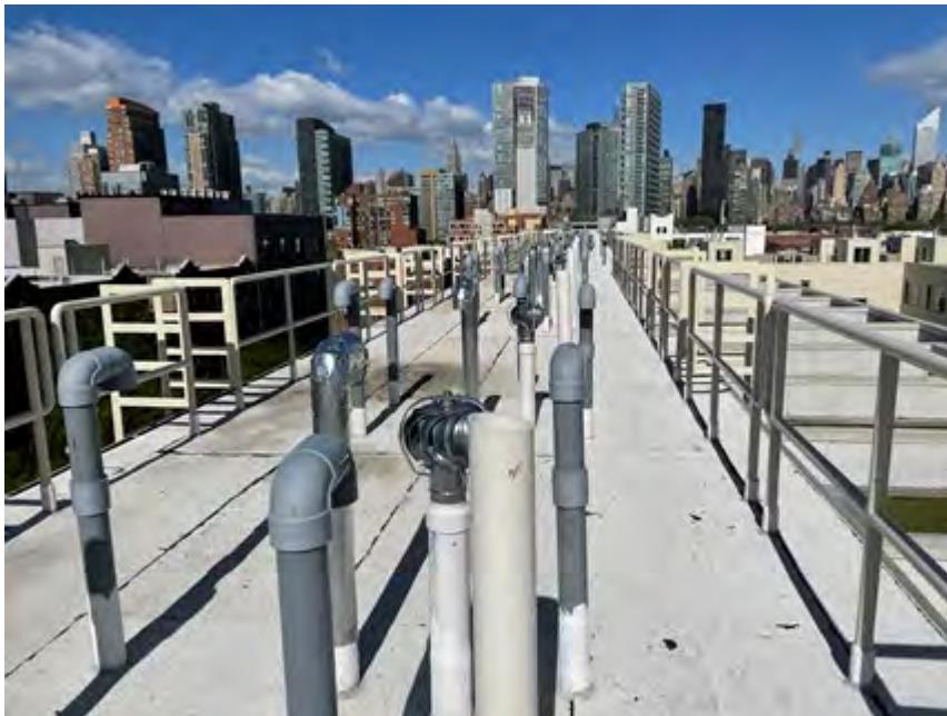
8. SSDS roof wind turbines at units 113 to 130, along 46 th Avenue
