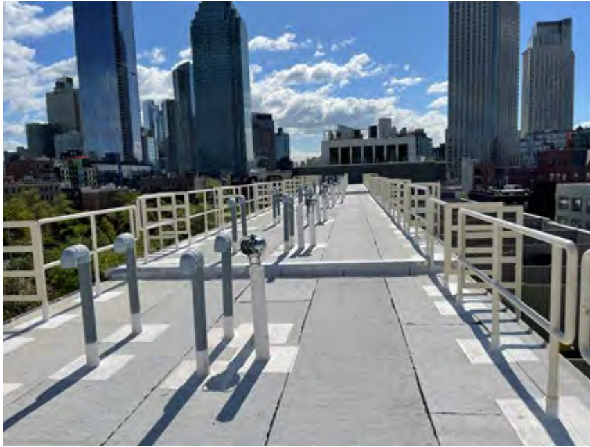
7. SSDS roof wind turbines at units 139 through 150, along 45th Road
