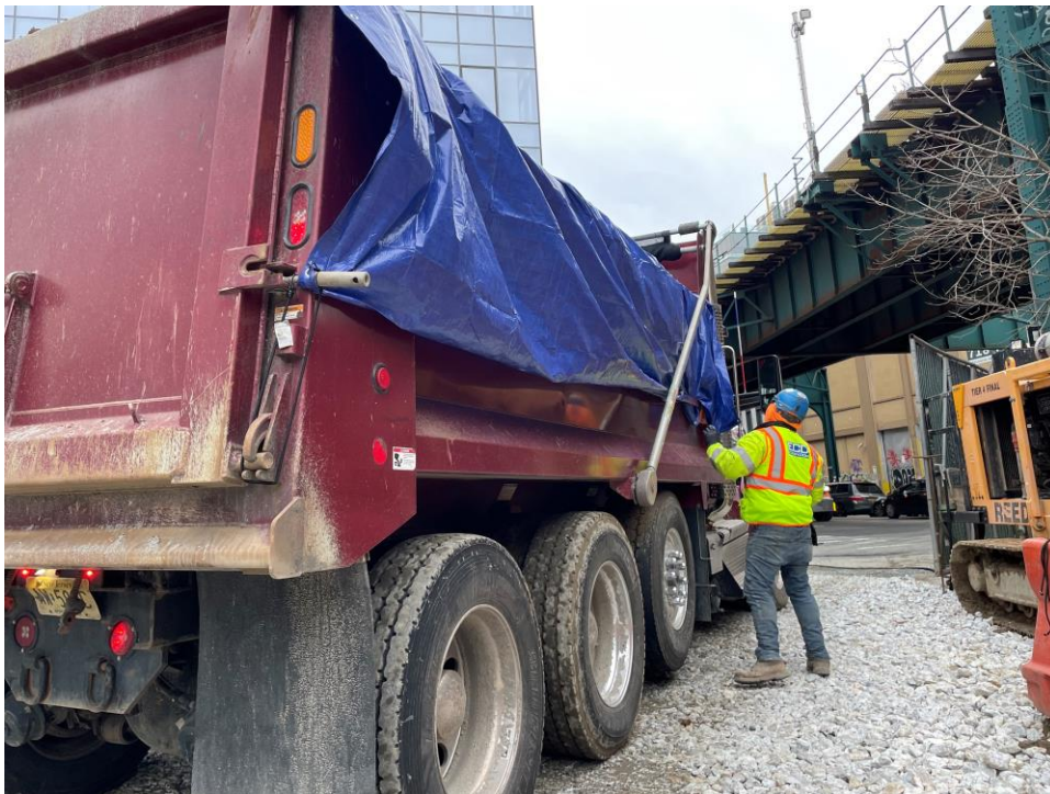
Photo 4: ECD securing truck cover with bungee cords for export off-site (facing south).
