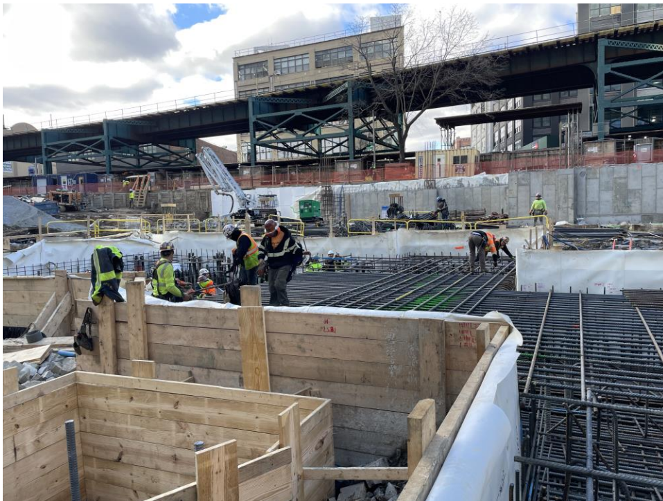
Photo 2: ECD installing rebar in the central part of the site (facing west).
