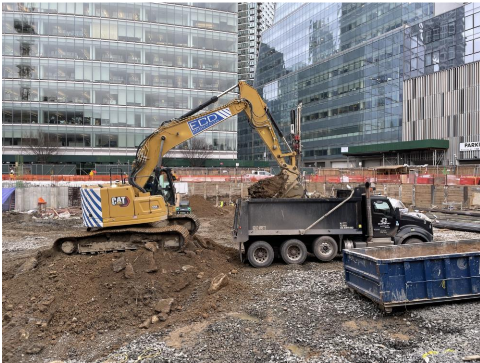
Photo 2: ECD loading a truck for off-site disposal in the southern part of the site (facing east).
