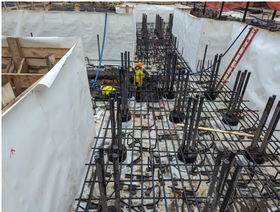
Photo 2: ECD installing waterproofing in the central part of the site (facing northeast).
