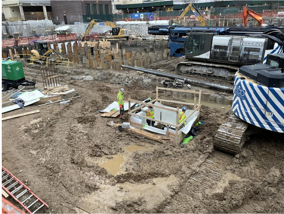
Photo 3: ECD installing waterproofing in pile caps in the western part of the site (facing northeast).
