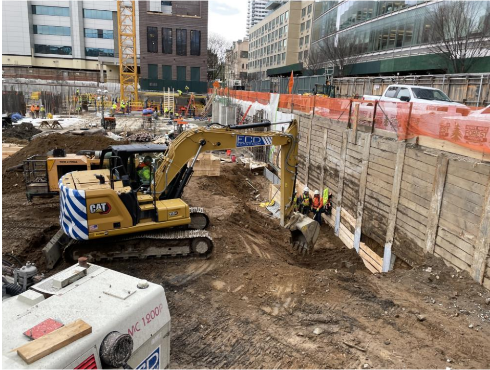
Photo 1: ECD excavating in the southeastern part of the site (WCG I, facing northeast).
