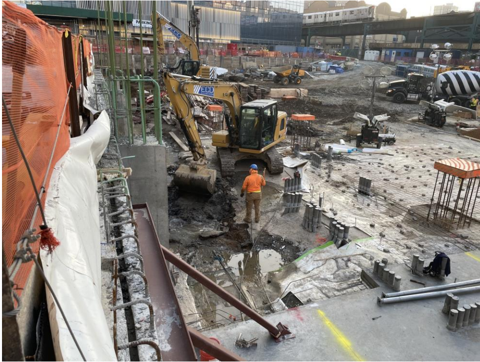
Photo 1: ECD excavating in the northeastern part of the site (WCG K, facing southwest).
