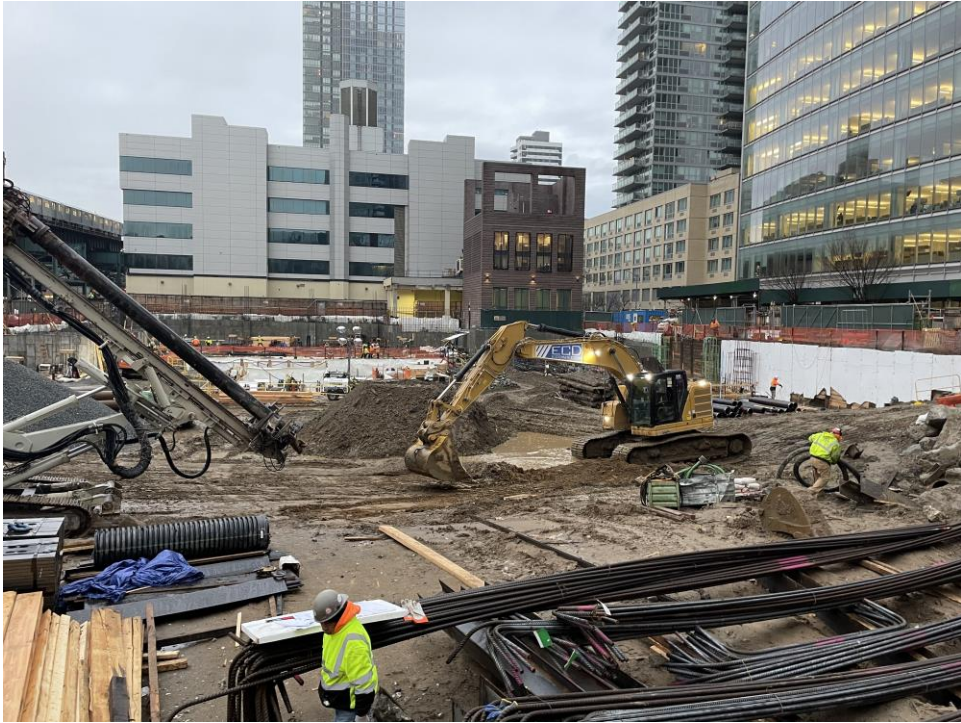
Photo 3: ECD grading material in the southern part of the site (facing northeast).
