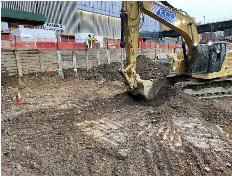
Photo 1: ECD excavating in the southeastern part of the site (WCG I, facing southwest).
