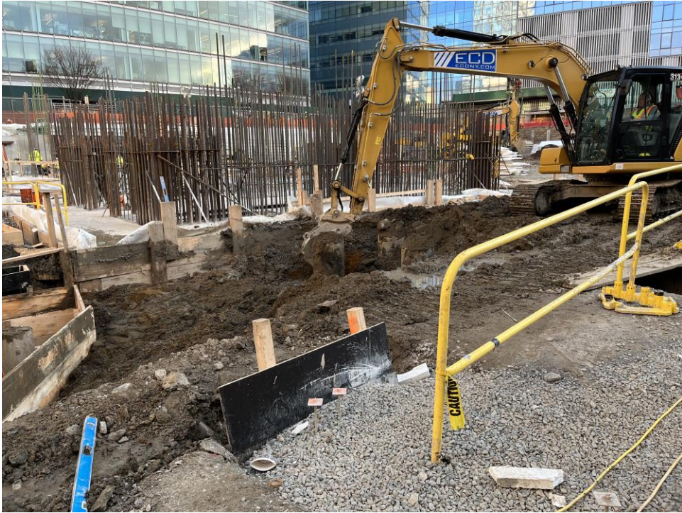
Photo 1: ECD excavating in the northwestern part of the site (WCG C, facing southeast).
