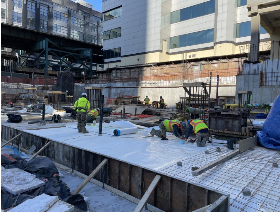
Photo 3: ECD installing waterproofing in the northeastern part of the site (facing northwest).
