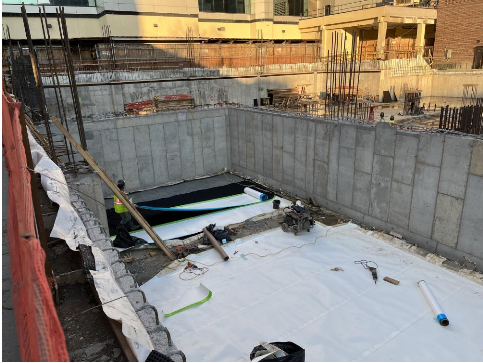
Photo 2: ECD installing waterproofing in the northwestern part of the site (facing northeast).
