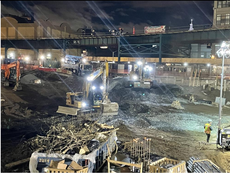
Photo 3: ECD backfilling imported stone in the southern part of the site (facing west).
