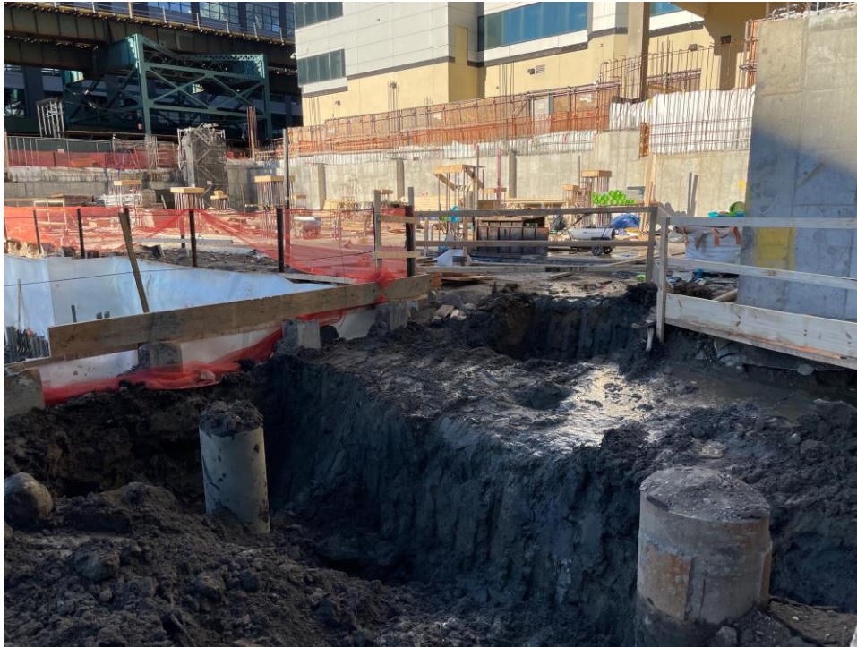
Photo 1: Excavated area in COMP H in the northeast part of the site (facing northwest).
