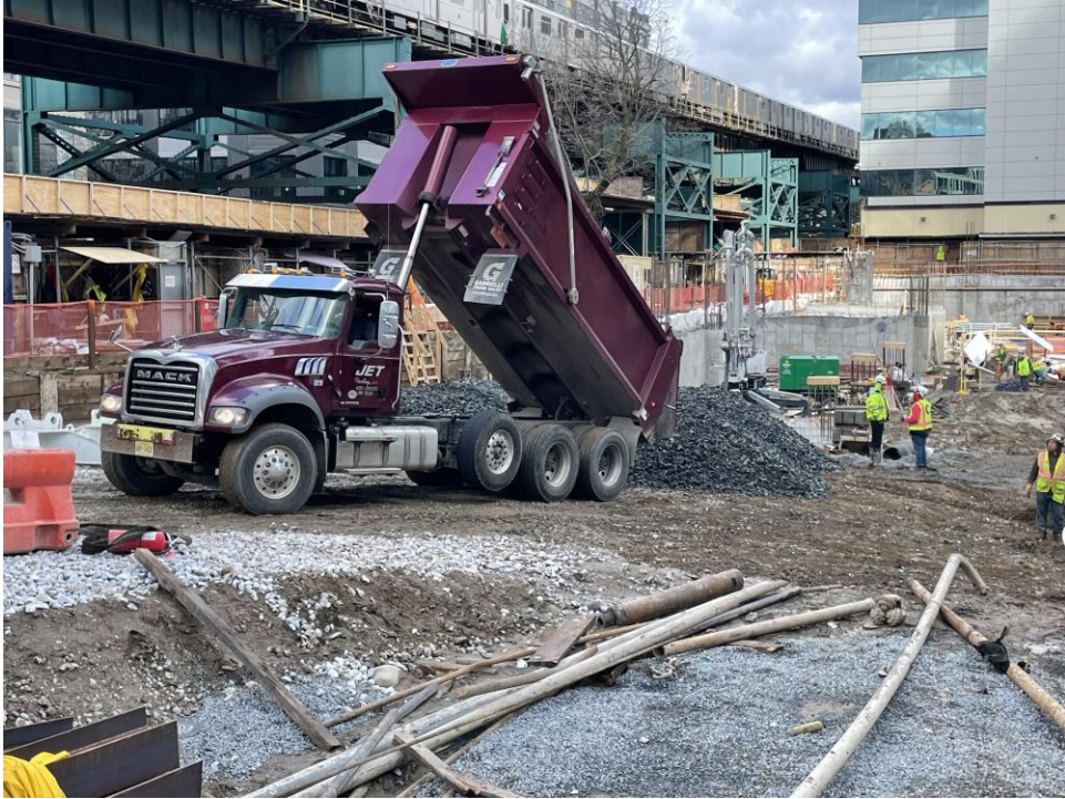
Photo 2: ECD importing 2'- 4'' tracking pad stone in the southwestern part of site (facing northwest).
