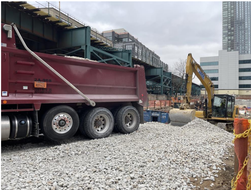
Photo 2: ECD importing stone for backfill on the site exit ramp in WCG COMP A (facing north).
