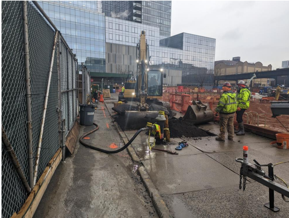
Photo 1: ECD excavating concrete off-site to the east of the site (facing southwest).
