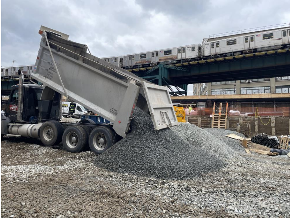
Photo 3: ECD importing 0.75-inch stone in the southwestern part of the site (facing west).
