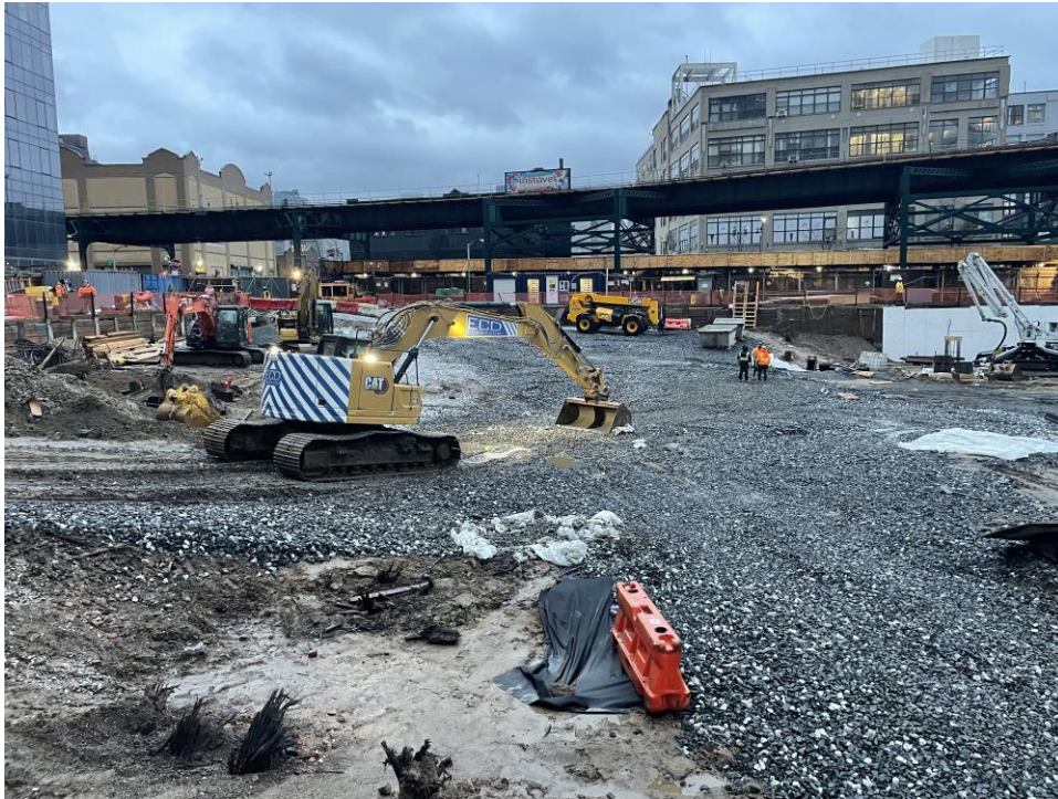
Photo 1: ECD grading in the southern part of the site (WCGs E2 and I, facing west).
