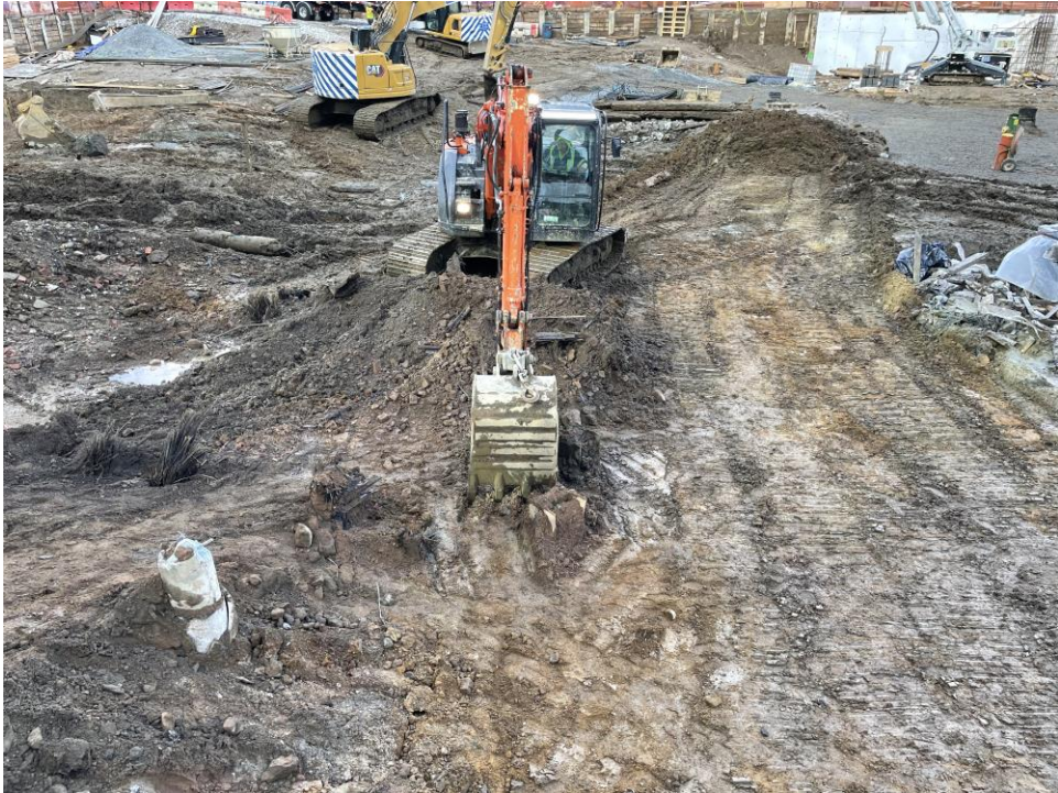
Photo 1: ECD grading in the southeast part of the site (WCG E2, facing west).
