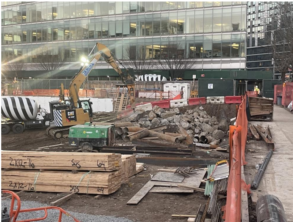
Photo 2: ECD chipping concrete in the C&D stockpile in the southeast part of the site (facing east).
