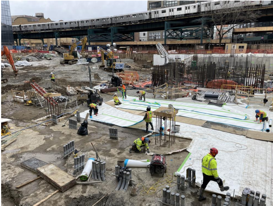
Photo 3: ECD installing waterproofing in the northeastern part of the site (facing west).
