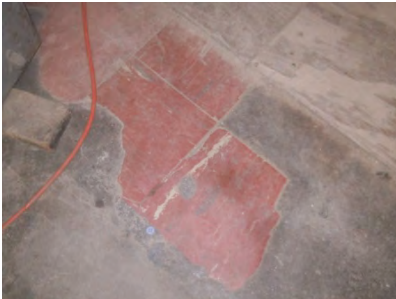
Suspect asbestos-containing floor tiles at the property.
