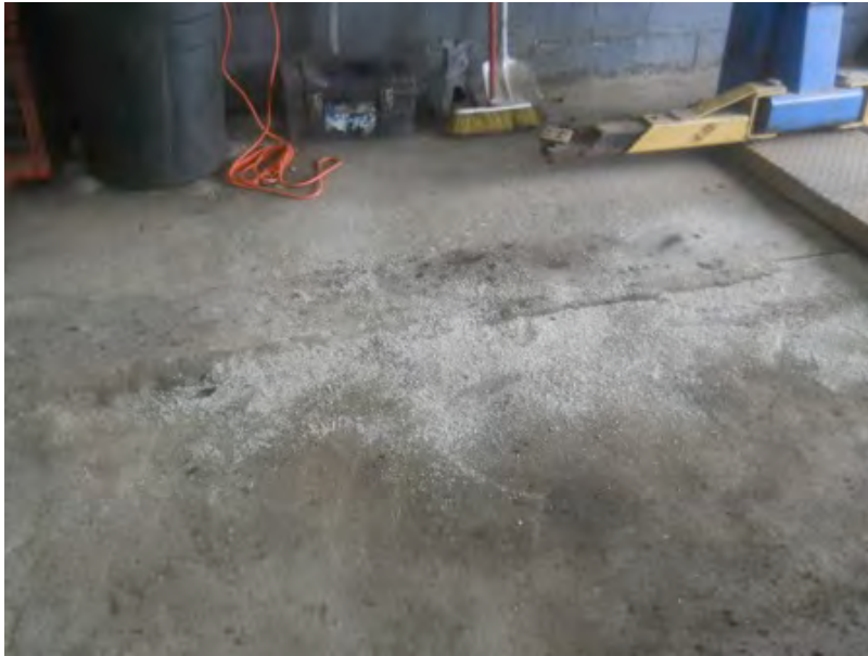
Typical oil stains at the property.
