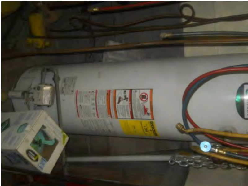
A hot water tank for the building.
