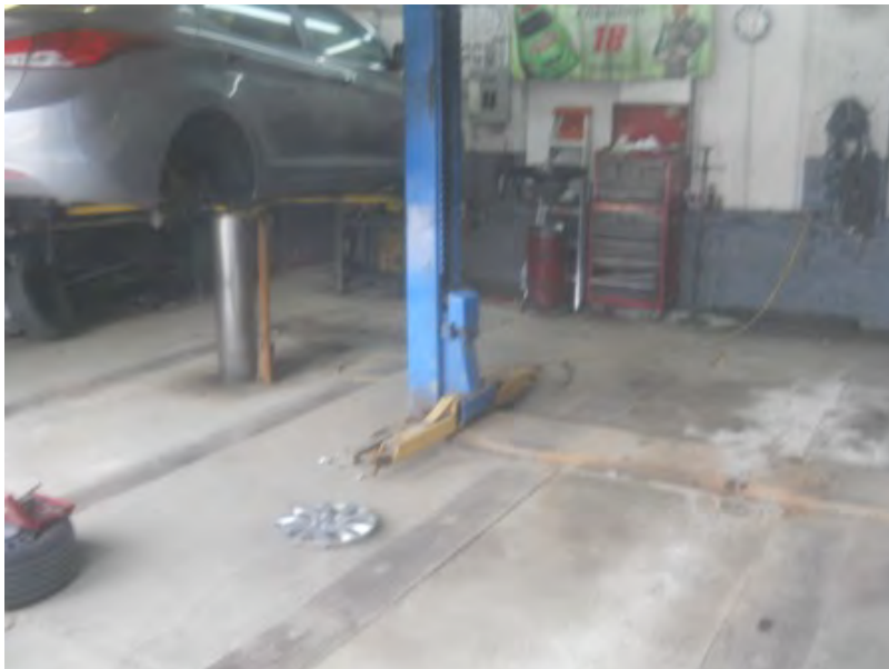
An aboveground lift at the property.
