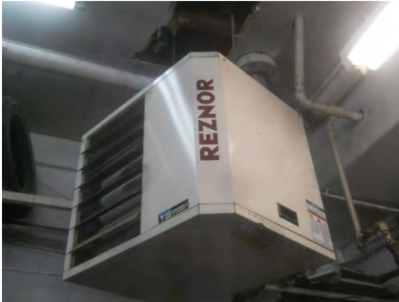
The heating equipment for the building.
