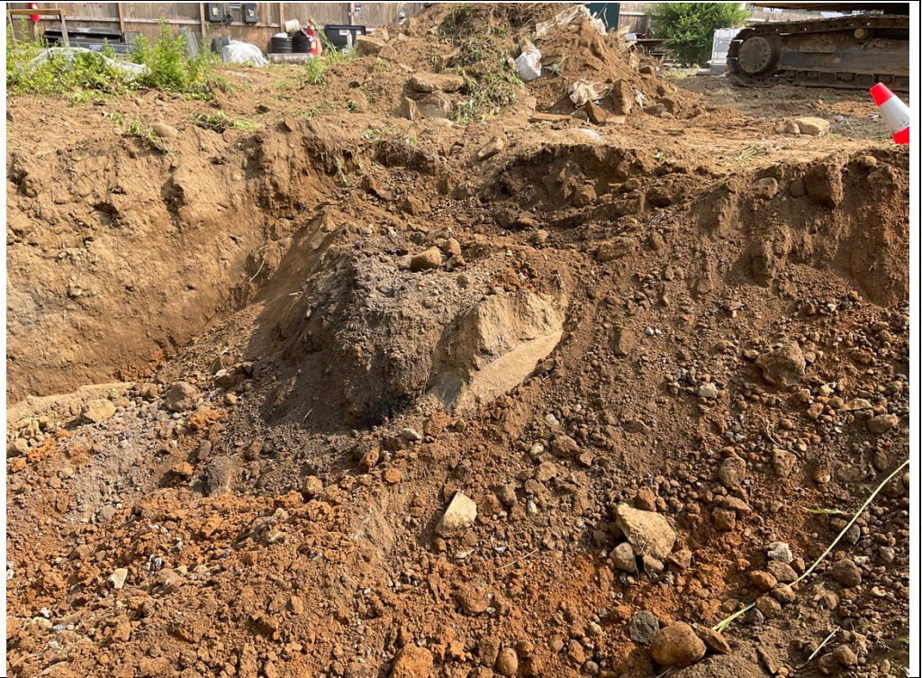
Photo 5 – An UST was found during the excavation at A3 in grid map around 9:35 am.
