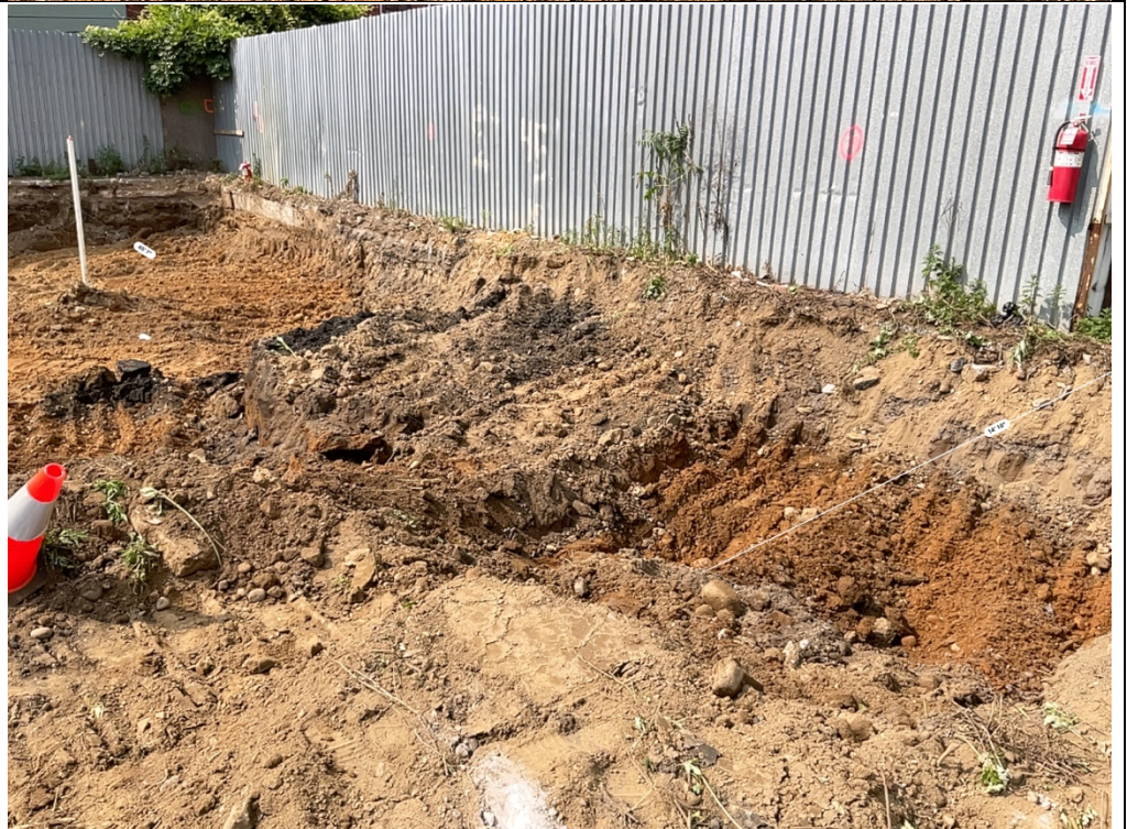
Photo 6 – The UST locates about 14'10" from the western boundary, 65'7" from southern boundary, and about 13" below ground surface.
