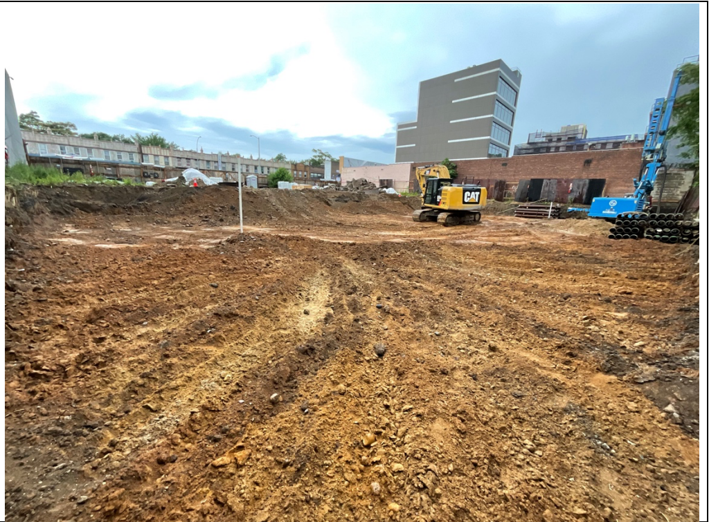
Photo 3 – Excavation area, 2-4 ft bgs, in the SW corner of the site, A3, A4, B3, and B4.
