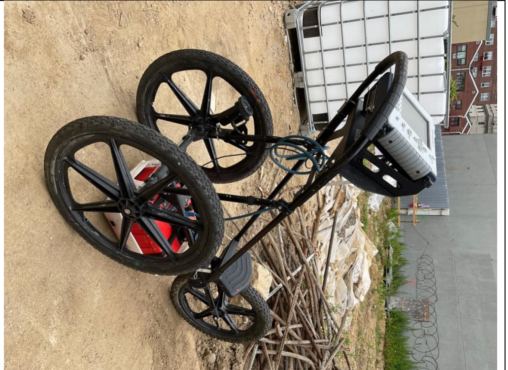
Photo 3- GPR survey was conducted in A1, A2, B1 and B2 to identify historical USTs in the area.
