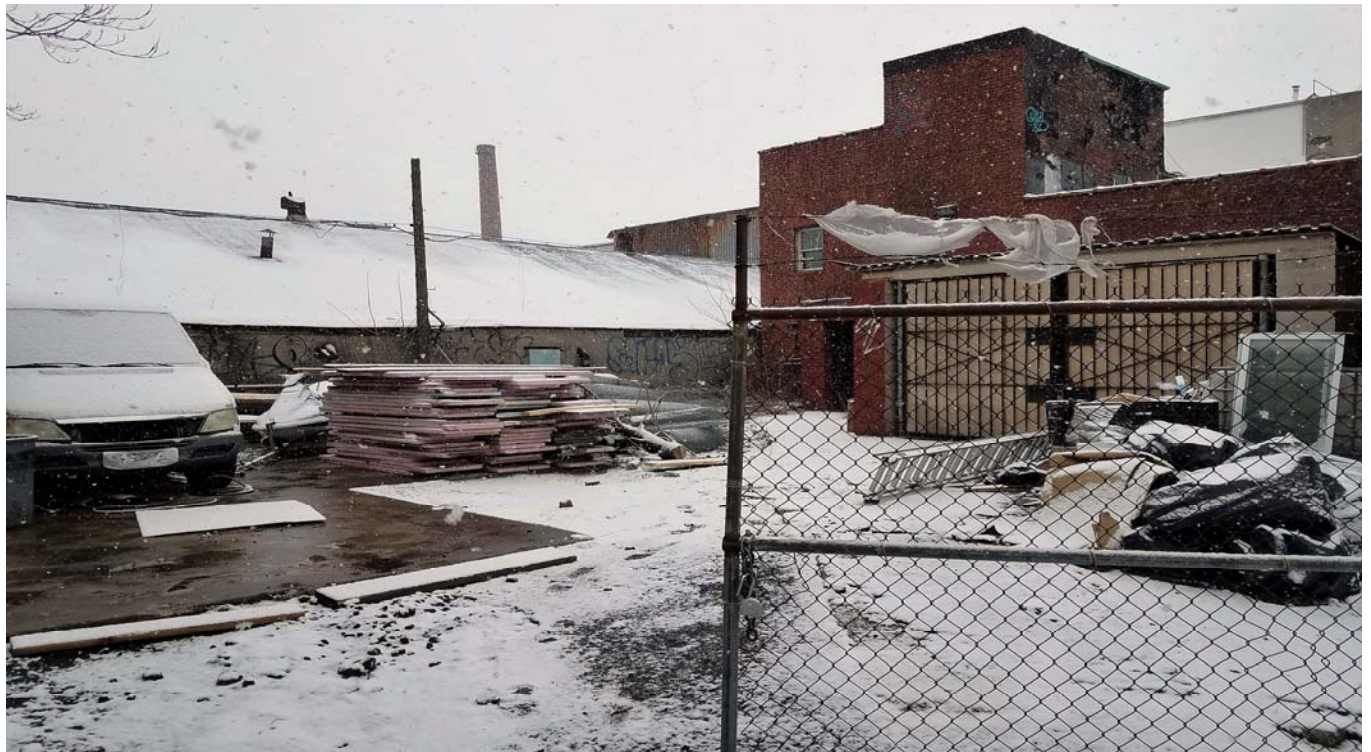
Photo 4 – Yard containing Tank D facing southwest.
