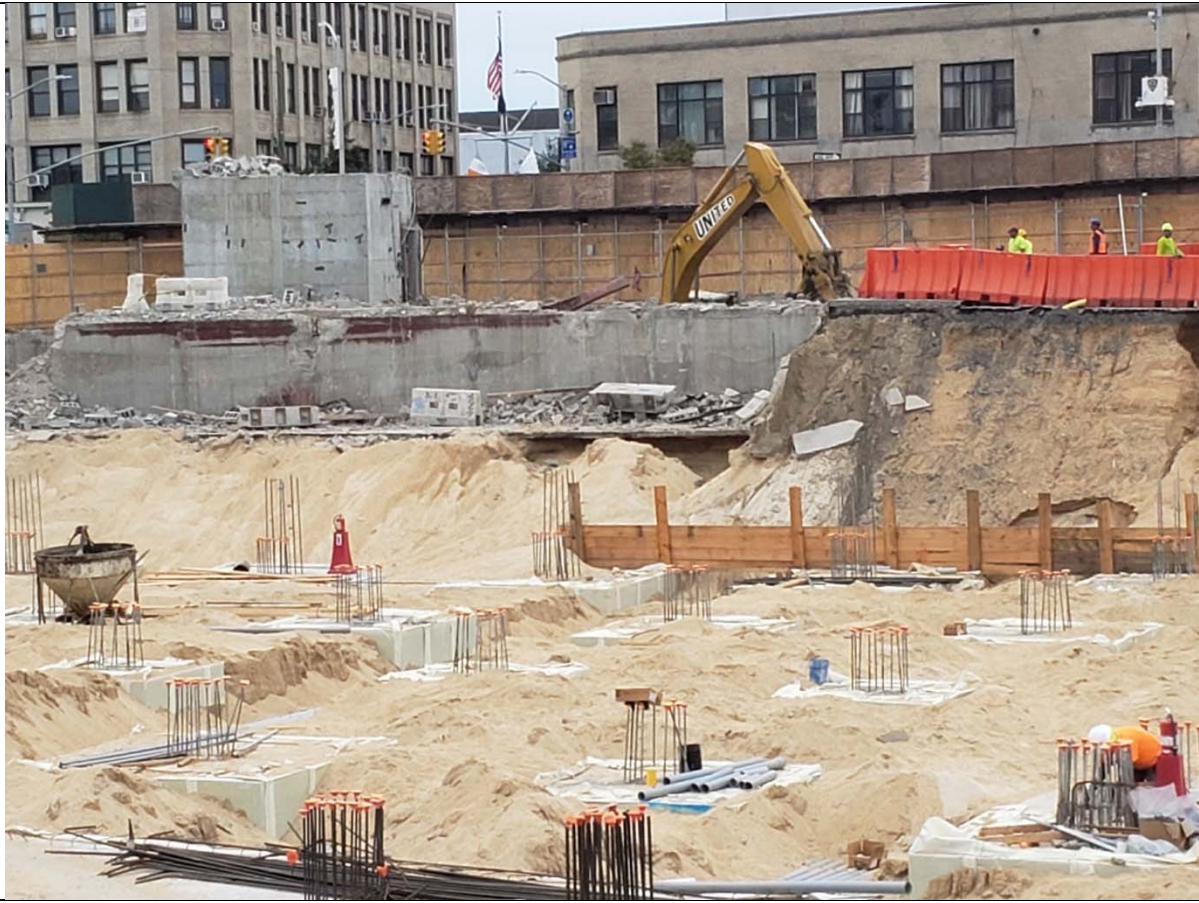
Photo 7 – View of southeast corner of excavation of Building B. Note excavation at former bank.
