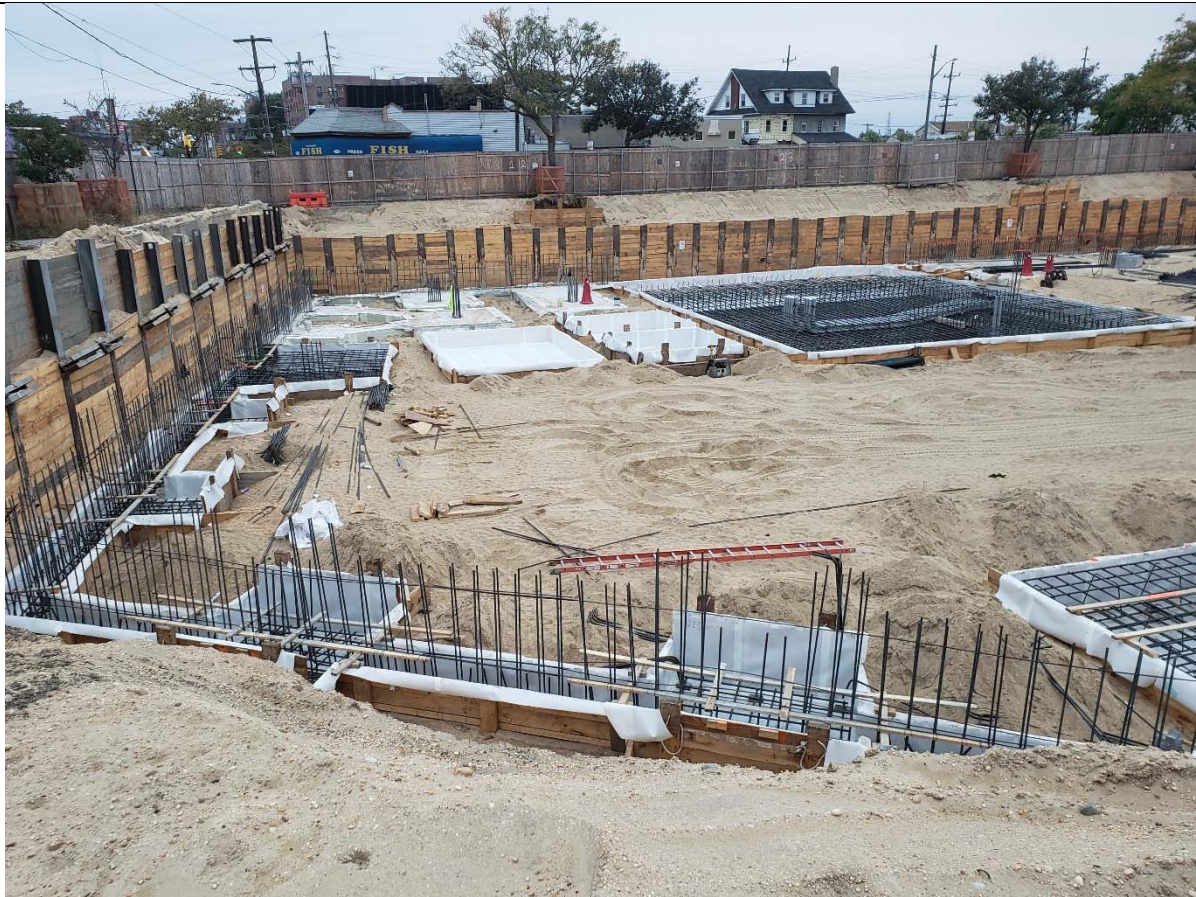
Photo 4 – View of Building C excavation near the southern portion of the building. View is looking west.
