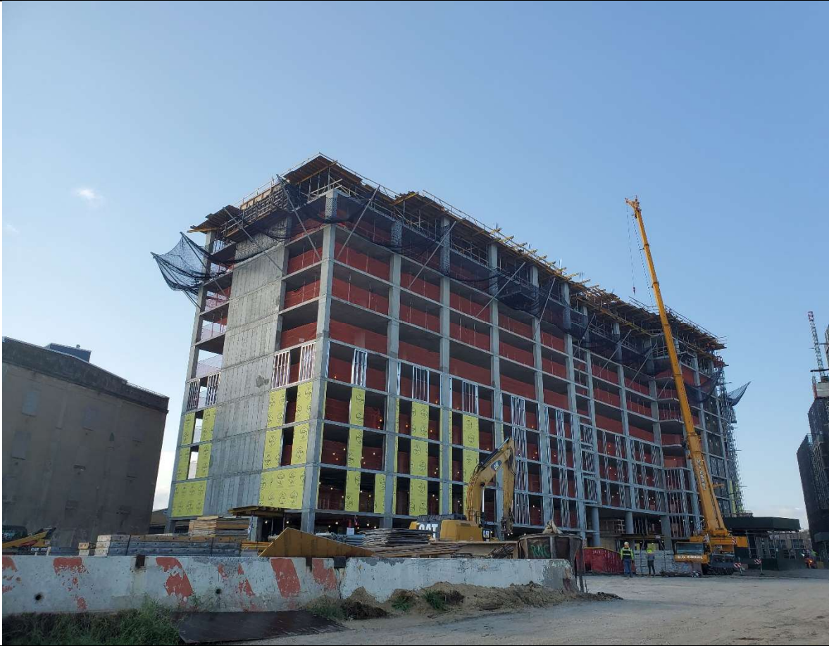
Photo 3- View of rebar, utility, and formwork installation in A3, A4, B3, and B4.
