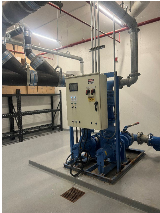
Photo 4: One of the Site's mechanical rooms in cellar.
