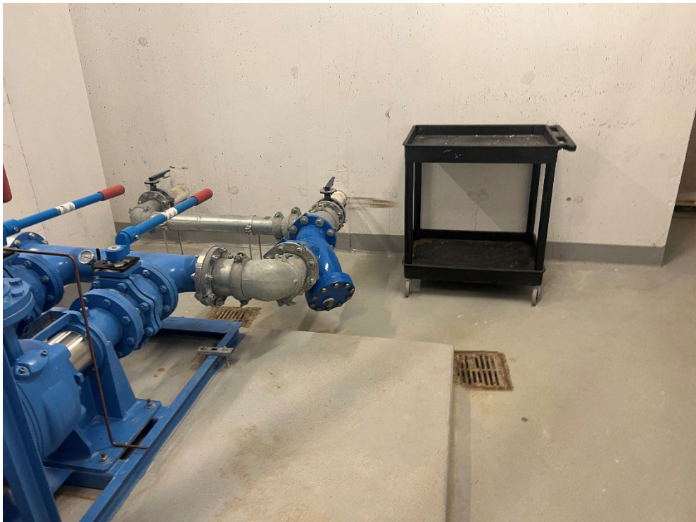
Photo 6: Mechanical room with floor drain in the cellar.
