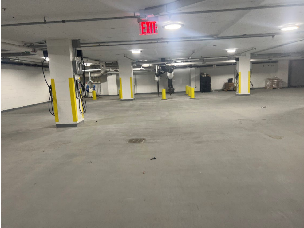
Photo 3: Cellar parking area with electric charging stations.
