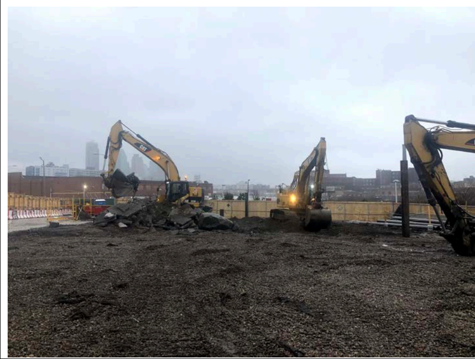
Photo 3: Looking northeast, StructureTech grading soil for leveling purposes and condensing C&D stockpile in WCG-4.
