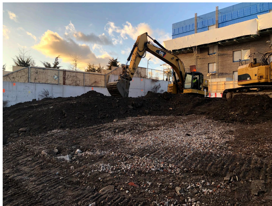
Photo 4: StructureTech continues moving material from the north end of WCG-3 to the south end for leveling.
