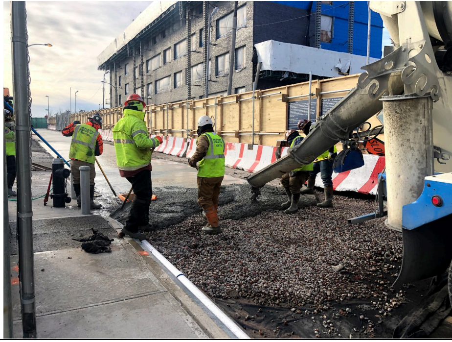
Photo 4: Progress update of filling in former bike lane along 2 nd Street at end of day.
