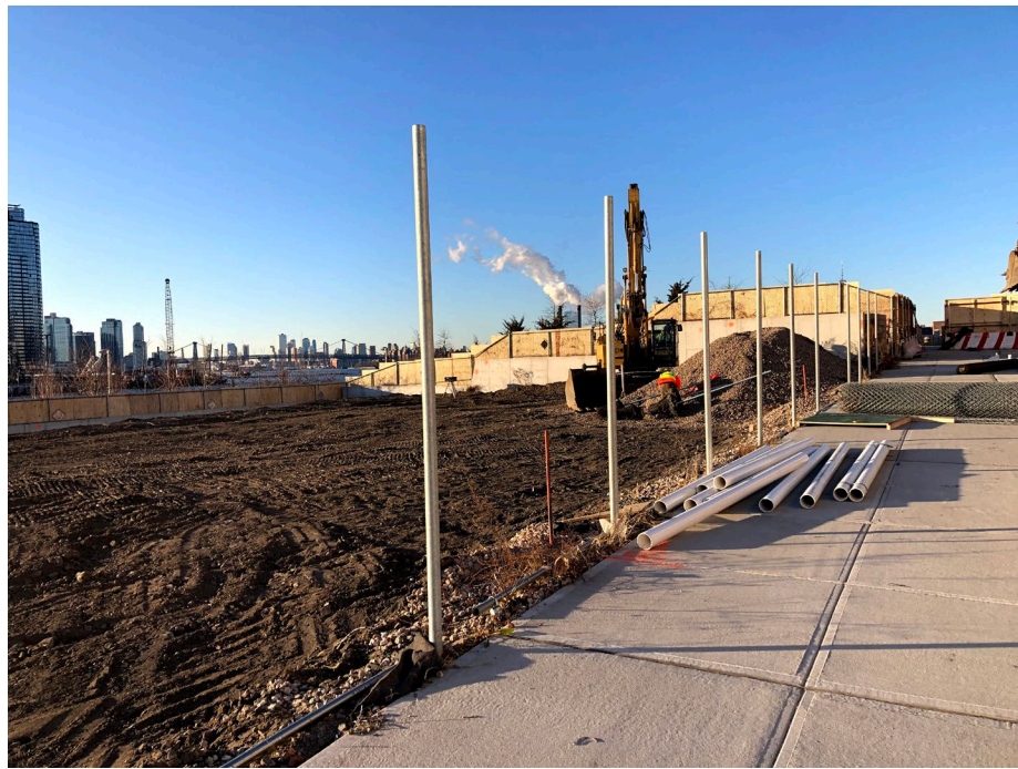
Photo 3: Looking southwest, site status of the southwest portion of the site during fence removal.
