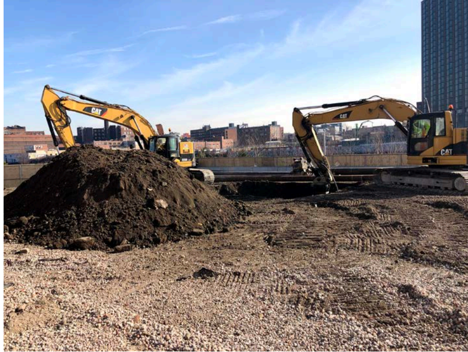
Photo 3: Looking southeast, StructureTech preclearing for pile driving in WCG-1. Material was replaced in excavation.
