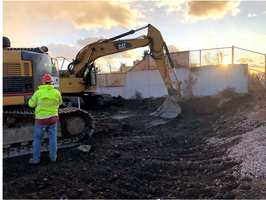
Photo 3: StructureTech begins moving material from the north end of WCG-3 to the south end to level the elevation of the site.
