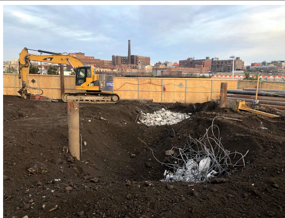
Photo 2: Looking east, site status of the east portion of the site with evidence of footings left in place from historical use at the property.
