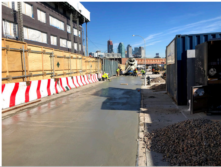
Photo 3: Looking northeast, StructureTech spreading concrete in former bike lane along 2 nd street.
