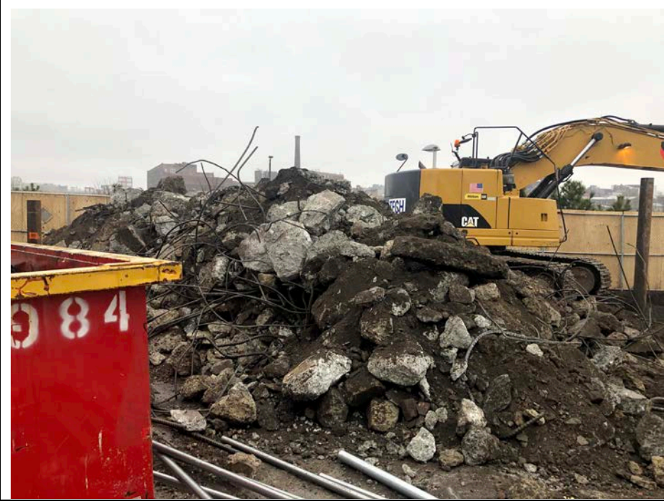
Photo 4: Looking east, site status of east portion of site including C&D stockpile.
