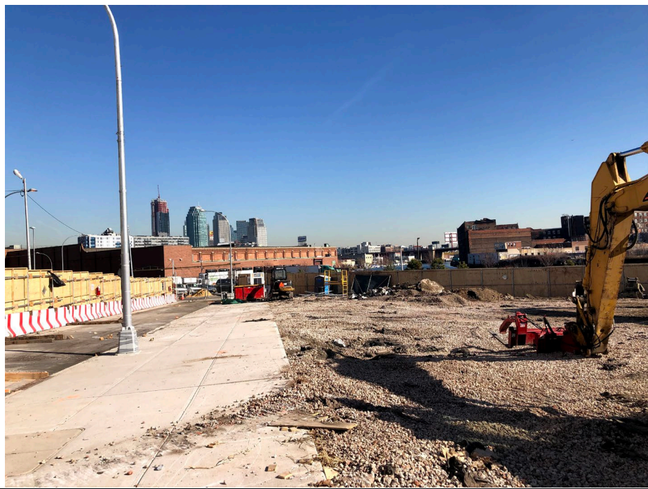
Photo 3: Looking northeast, site status of the northeast portion of site after RCA grading.
