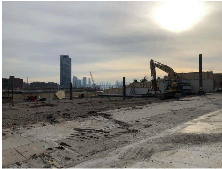
Photo 3: Looking southwest, site status of the southwest portion of site including index piles in WCG-3.
