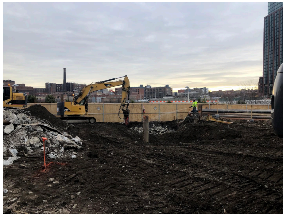
Photo 3: Looking east, site status of the east portion of the site with evidence of footings left in place from historical use at the property. Water being used for dust suppression as concrete is removed.
