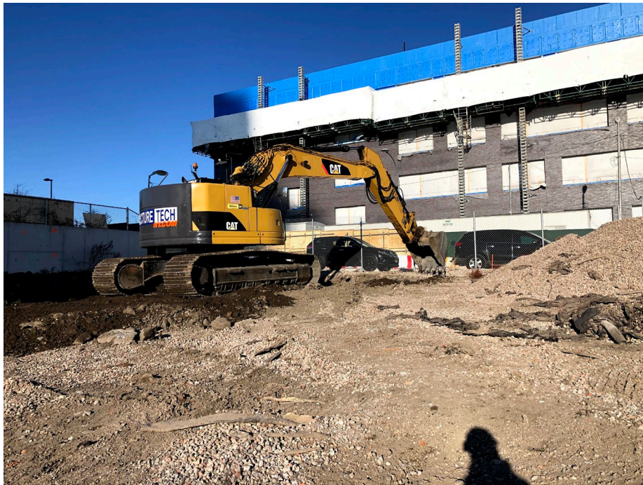
Photo 1: Looking northwest, StructureTech moving material from the north end of WCG-3 to the south end to level the elevation of the site.
