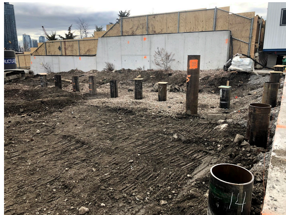
Photo 2: Looking southwest, index pile driving continues in the west side of the site WCG-3.
