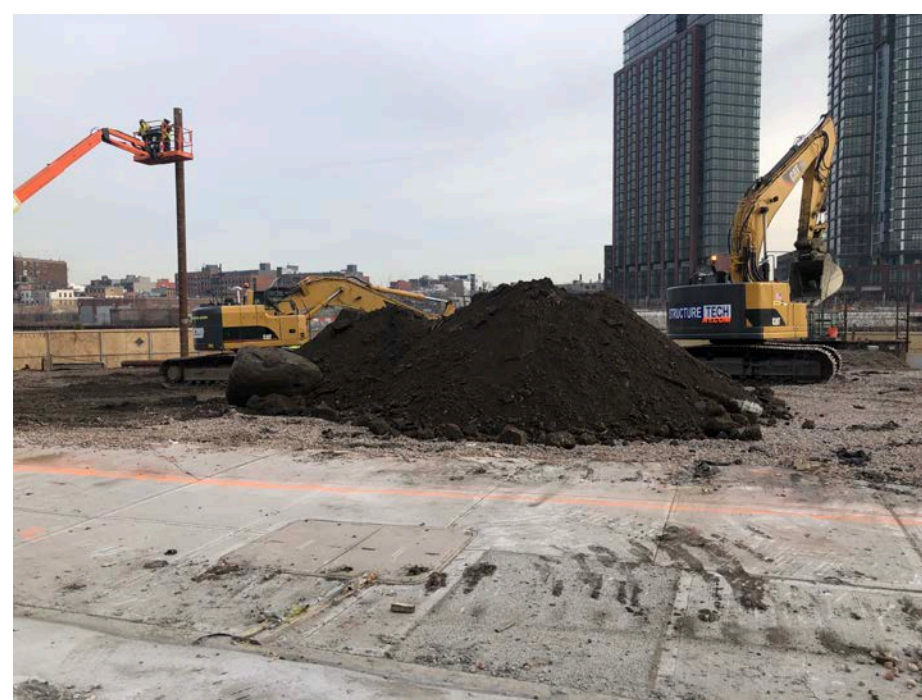
Photo 2: Looking southeast, StructureTech begins excavating in WCG-1 and WCG-2 for preclearing purposes.
