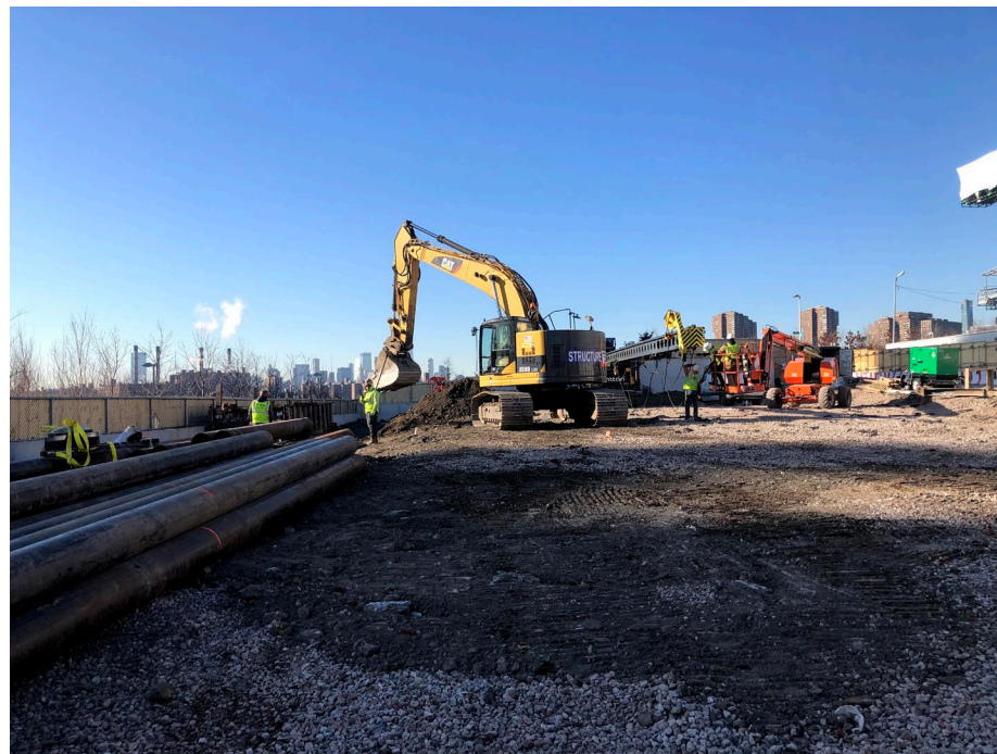
Photo 1: Looking west, site status of the western portion of the site including two excavators, one manlift, and one drill rig.
