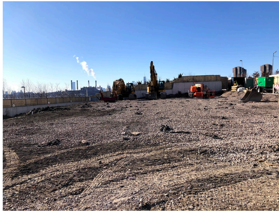
Photo 1: Looking west, site status of the west portion of the site including two excavators and manlift.
