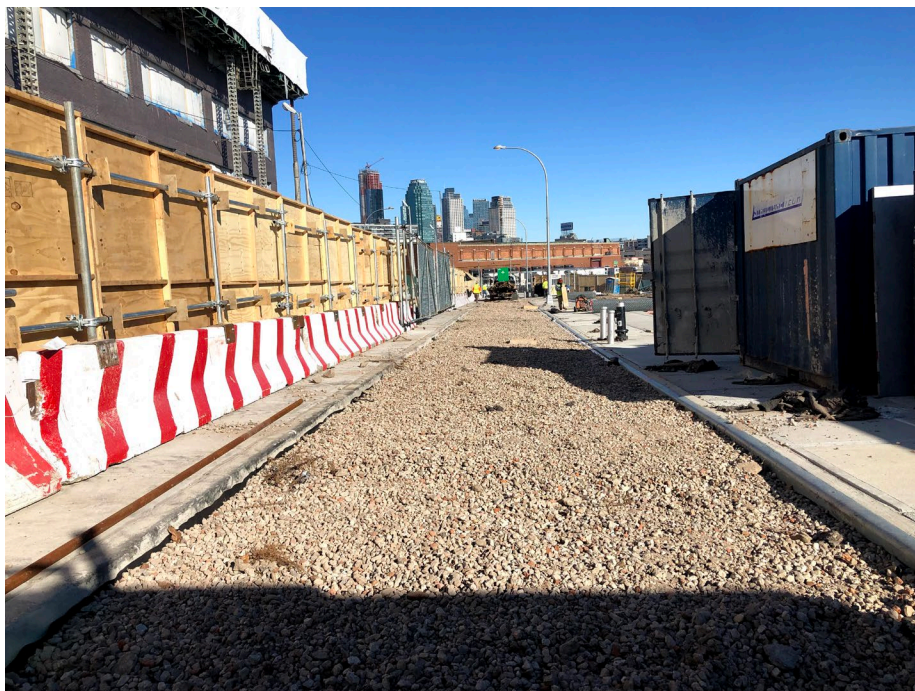
Photo 2: Looking east, site status of 2 nd street after StructureTech placed RCA to level bike path.
