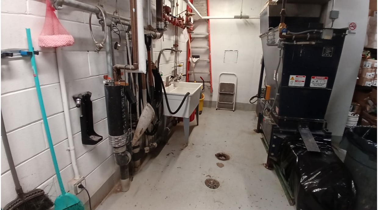
Photograph 8: View within a trash compactor room with floor drains, located in the basement.
