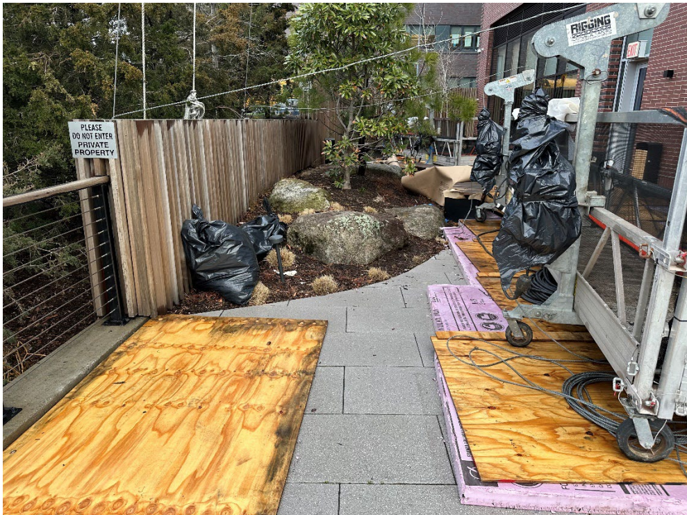
Photo 6: Outdoor patio area with materials for window cleaning.
