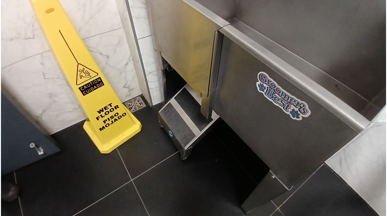
Photograph 10: View of floor drain adjacent to a washing basin station located within the basement pet grooming room.
