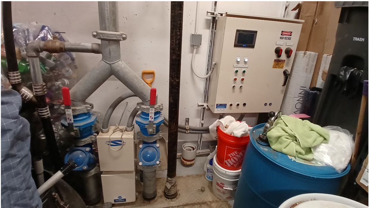
Photograph 7: View within a mechanical room, located in the basement.
