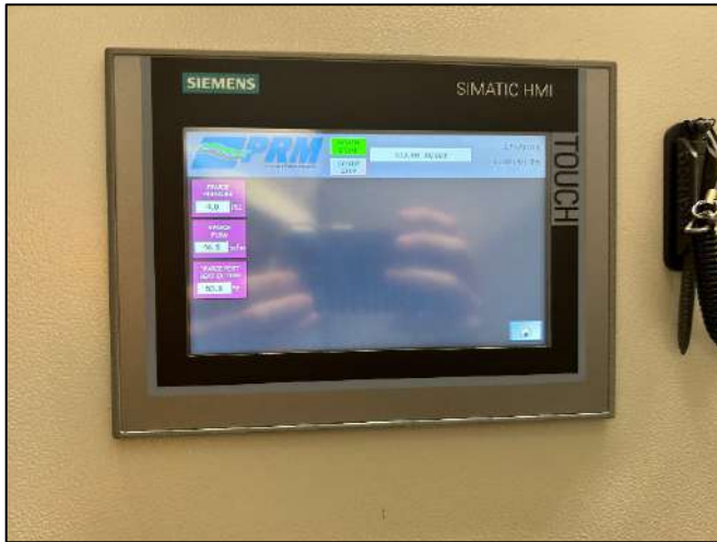
Photograph 1: Biosparge control panel.
