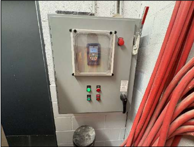
Photograph 9: SSDS control panel.
