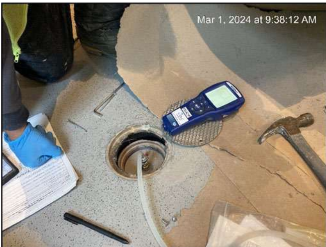
Photograph 11: Collecting SSDS monitoring point readings.
