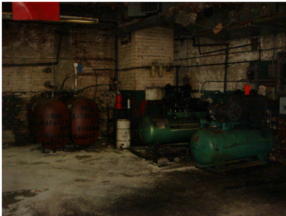
Photo 11: View of two (2) 275 gallon bulk motor oil ASTs and two (2) air compressors located in the two story masonry building to the south of the repair shop
