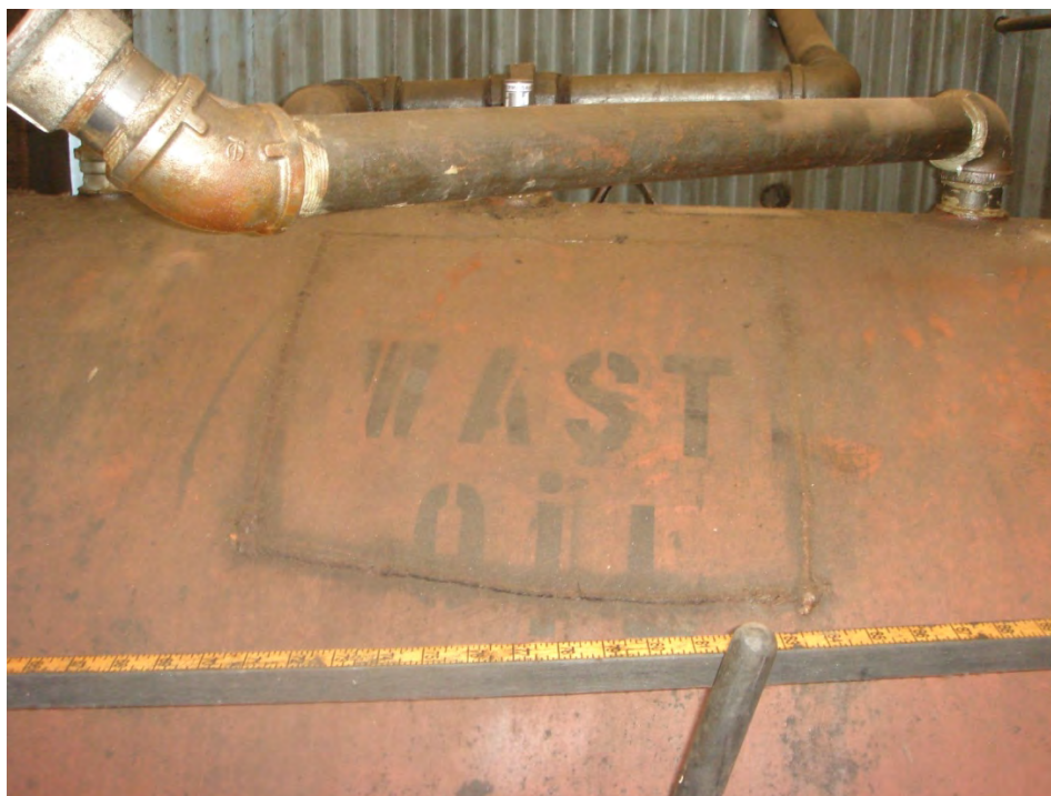
Photo 12: View of the exterior waste oil AST with a capacity of 450 gallons located adjacent to the repair shop
