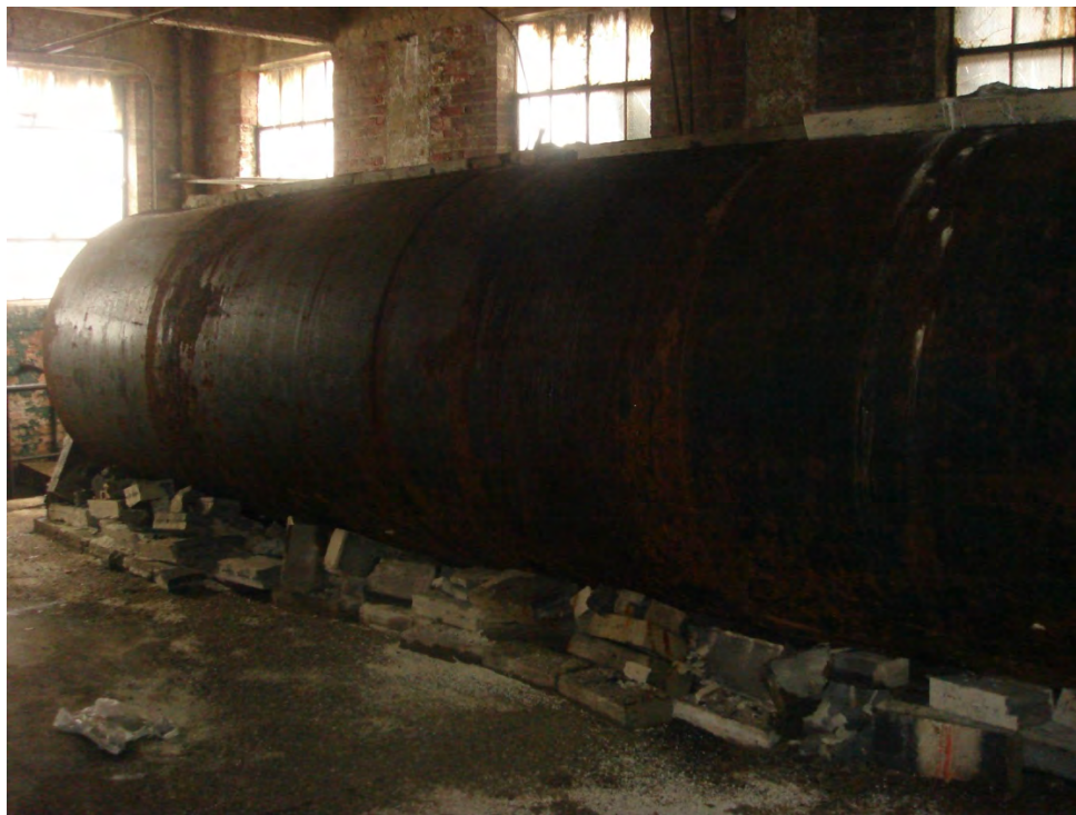
Photo 12: View of the former 5,000 gallon heating oil tank that was decommissioned after Hurricane Sandy
