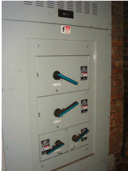
Photo 11: View of the interior electric control switches located in the two story masonry building adjacent to the northeastern corner of the Site
