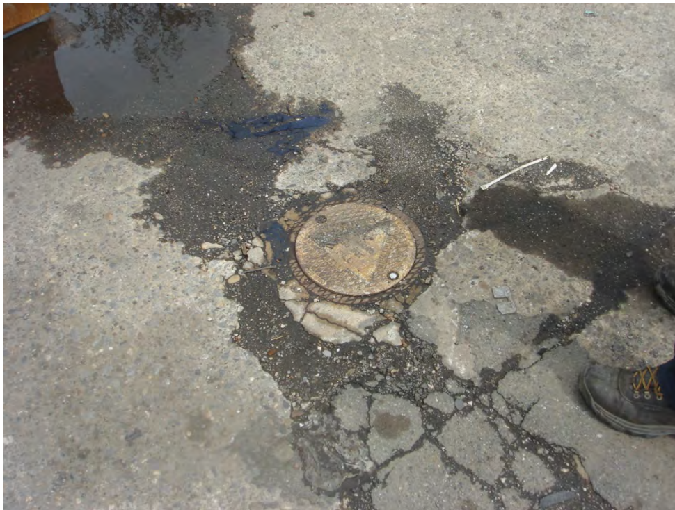
Photo 7: View of one of the multiple decommissioned monitoring wells found on the Site
