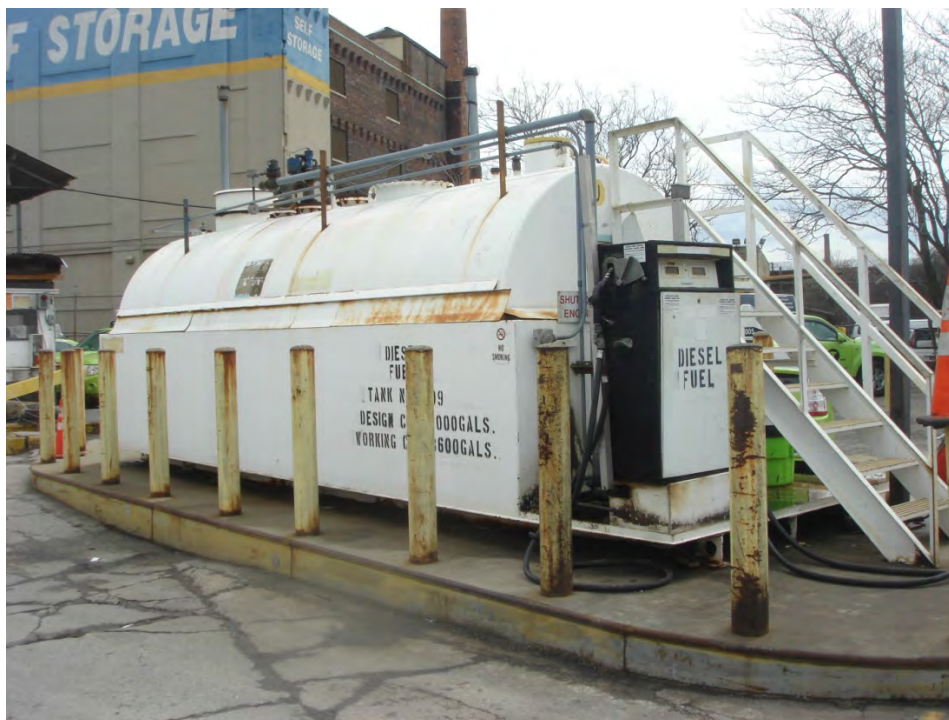
Photo 6: View of the 4,000 gallon diesel fuel above ground storage tank located adjacent to the former fueling racks
