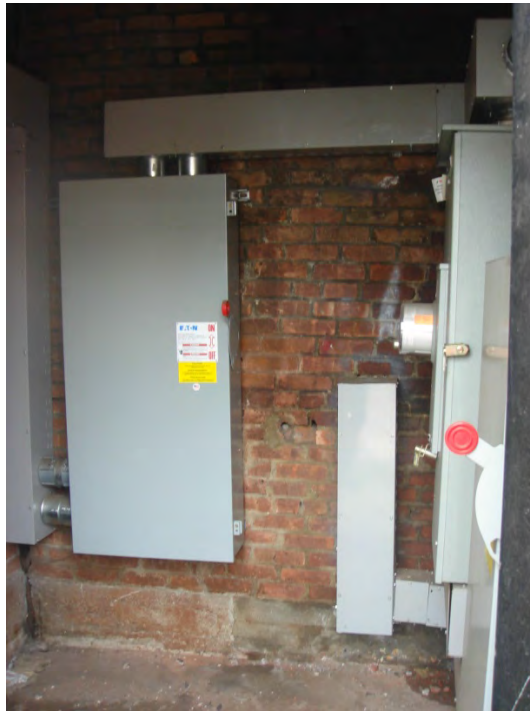
Photo 11: View of the interior electric control boxes located in the two story masonry building adjacent to the
