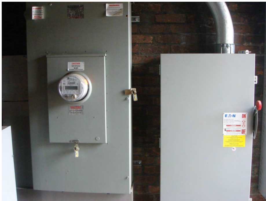
Photo 12: View of the interior electric control box and meter located in the two story masonry building adjacent to the northeastern corner of the Site
