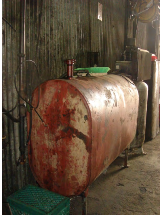
Photo 11: View of a 500 gallon AST located within the repair shop
