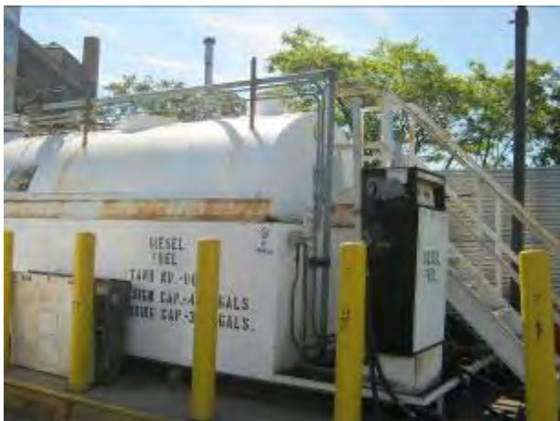
23. View of diesel AST is the northeast portion of the subject property
