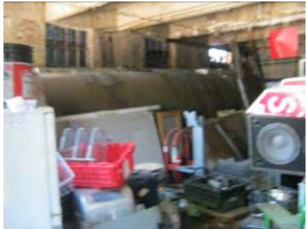
14. View of the out of use 5,000-gallon heating oil AST in Building C
