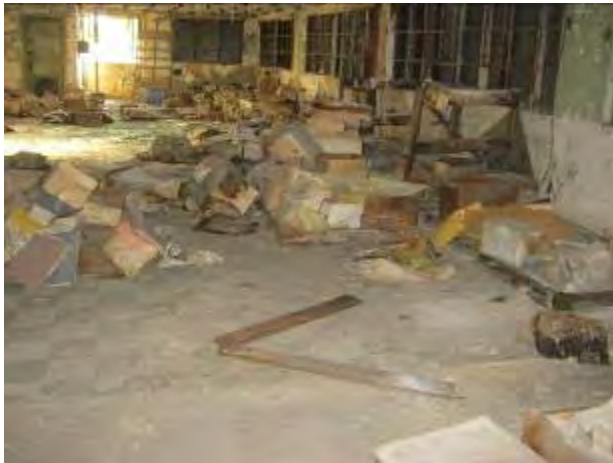
13. View of damaged ACMs on the second floor of Building B
