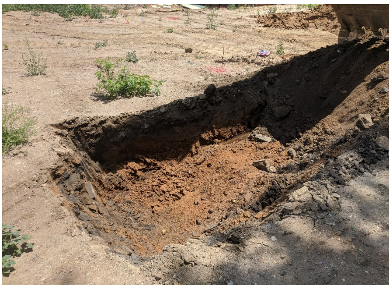
Photo 12, View of construction debris (e.g. bricks) being excavated from TP-3.
