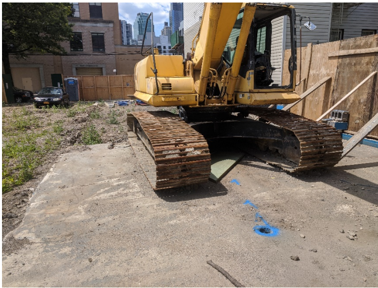
Photo 1, View of a water pipe located along the northern edge of the Site.
