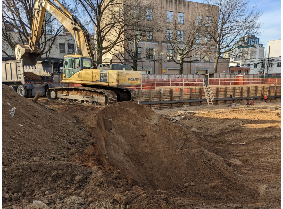
Photo 1 – View of excavator loading hazardous waste from SB-102 hotspot in Quadrant 3, facing south
