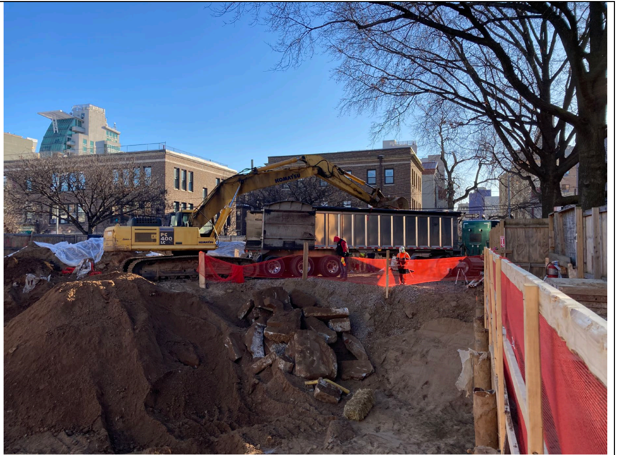
Photo 3 – View of the excavator loading clean soil from Quadrants 1 and 6 into truck for export, facing east.
