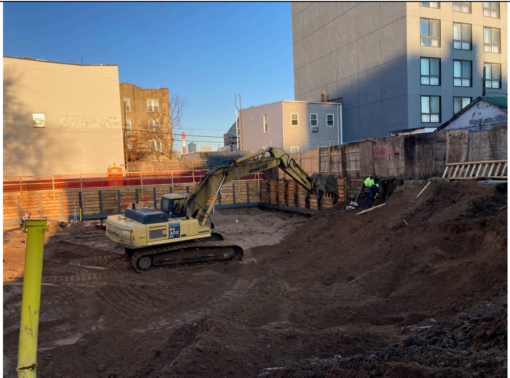
Photo 2 – View of the workers completing shoring work along the northern site boundary (Quadrant 2)
