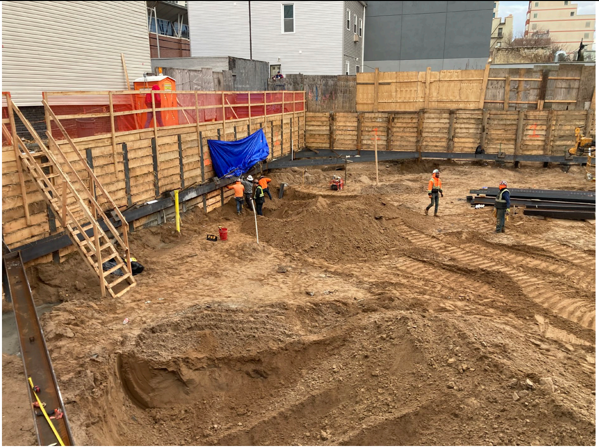
Photo 3 – View of soil scraped to allow further lagging work to be performed in Quadrant 1.
