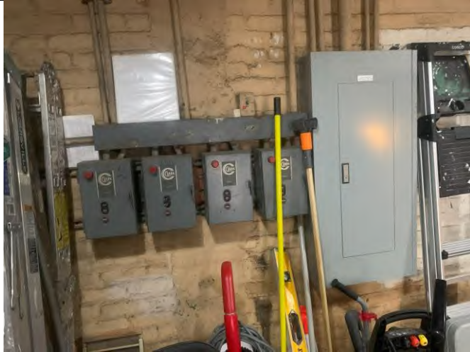
Electric panel in maintenance room
