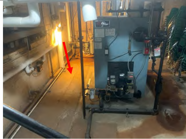
Proposed VMP in maintenance room next to sump in northeastern corner of maintenance room
