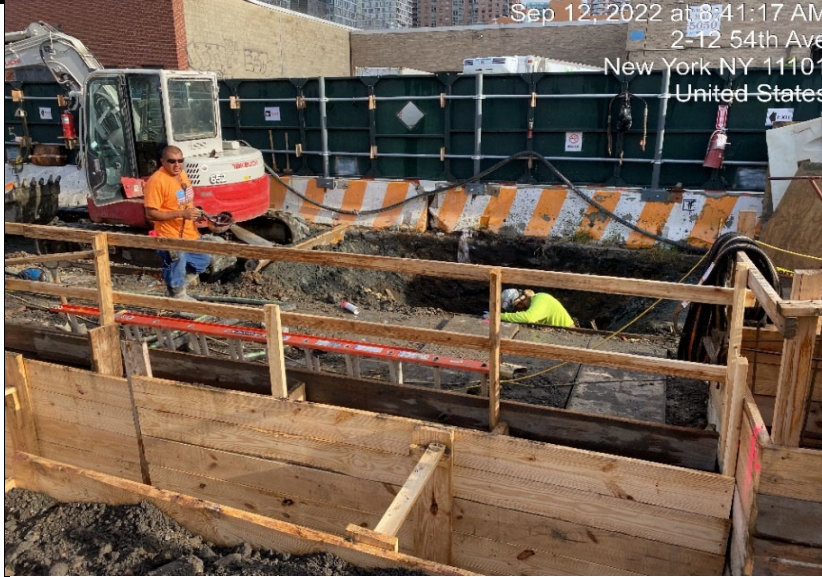
Photograph 1 - Excavation of soil in Grid WC-05 for foundation elements, view facing north.
