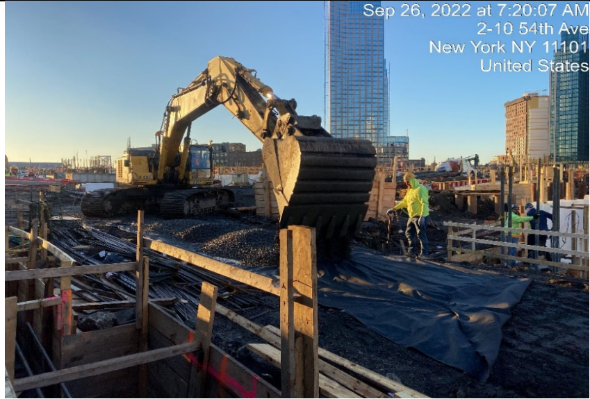
Photograph 1 - Installation of 3/4" stone on top of geotextile in Grid WC-02, view facing southeast.
