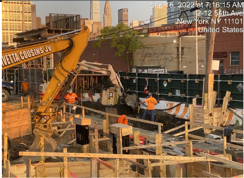
Photograph 1 - Excavation of soil in Grid WC-05 for foundation elements, view facing northwest.
