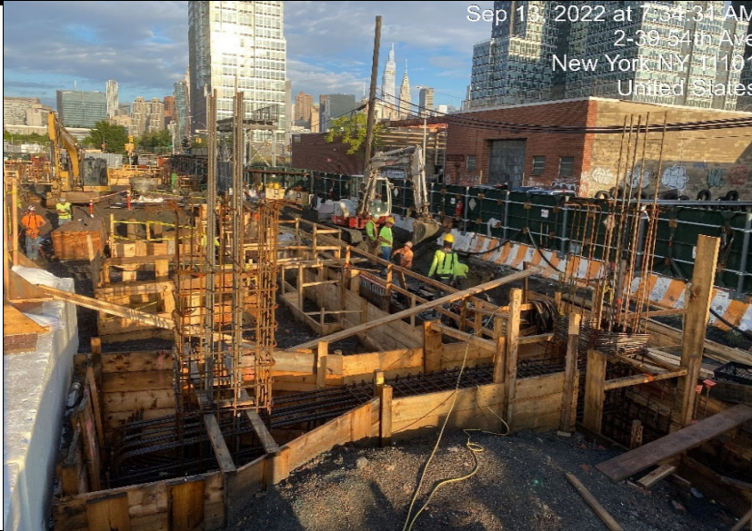
Photograph 1 - Excavation of soil in Grid WC-05 for foundation elements, view facing northwest.
