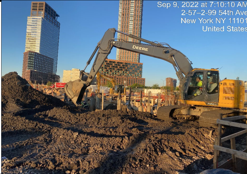
Photograph 1 - Excavation of soil in Grid WC-02 for foundation elements, view facing southwest.
