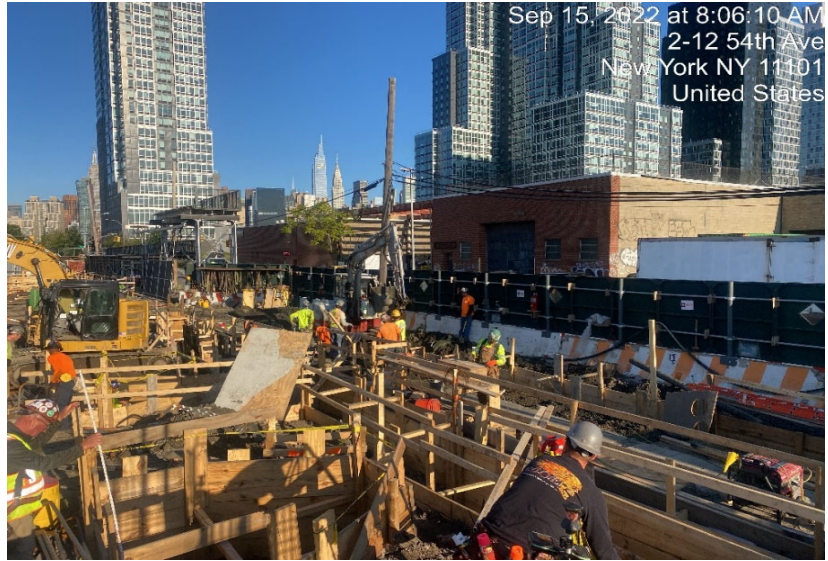
Photograph 1 - Excavation of soil in Grid WC-05 for foundation elements, view facing northwest.
