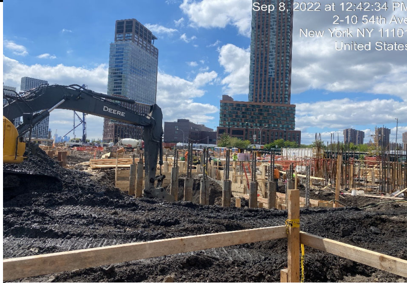
Photograph 1 - Excavation of soil in Grid WC-02 for foundation elements, view facing southwest.
