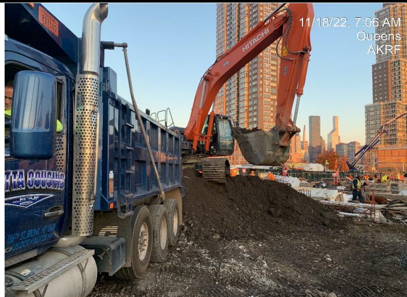
Photograph 2 - The landscaping contractor preparing to export soil from WC-17, view facing northwest.
